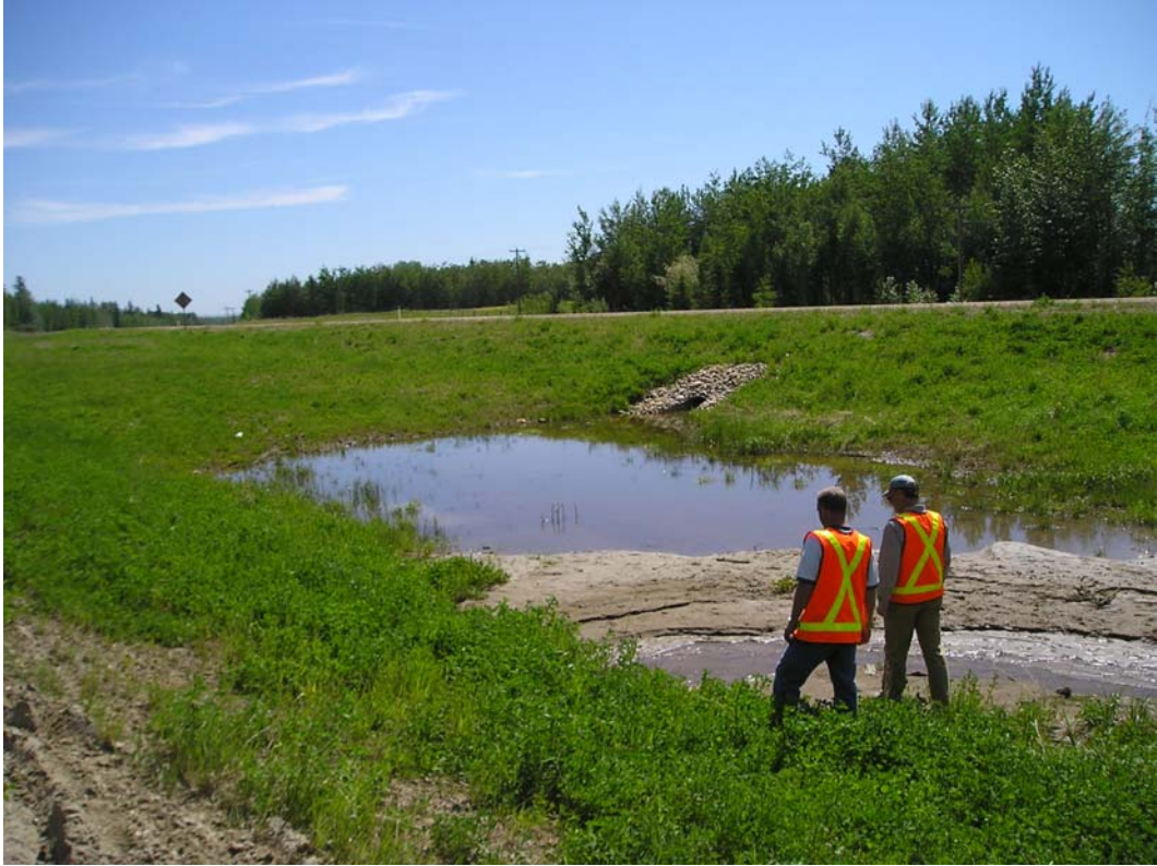
Photo 5 – Sand/Silt bar and ponded water in twin culvert inlet area. May 31, 2005
