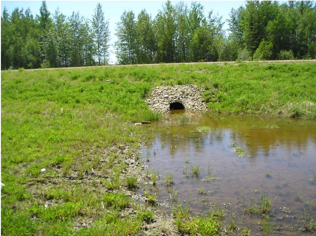
Photo 6 – Ponded water in centreline culvert outlet area. May 31, 2005
