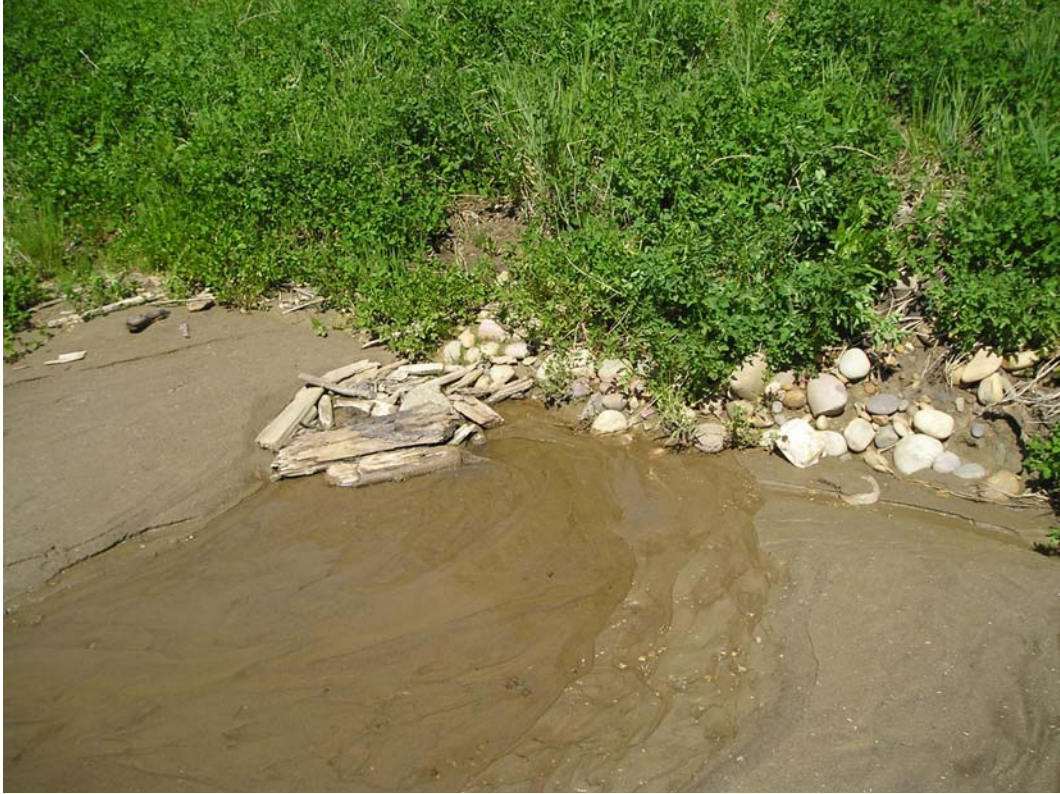
Photo 3 – Inlet of twin culverts (water seeping in through overlying silt and sand).
