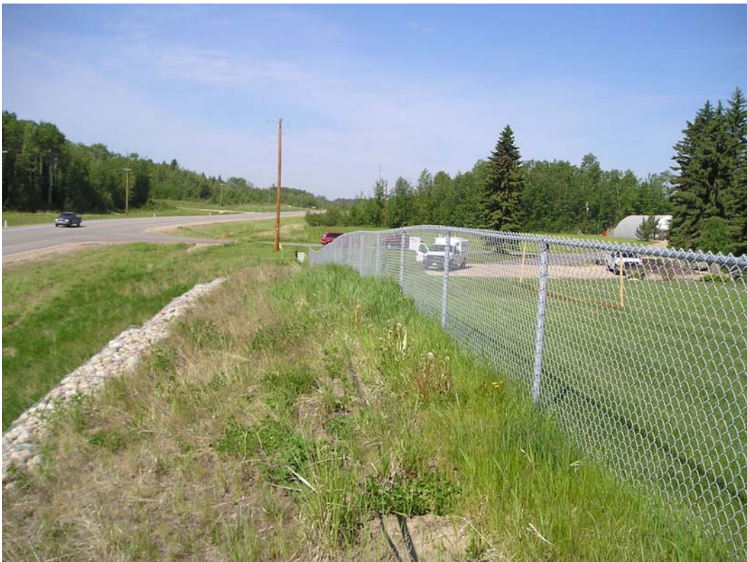
Photo 4 – Sag in Fence between Sinkhole #1 and depression in lawn. (Looking west).
