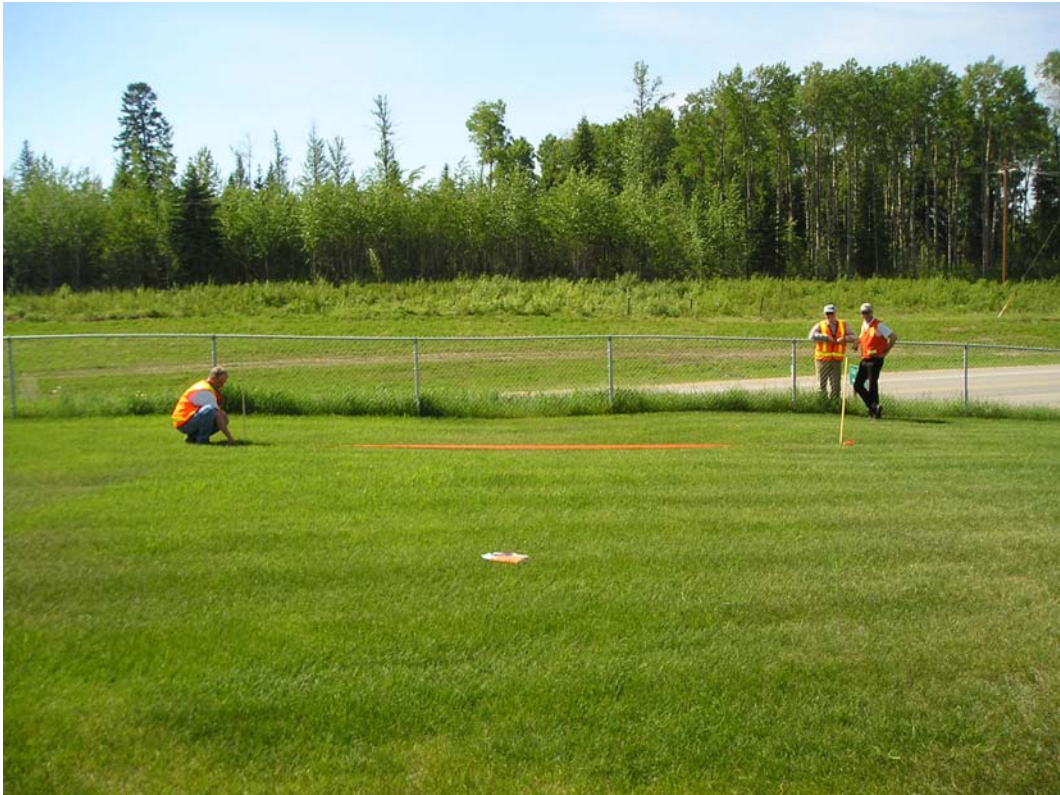
Photo 5 – Depression in lawn area and sag in fence. May 31, 2005
