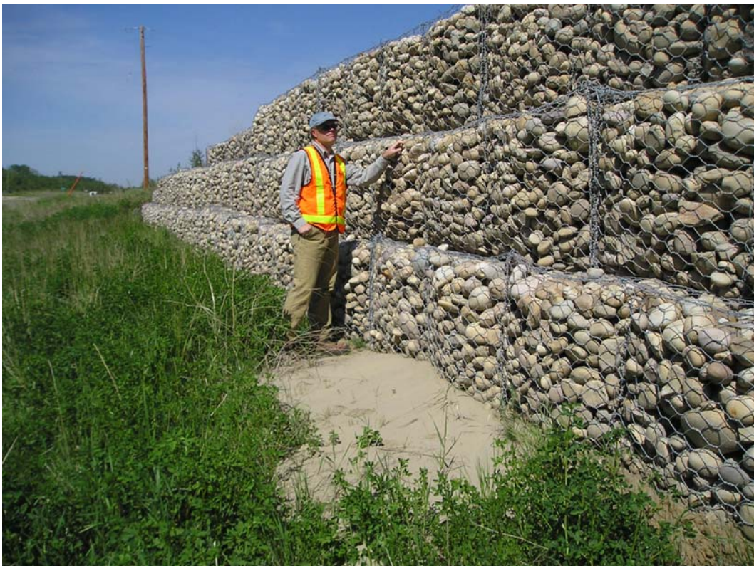
Photo 8 – Fine sand deposit at toe of wall adjacent to Sinkhole #1. May 31, 2005
