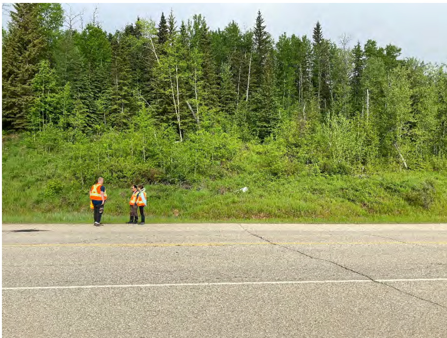
Photo 4: Slope failure. Looking west.
