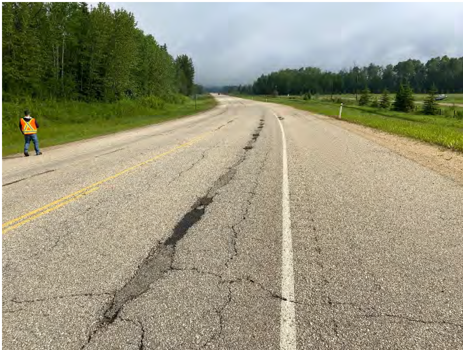
Photo 2: Pavement cracks along Highway 32, north of slope failure. Looking north.
