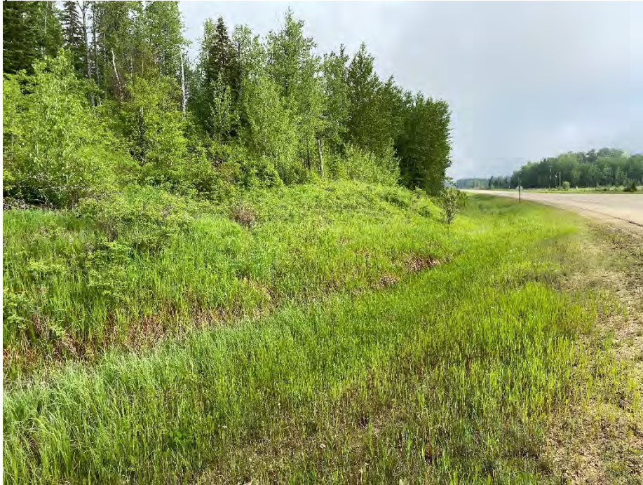
Photo 5: South side of slope failure. Looking north.
