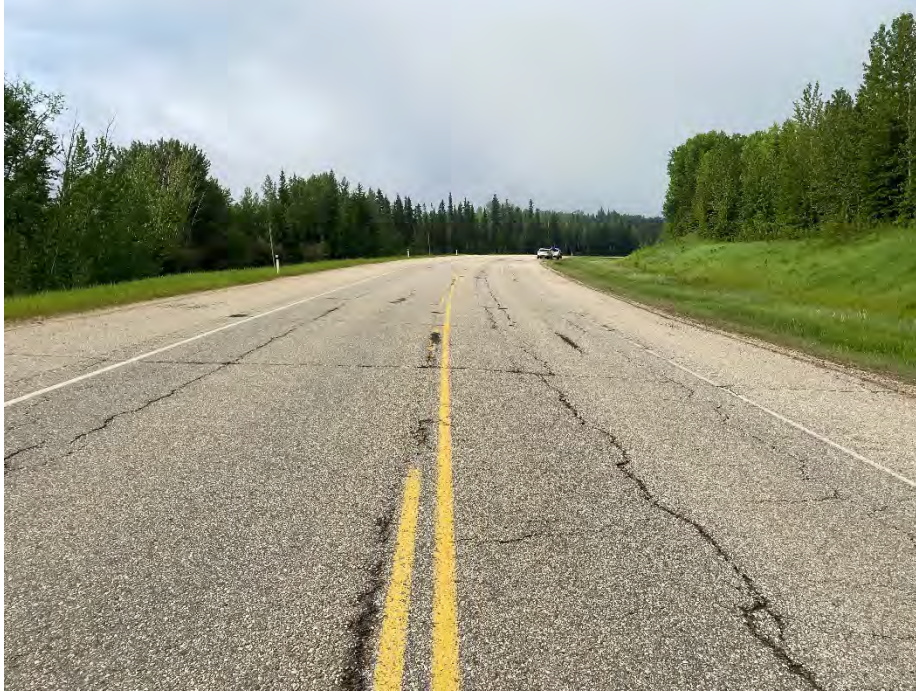
Photo 1: Pavement cracks along Highway 32, near slope failure. Looking south.
