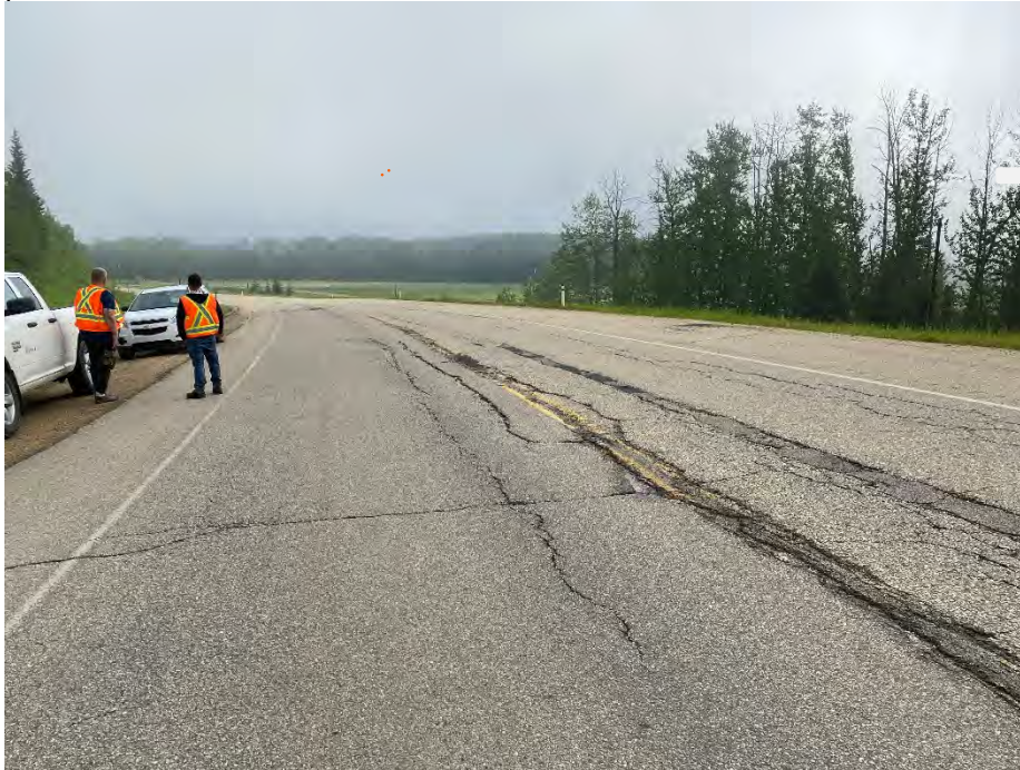
Photo 3: Pavement cracks along Highway 32, north of slope failure. Looking northeast.
