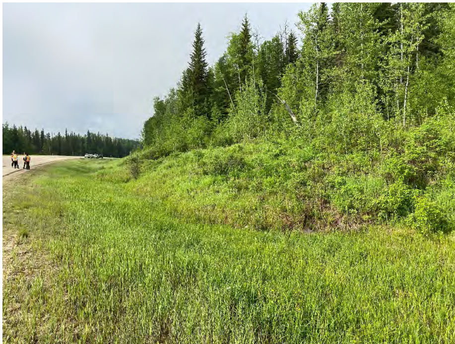
Photo 6: North side of slope failure. Looking southwest.
