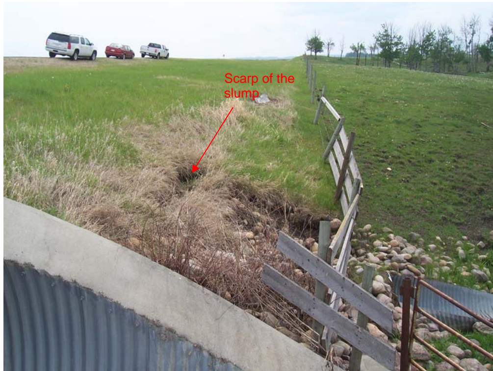
Culvert inlet slump.
