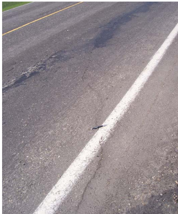
Faint pavement crack with no differential drop.
