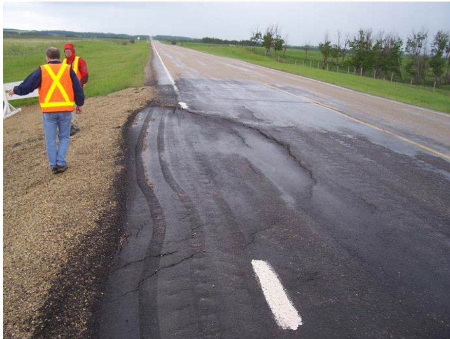
Photo 1 - View of the distressed area.
