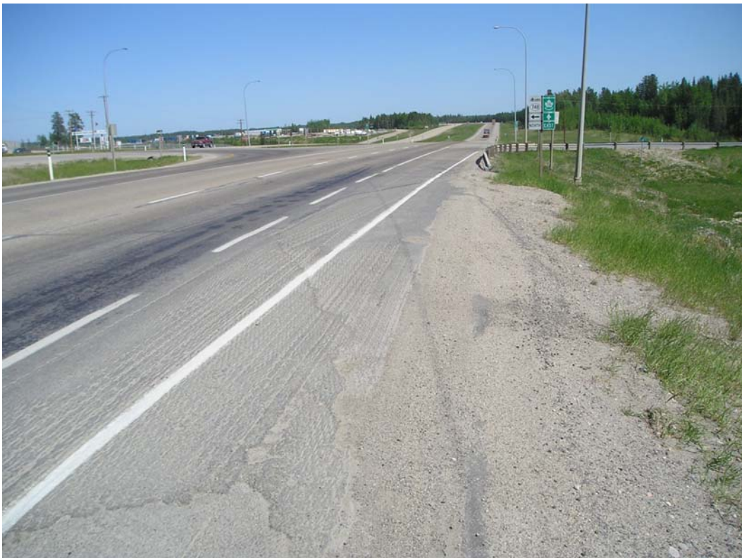
Photo 2 – Looking east at main crack location.
