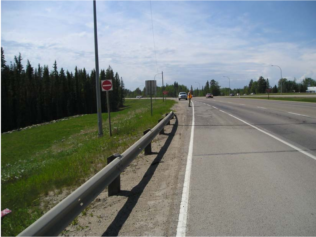
Photo 1 - Looking west at pavement distress area.
