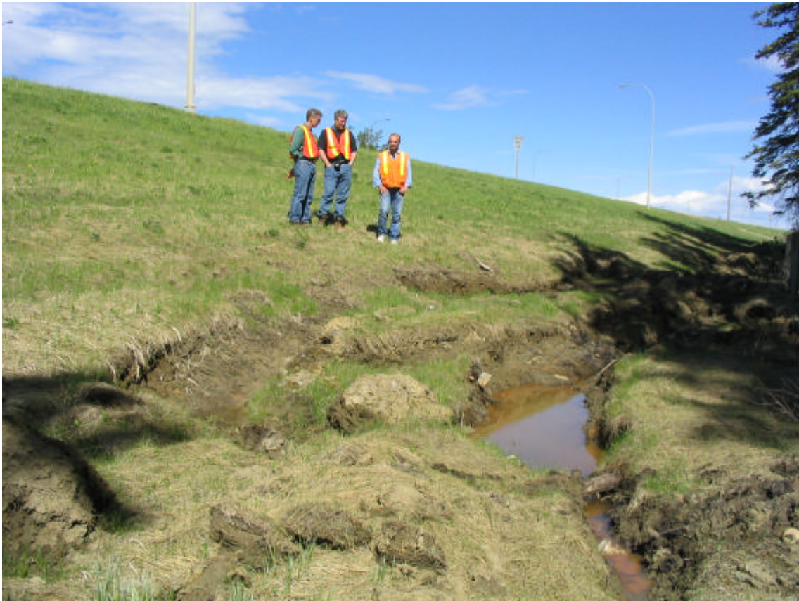
PHOTO 8 PONDED WATER IN RUTS
