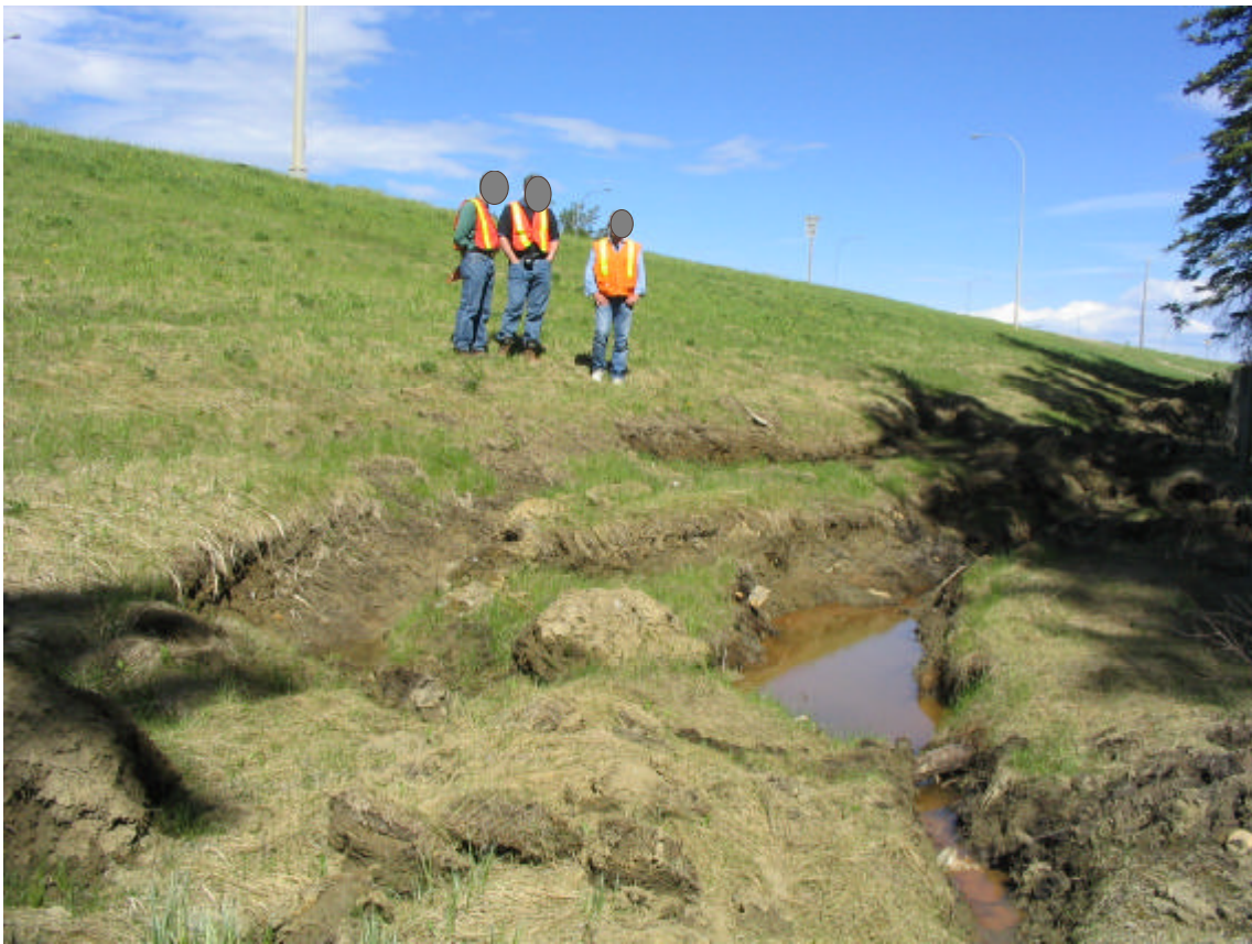
PHOTO 8 PONDED WATER IN RUTS
