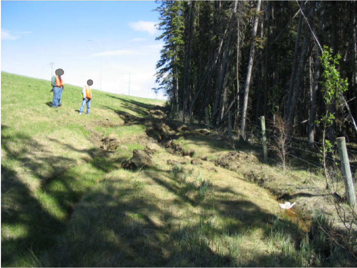
PHOTO 7 RUTTED ZONE WEST OF SLIDE AREA (LOOKING EAST)
