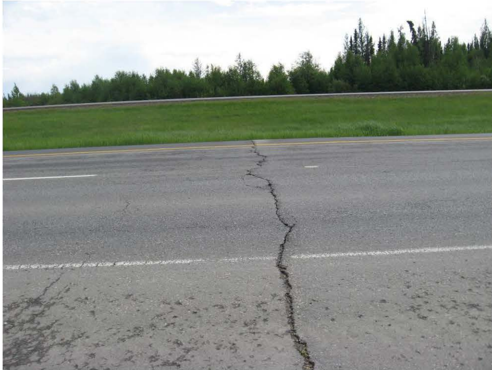
Photo 3 – Looking south at west crack, June 11, 2008.
