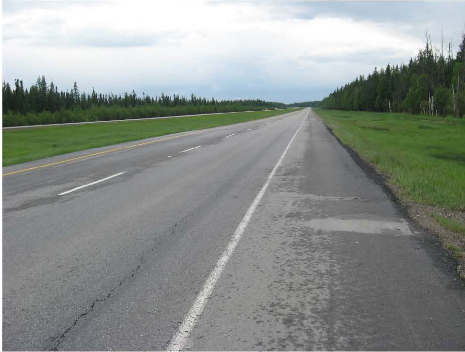
Photo 1 – Looking west toward distressed section, June 11, 2008.
