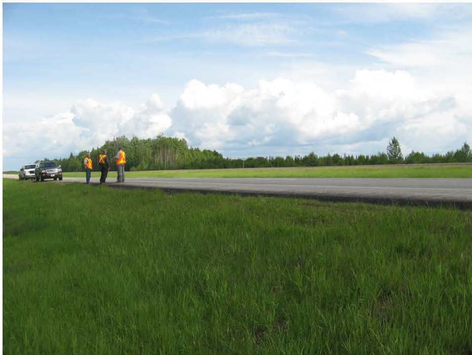
Photo 4 – Looking southeast at distressed section. Note lack of obvious displacement compared to surrounding pavement, June 11, 2008.
