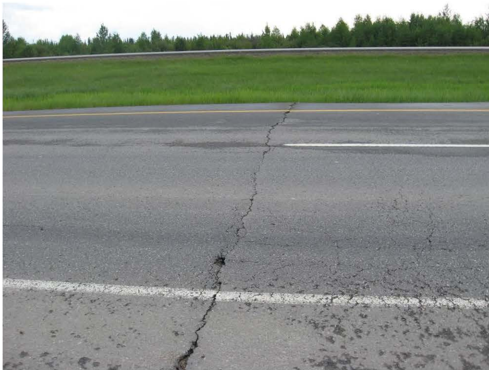
Photo 2 – Looking south at east crack, June 11, 2008.
