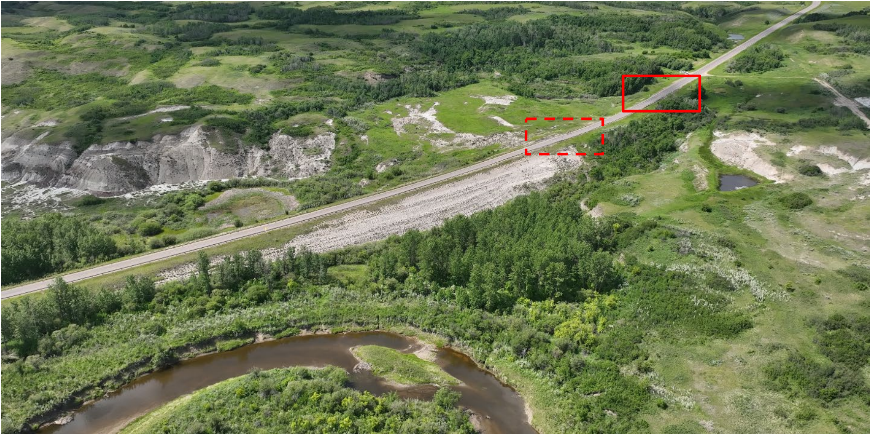
Photo 1 Oblique aerial photo of the C003 site (approximate area of pavement patching indicated by red rectangle and area of pavement patching with recent cracking, settlement, and guardrail buckling indicated by rectangle with red dashed line). Photo taken June 17, 2024, facing northwest.
