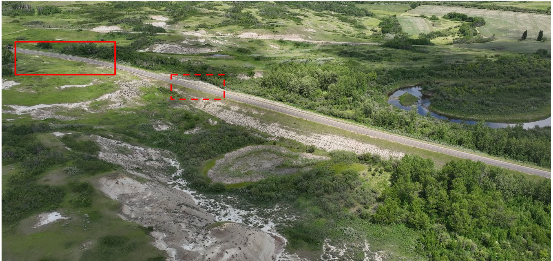
Photo 2 Oblique aerial photo of the C003 site (approximate area of pavement patching indicated by red rectangle and area of pavement patching with recent cracking, settlement, and guardrail buckling indicated by rectangle with red dashed line). Photo taken June 17, 2024 facing east.
