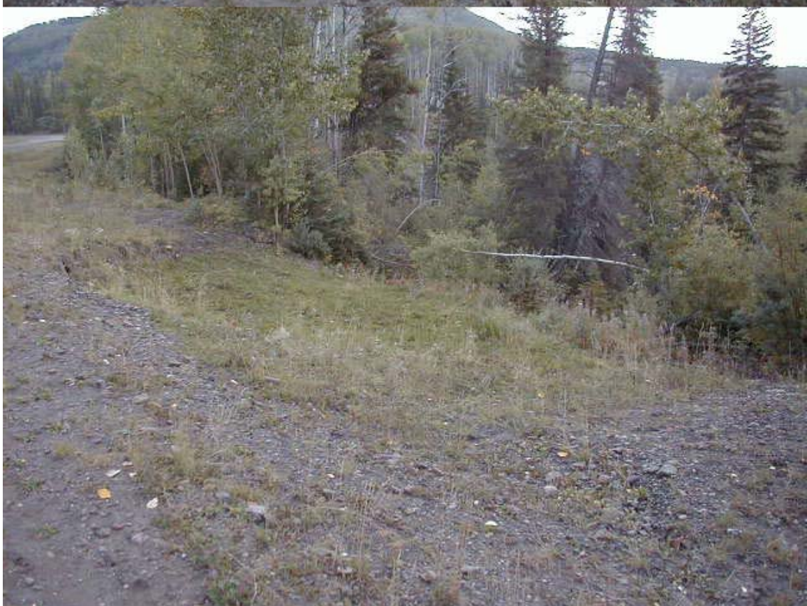
Looking north over second slide area about 30 m to the south. No culvert is present at this location but seepage was also observed.
