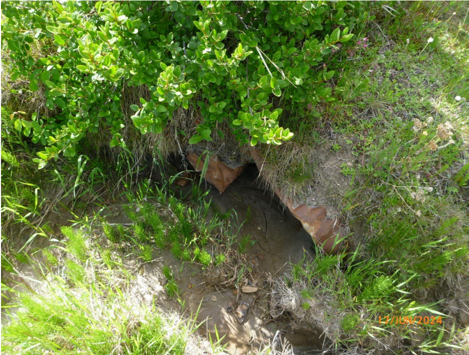
Photo 21 Damaged culvert or metal debris observed at the base of the erosion gully. Photo taken June 17, 2024.
