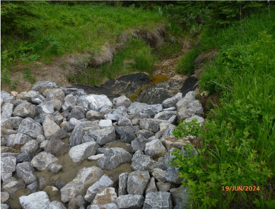
Photo 11 Downstream limit of the riprap-lined channel. The non-woven geotextile extends past where the Class 1 riprap was placed. Photo taken June 19, 2024, facing north.
