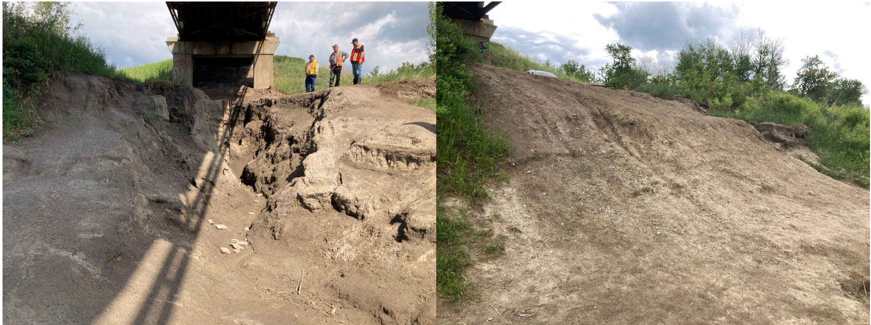
Photo 20 Large erosion gully on the east riverbank below the bridge was backfilled between the 2021 and 2024 inspections. Left and right photos taken June 24, 2021, and June 19, 2024, respectively.
