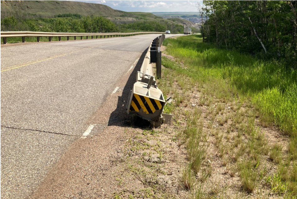
Photo 11 Impact attenuator for the south (eastbound ) guardrail is damaged and was likely damaged during snow clearing activities. Photo taken June 19, 2024, facing east.
