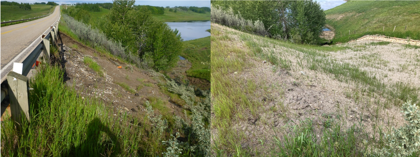
Photo 1 An overview of the C073 slide area from the north (westbound) shoulder of Hwy 580, before and after repairs. Photos taken July 10, 2019 and June 23, 2021 facing west and northwest, respectively.
