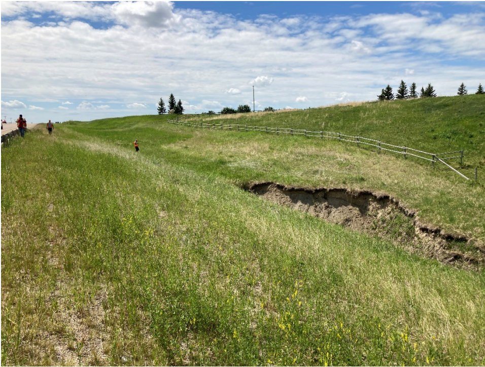
Photo 5 Erosion site approximately 4.7 km north of Carstairs, in the west (southbound) ditch of Hwy 2A. Photo taken June 23, 2021 facing southwest.
