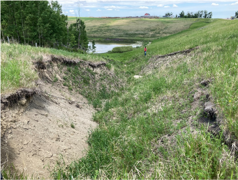
Photo 7 The sides of the erosion gully are near-vertical, and the depth of the erosion gully decreases as it progresses north. Photo taken June 23, 2021 facing northwest.
