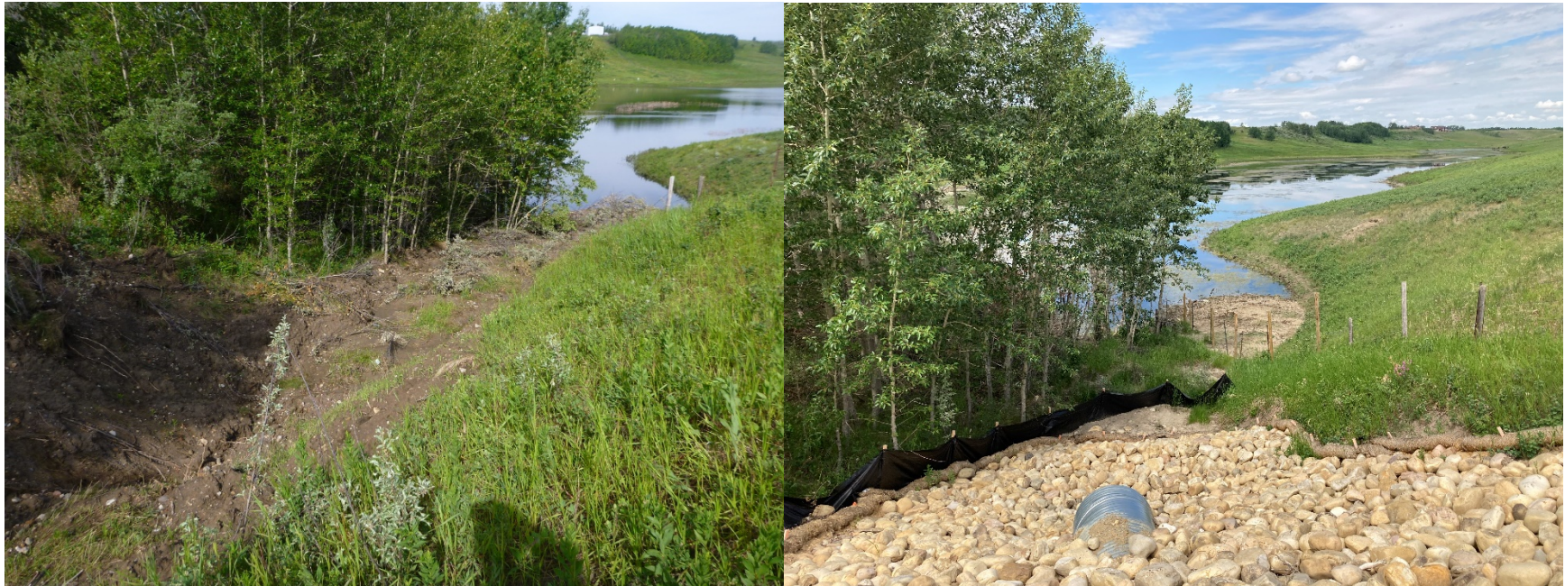
Photo 2 Area near Carstairs Creek where failed material from the C073 slide sloughed into when the embankment failed in 2019, before and after the 2020 repairs. Photo taken July 10, 2019 and June 23, 2021 facing northwest.
