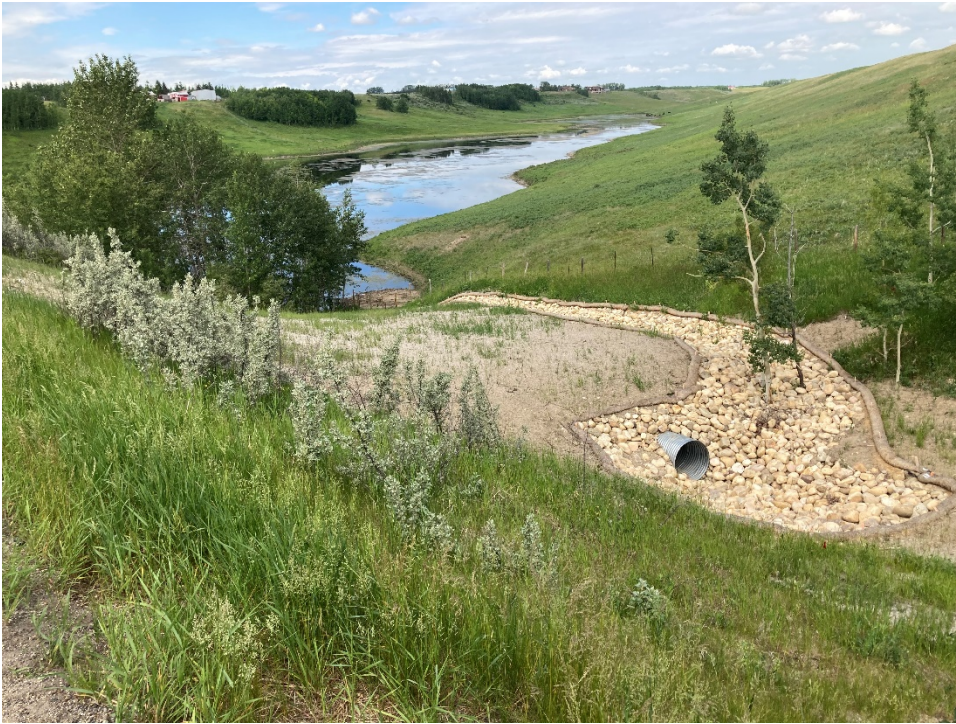
Photo 3 The east side of the slide repair, 900 mm diameter CSP culvert inlet, riprap apron, and overflow channel. Photo taken June 23, 2021 facing northwest.
