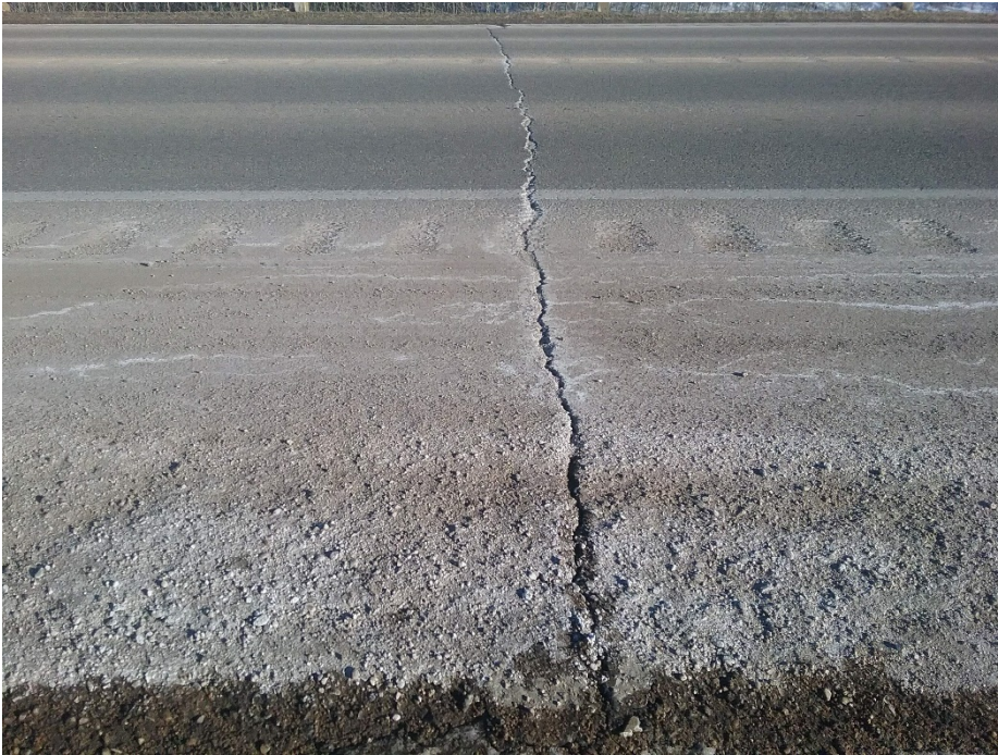
Photo 5 Transverse pavement crack extending entire width of highway. Photo taken on February 28, 2018.
