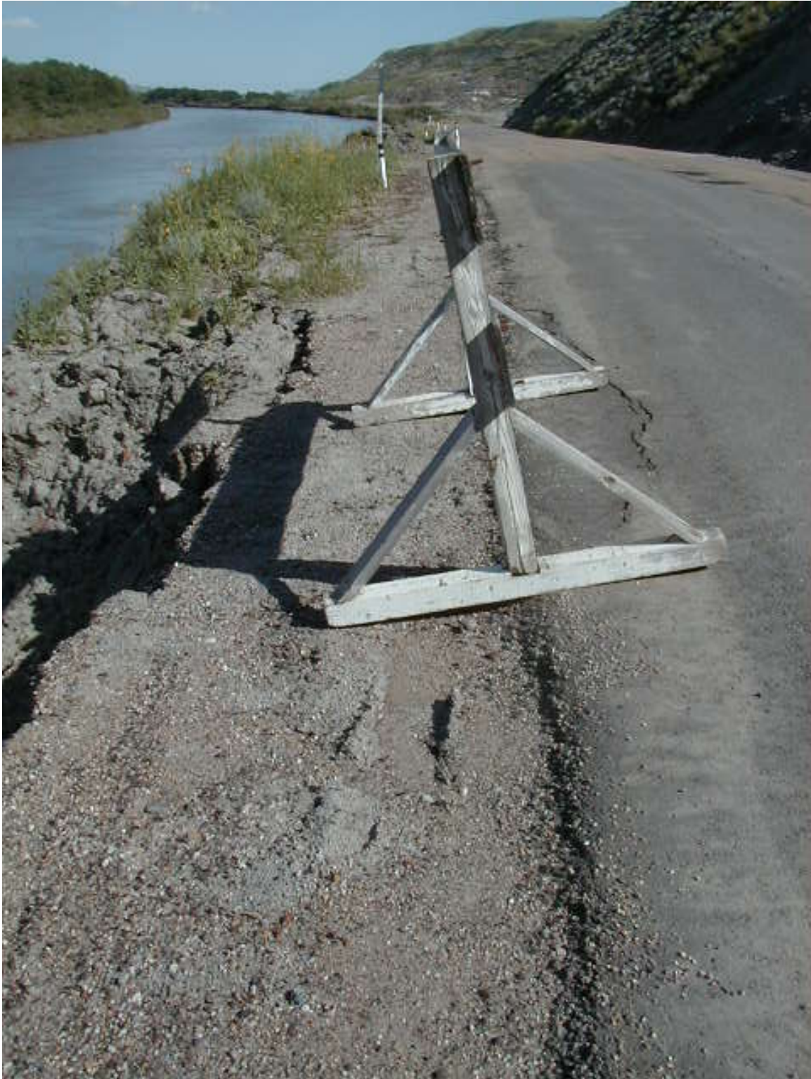
Observed cracking in pavement
