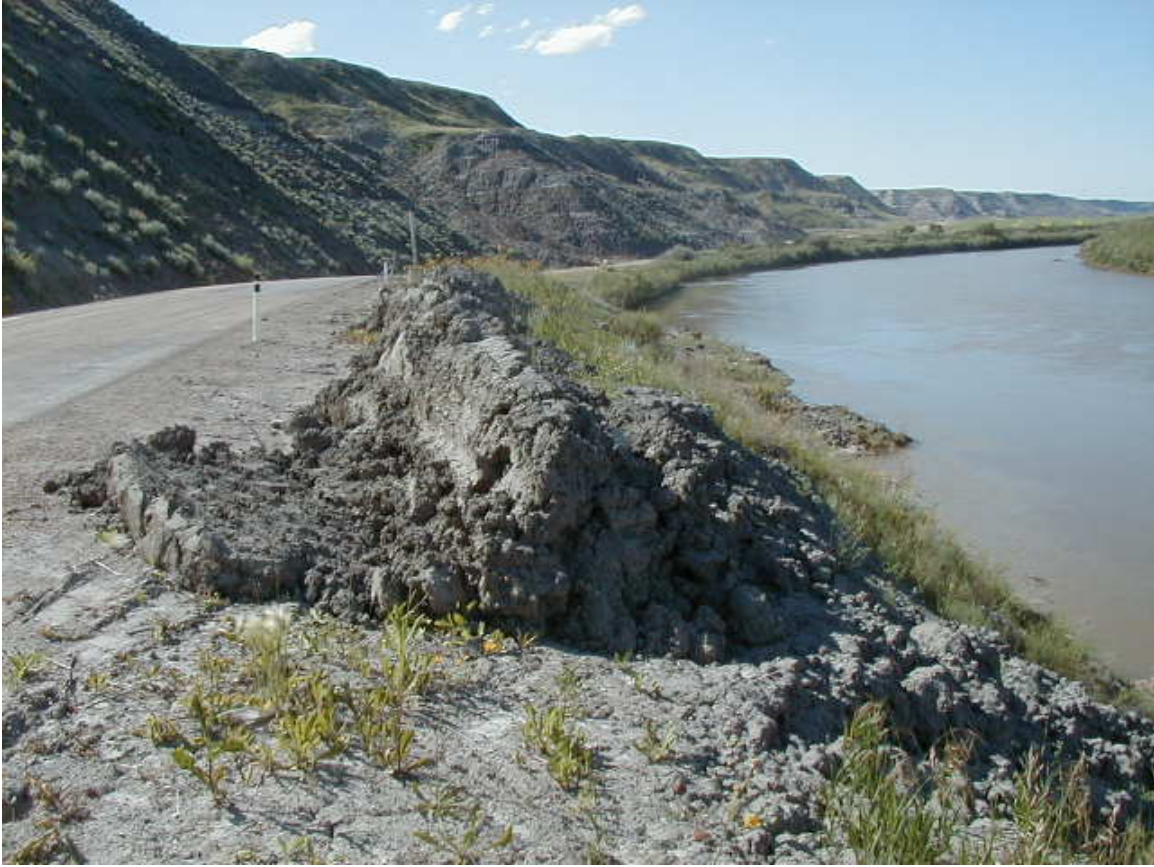
Ditch spoil pile placed at crest of slope
