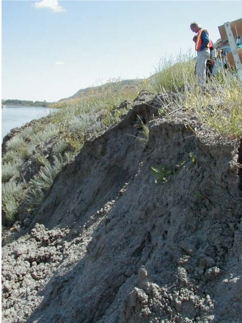
Steep scarps to the south of the main slide. The area of instability extends for a width of about 14 m.
