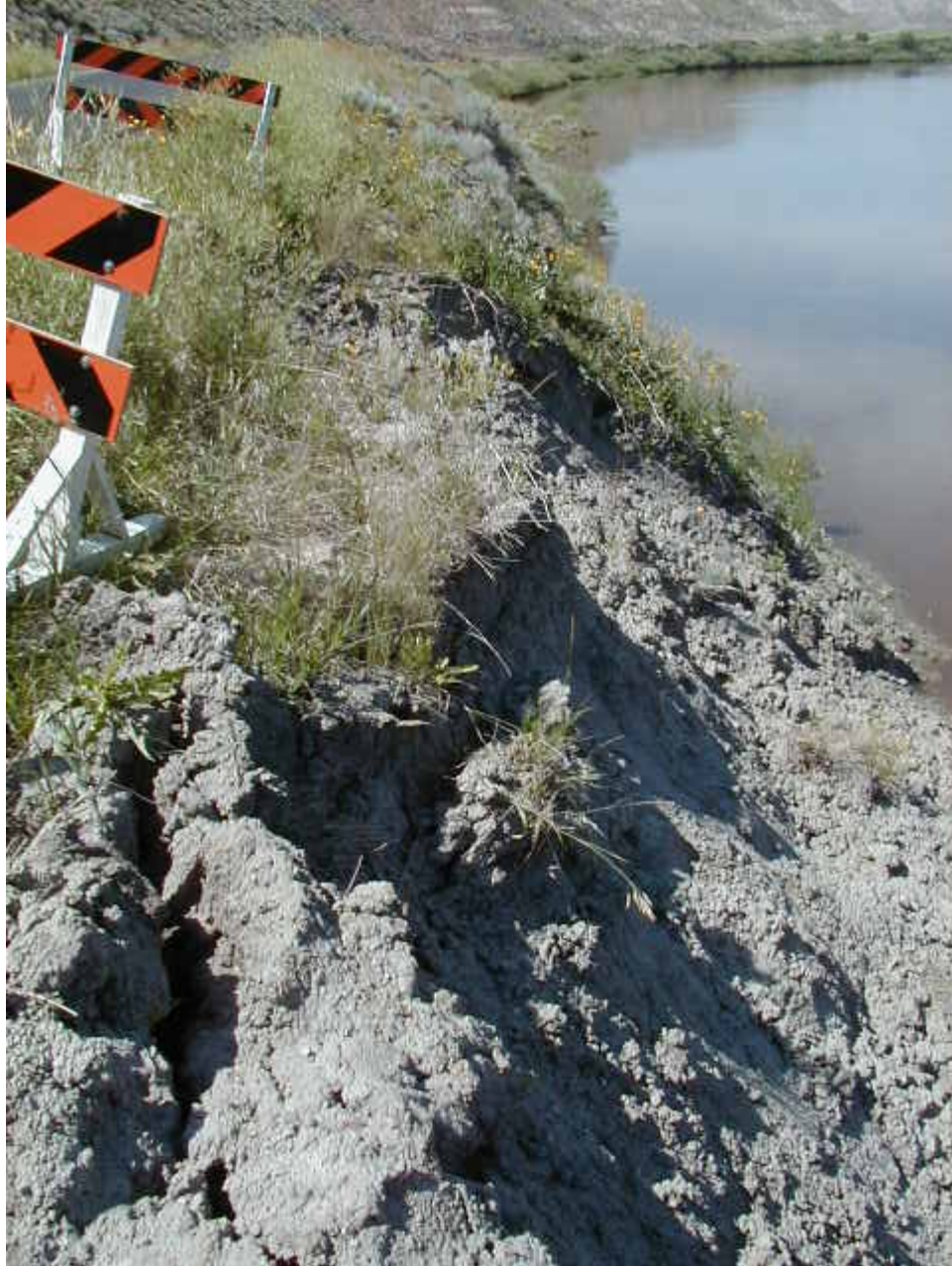
Looking north. Note cracks in lower left corner of photo.
