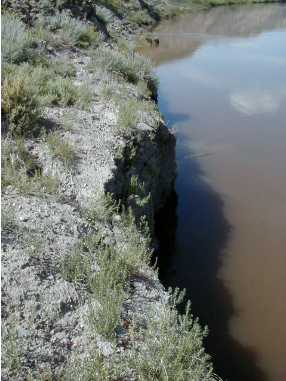
Typical erosion along riverbank.
