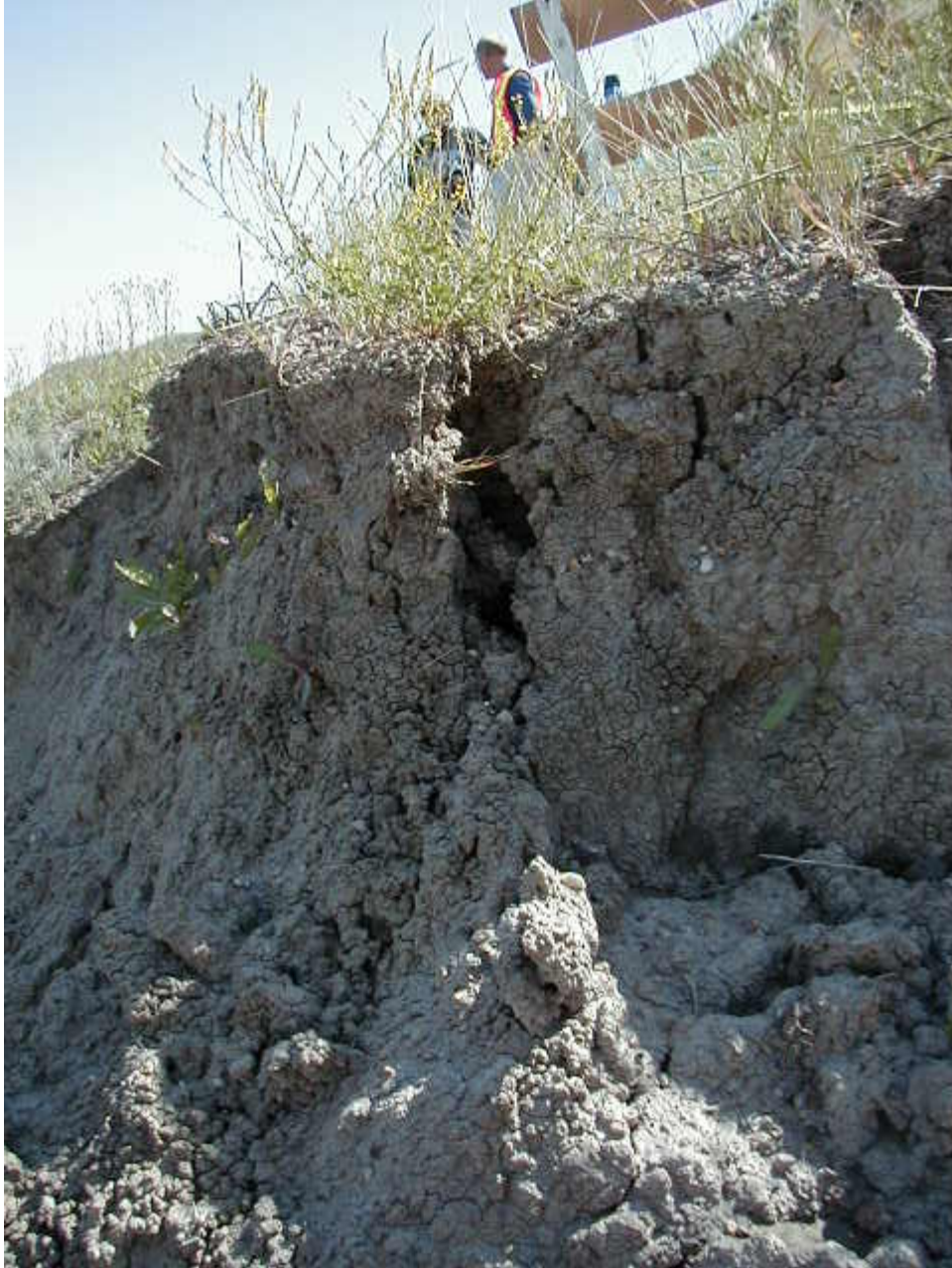
Looking south. Note cracking of slope.
