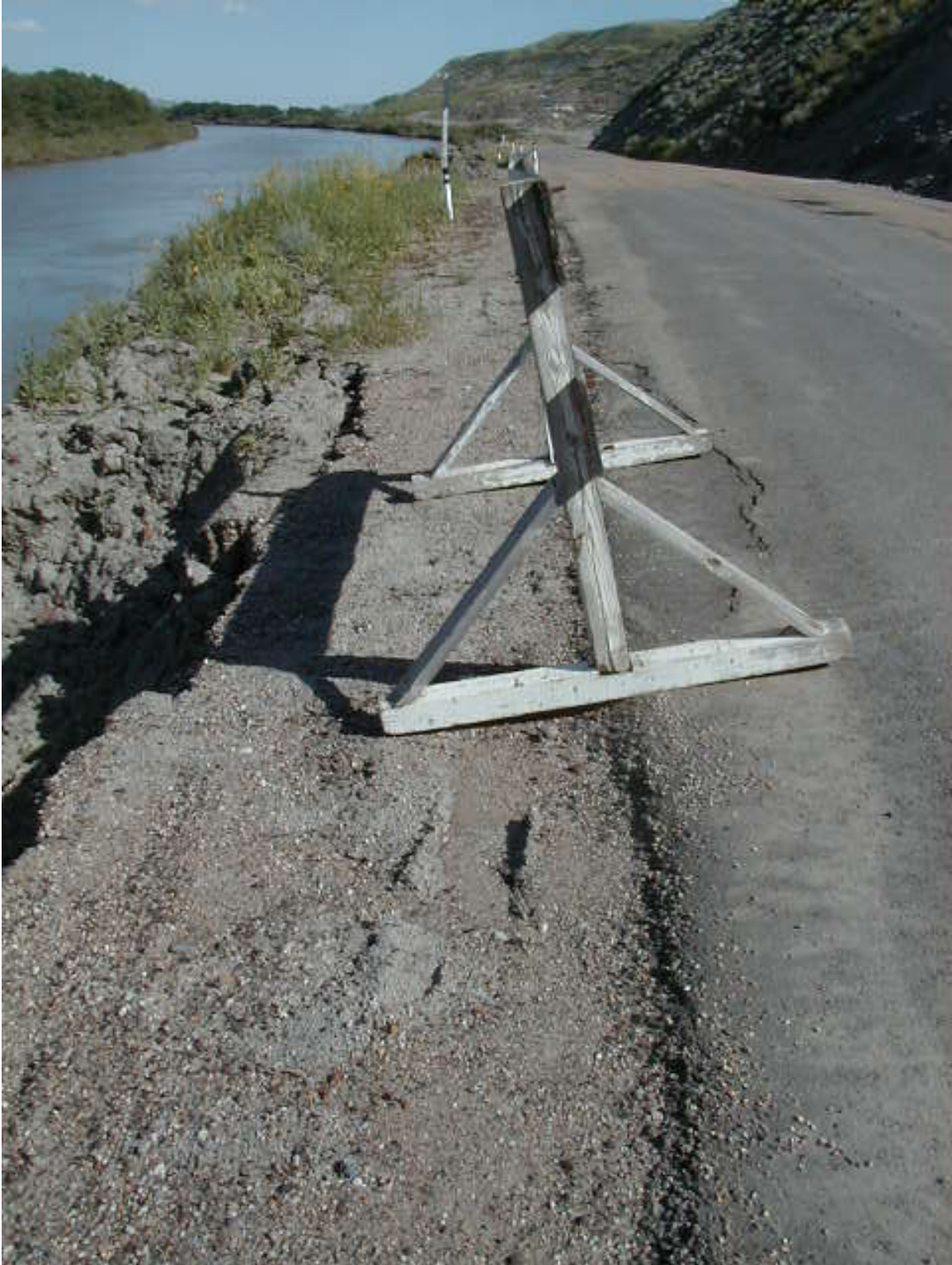
Observed cracking in pavement
