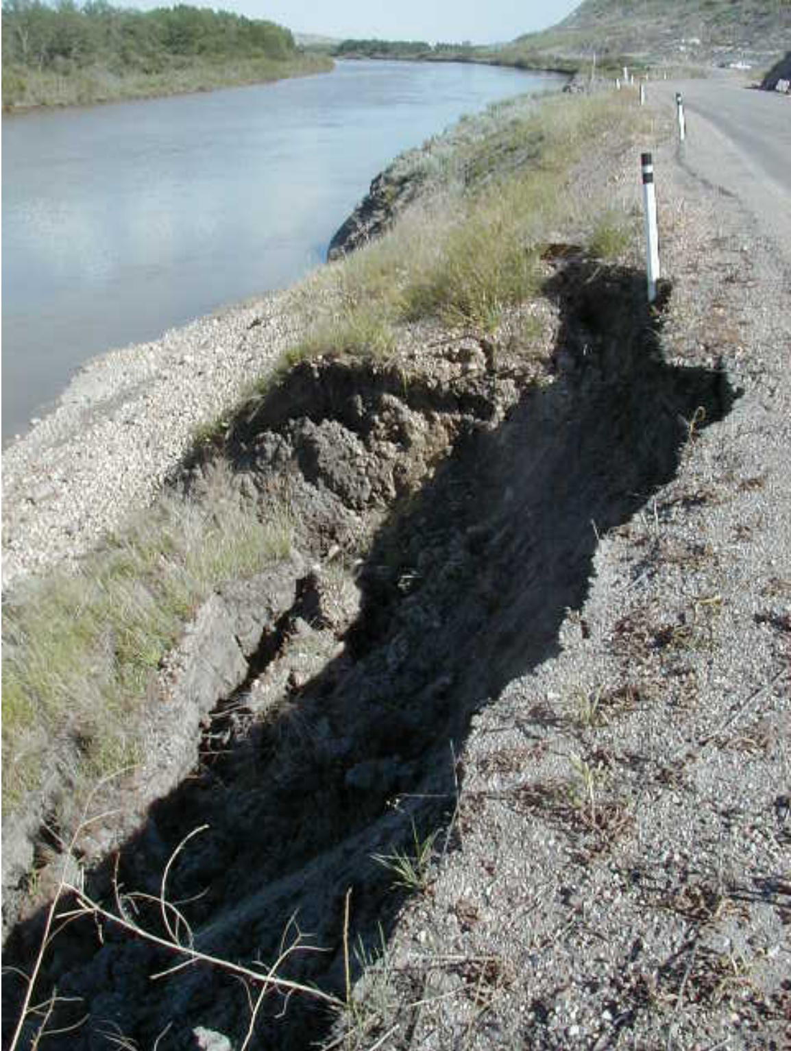
View of new slump section at north end of gravel berm due to June 2005 flooding. Width is about 13 m.
