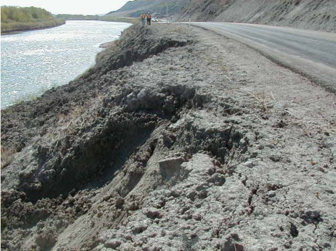
Two new unstable areas have appeared with scarps regressing towards the pavement
