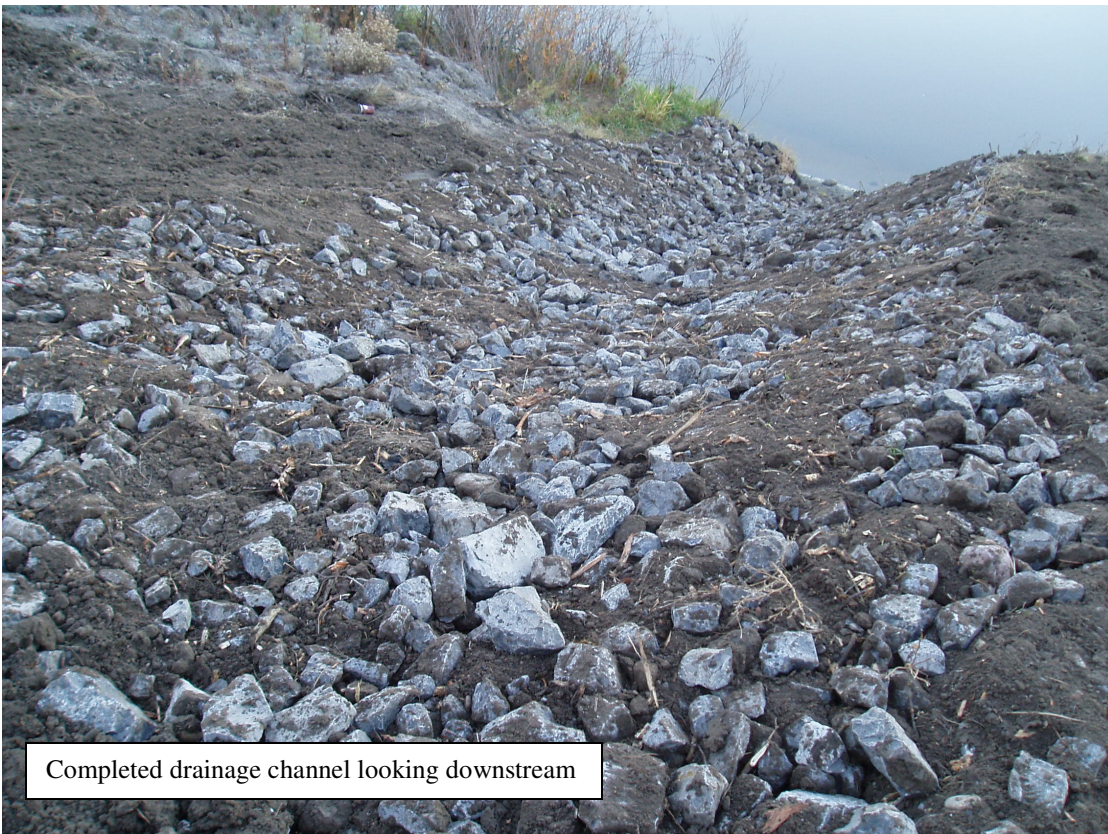
Construction of rock-lined drainage channel at north end of repair area looking downstream
