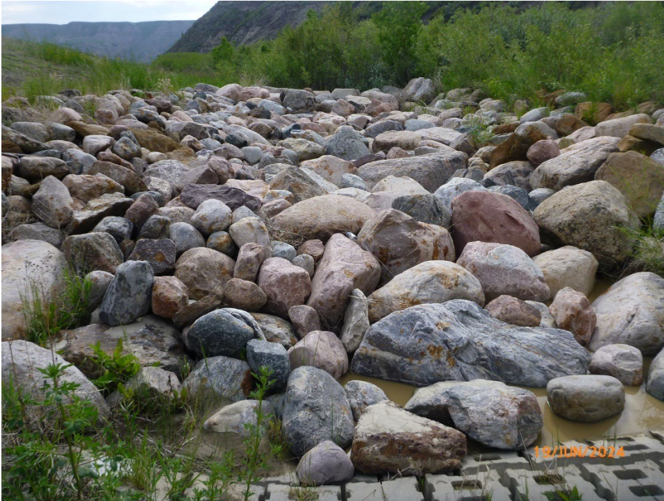
Photo 9 Riprap energy dissipation structure consisting of Class 3 riprap at the east extent of the south (eastbound) ditch repair. Photo taken June 19, 2024, facing southeast.
