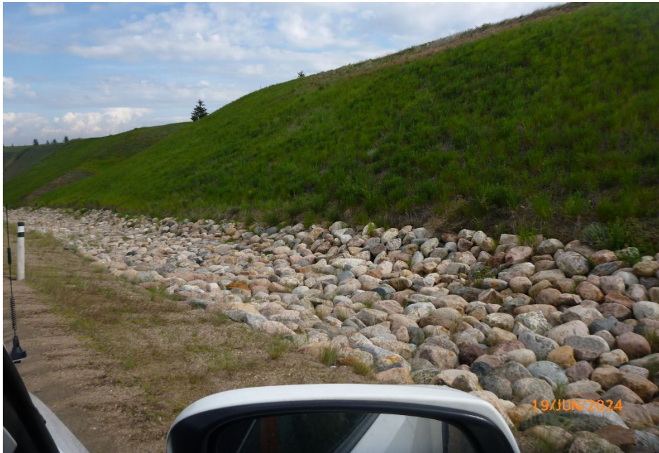
Photo 12 Riprap armoring in the north (westbound) ditch east of the Morrin Bridge. Photo taken June 19, 2024, facing north.
