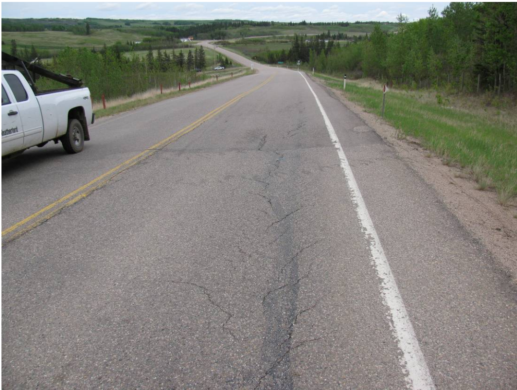
Photo #5 5-10mm wide open cracks outside the western limit of the patched area, looking east
