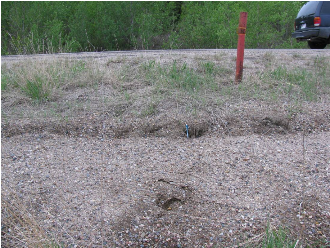
Photo #8 Settlement of gravel in contact with the wall downslope face by up to 150 mm, looking south
