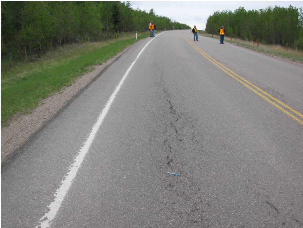
Photo #2 10-15 mm wide reflective crack on the highway EBL, looking west
