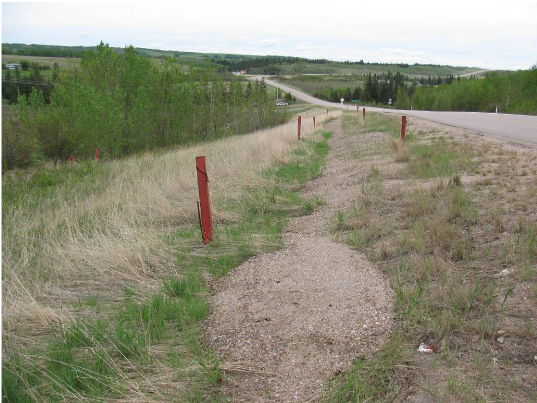
Photo #6 Gravel fill placed along the wall face in late 2009, looking west
