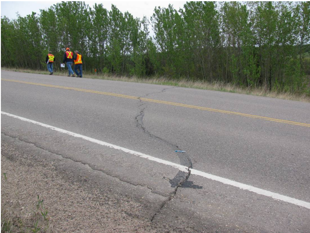
Photo #4 10-25 mm wide open arc-shaped crack at the western limit of the slide, looking north
