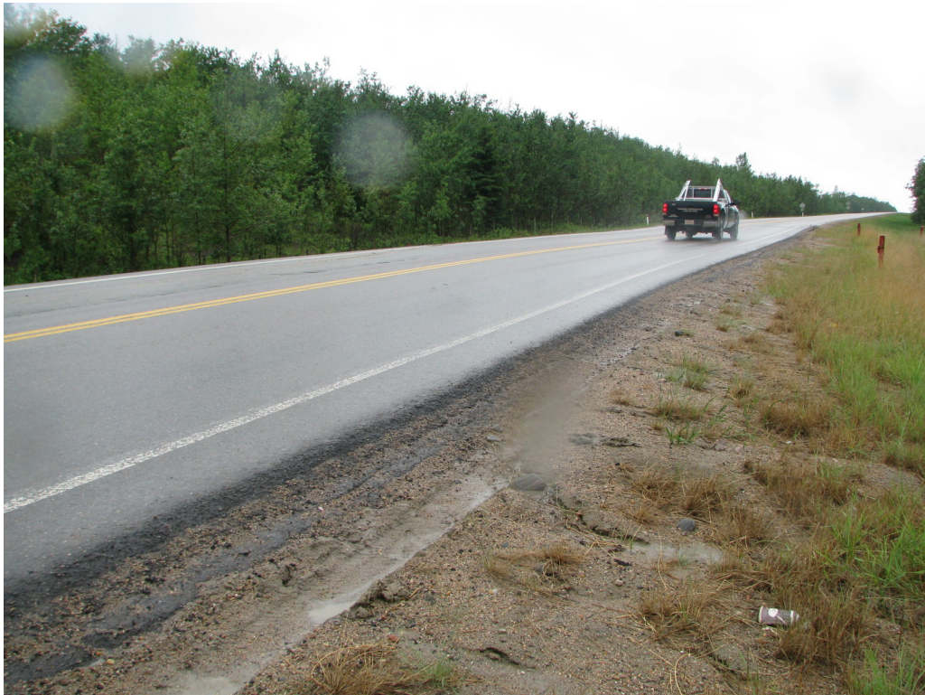
Photo #2 Looking southwest at the slight dip on the highway WBL, note the dip below the passing vehicle
