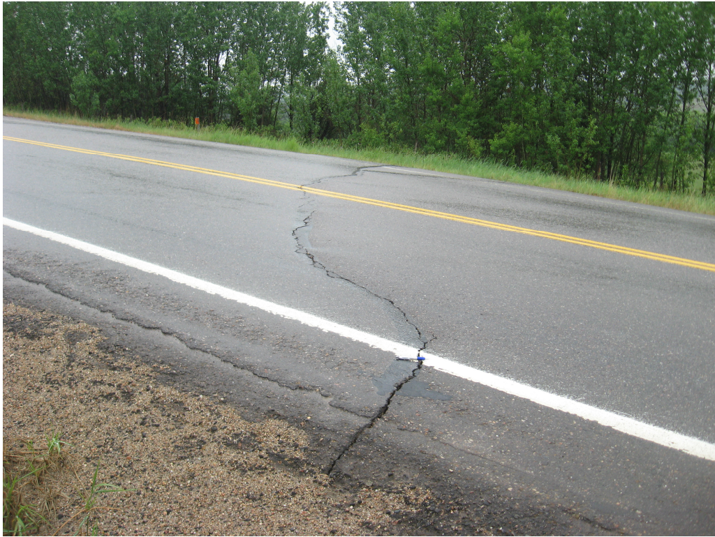
Photo #3 Open arc-shaped crack at the western limit of the slide, looking east
