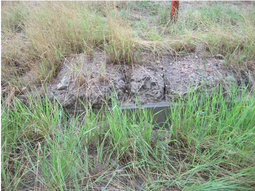
Photo #4 Existing crack along the downslope face of the wall, looking south
