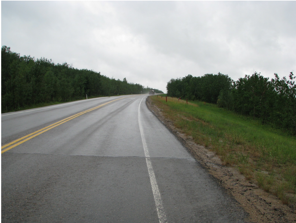
Photo #1 General view of highway surface at slide location, looking west
