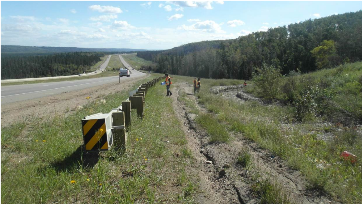
Photo #9 - Looking South along west side slope from north end of existing guardrail; note the presence of erosion rills on the side slope; surface flow has been eroding the slope surface; the slope should be graded along with using compost filter berms as needed to direct water into the armored ditch.
