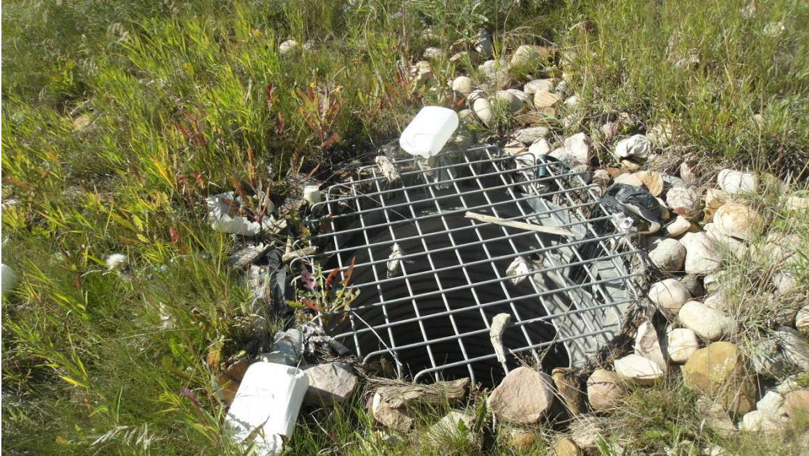
Photo #5 - Looking at median ditch drop pipe Grate; note the presence of minor trash around the grate; needs to be cleaned.
