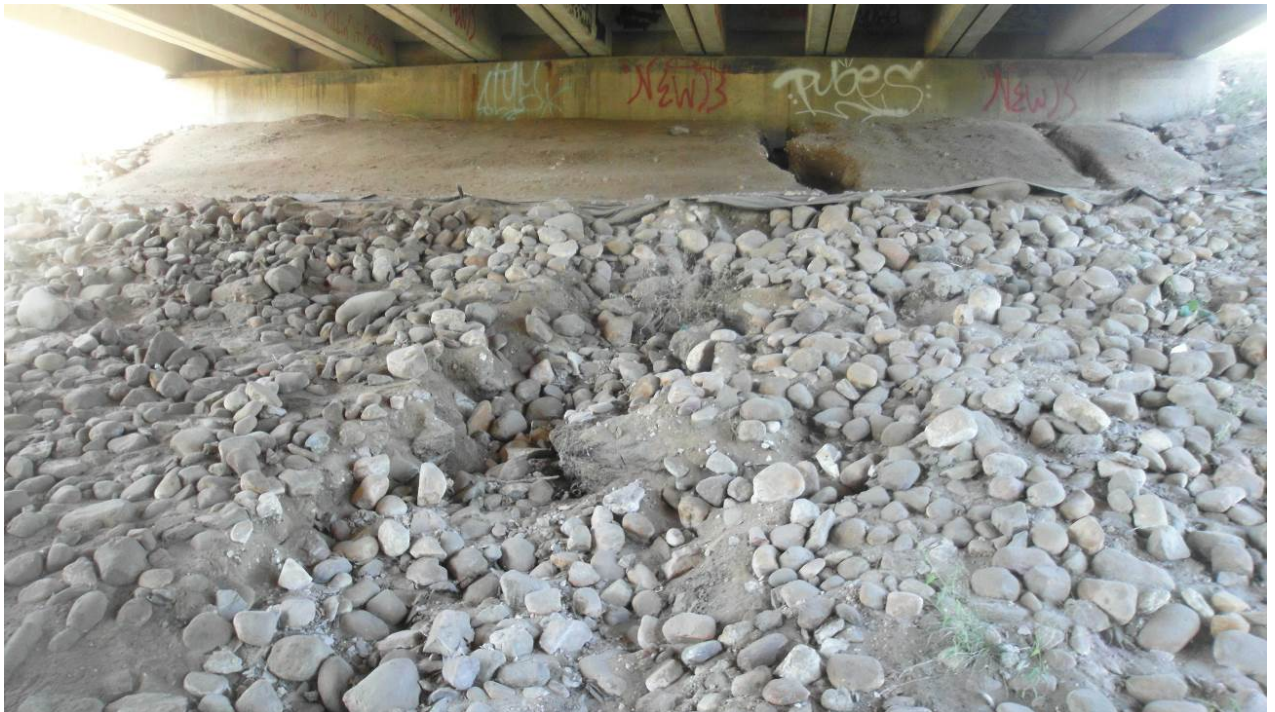
Photo #3 - Erosion gullies near the abutment seat and displaced riprap under the highway northbound lane bridge.
