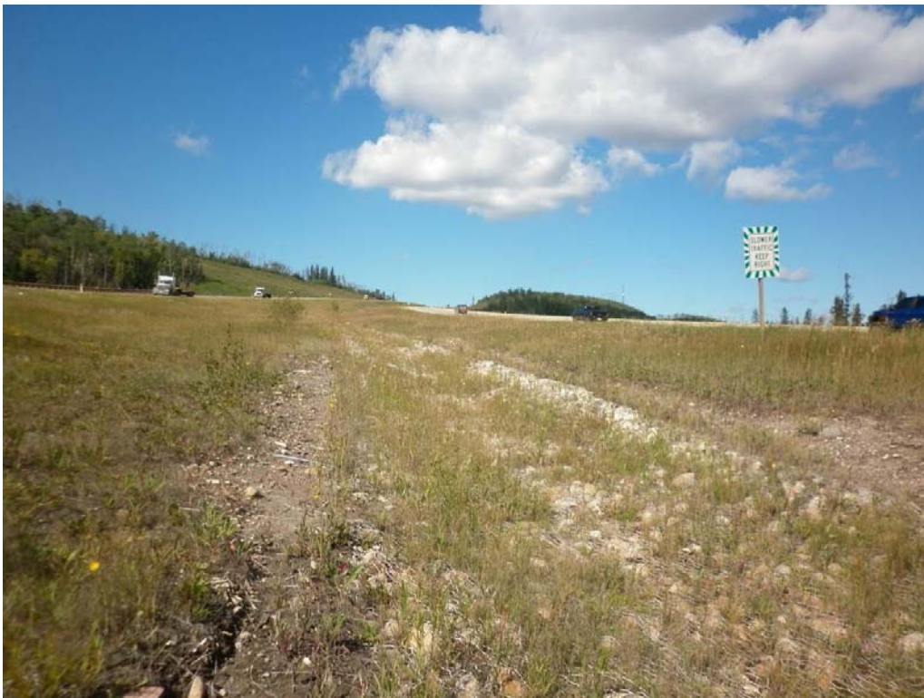
Photo #6 - Looking north at the median ditch; vegetation grew in the gabion mattress
