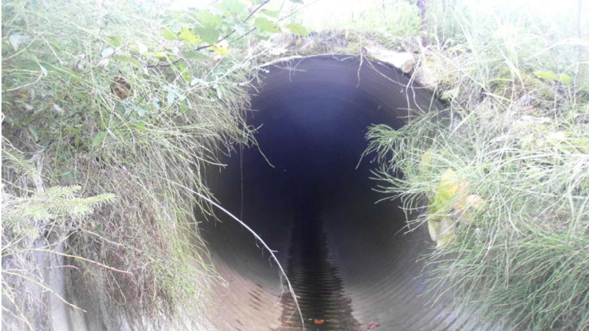
Photo #20 Looking inside one of the twin culverts from the inlet location.
