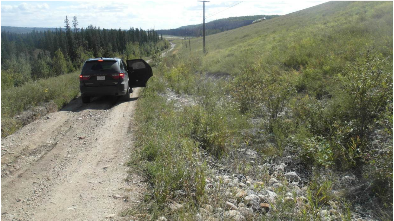
Photo #1 - Looking south at the gabion mattress from the upper part of east side slope
