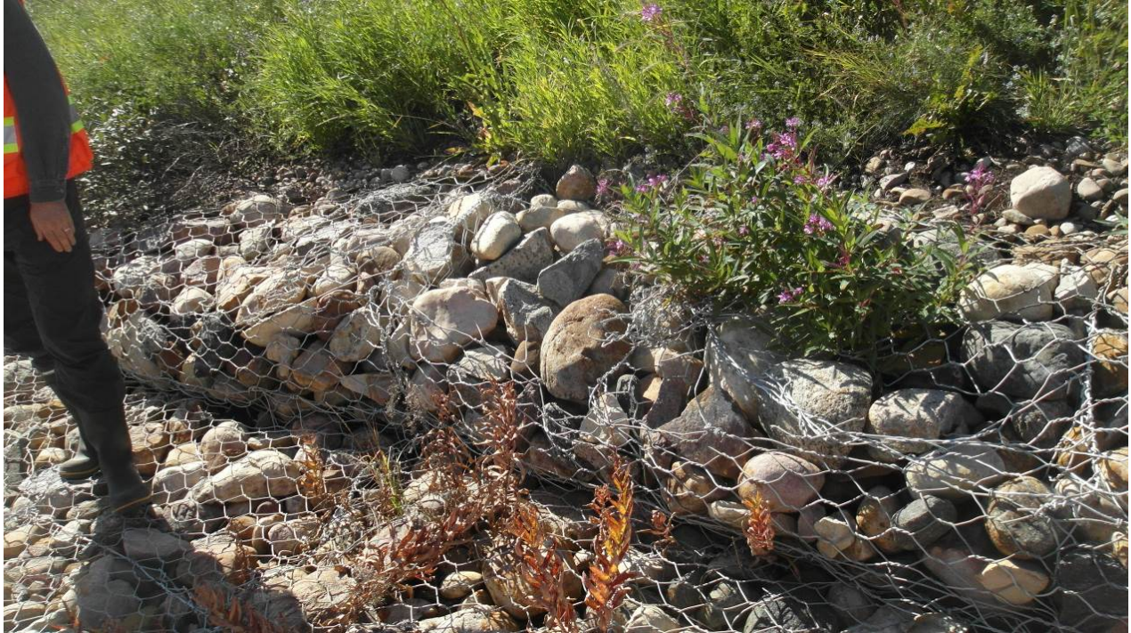
Photo#16 Looking west at a raptured gabion basket within the west ditch gabion channel; back slope is likely pushing against channel walls.
