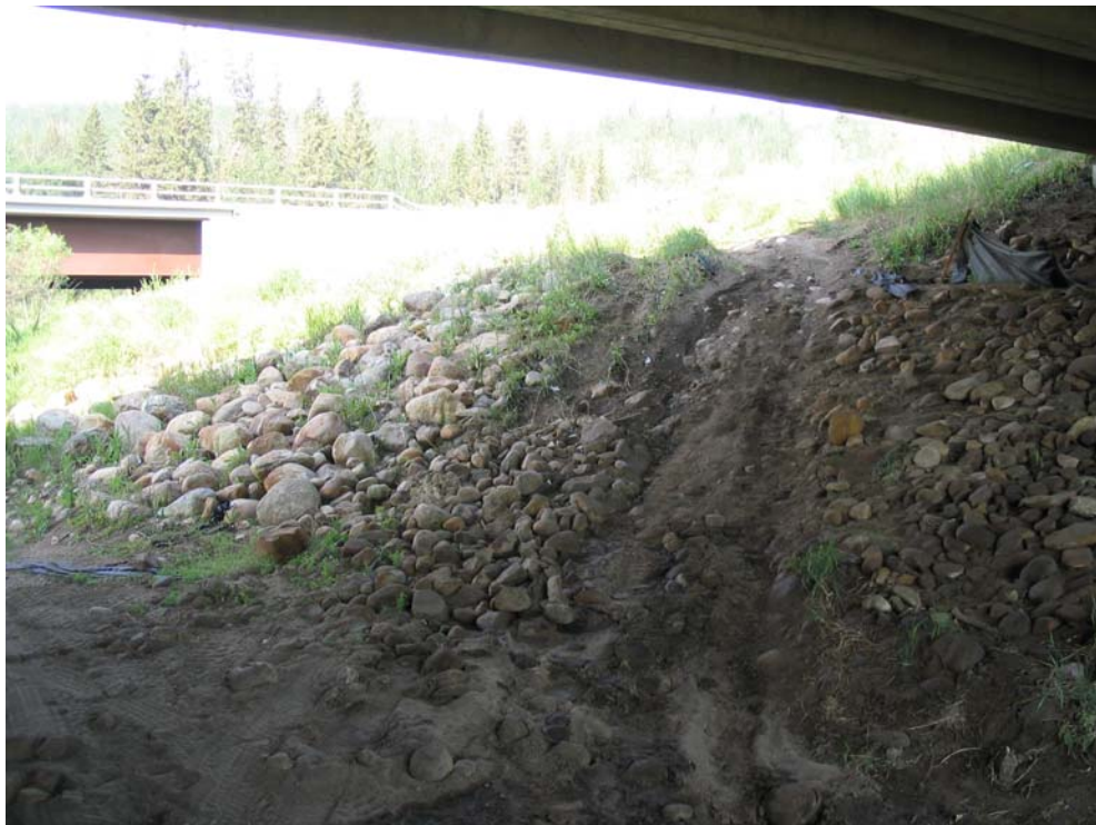
Photo 4 - Erosion Along a Quad Trail Under the Northbound Bridge.
