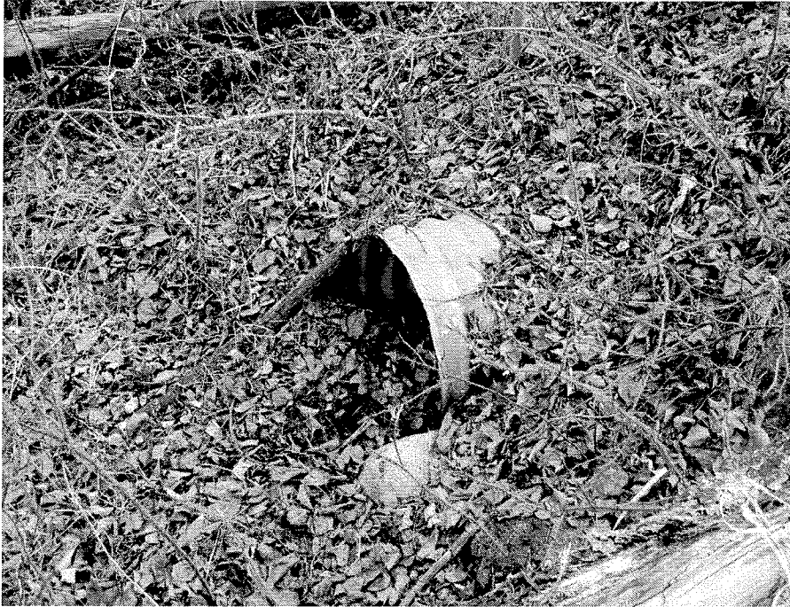
Photo 9- Looking at the outlet of the old highway 400 mm diameter CSP culvert- Note the debris inside and in the vicinity of the culvert.
