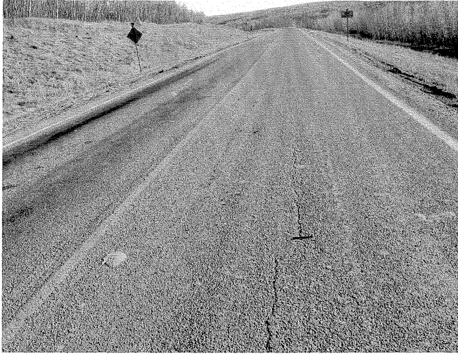
Photo 5 - Looking south at a longitudinal crack along highway SBL surface
