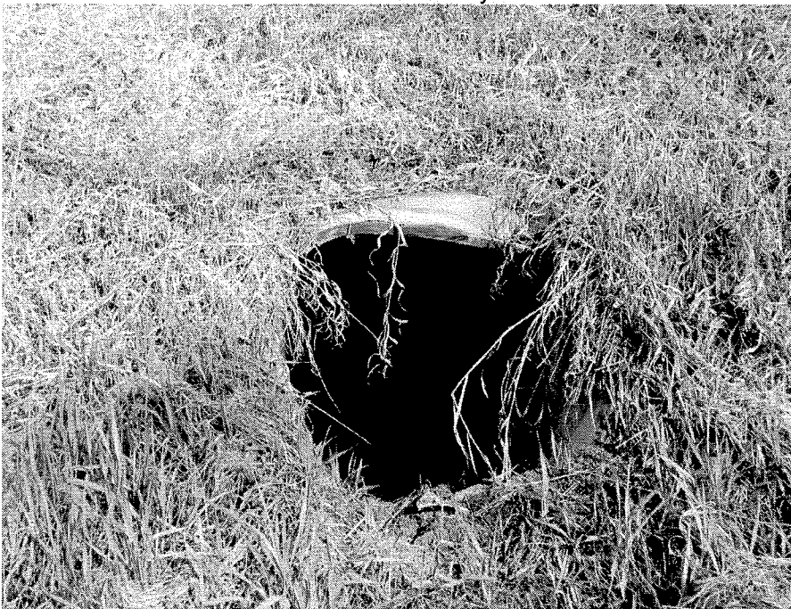
Photo 10- Looking at the outlet of the 600 mm diameter CSP culvert- The outlet is distorted and water is standing inside the culvert outlet
