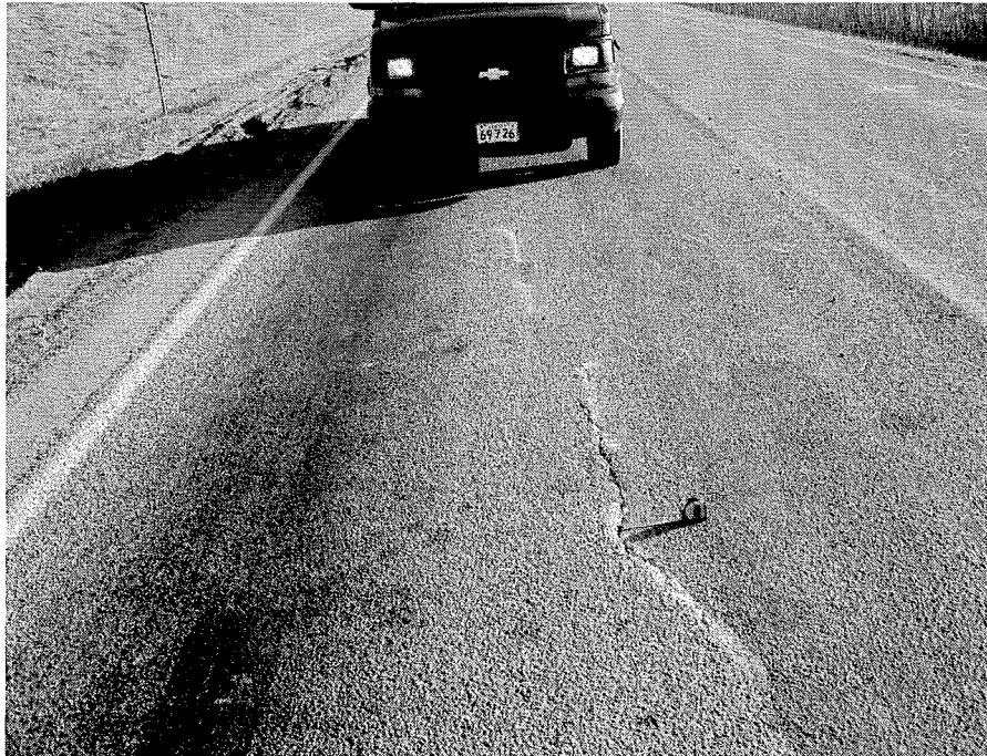
Photo 6- Looking south at a longitudinal crack along highway NBL surface
