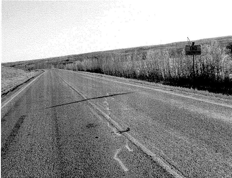
Photo 7 - Looking south at the southern diagonal crack of the slide
