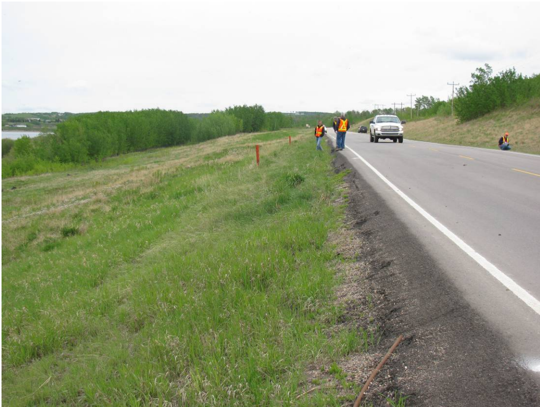
Photo #6 Looking at the highway side slope where the wall was constructed; note the growth of vegetation on the highway side slope (looking north)
