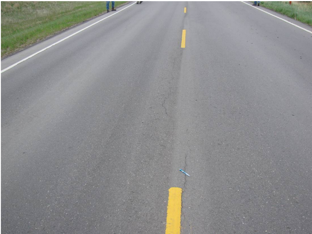
Photo #2 Looking south towards a reflective faint crack on the highway surface
