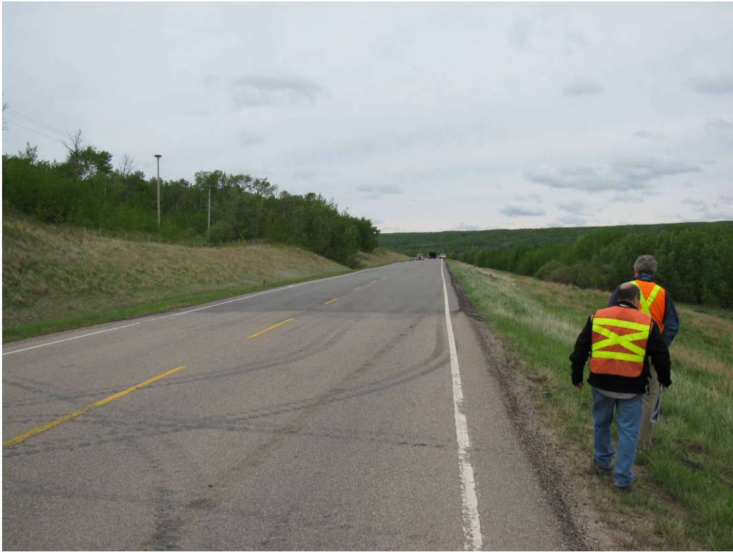
Photo #1 General view of highway surface at the slide repair location (looking south)
