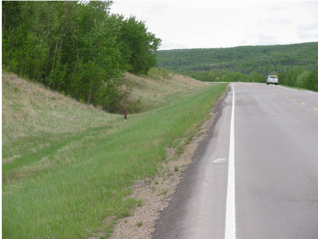
Photo #3 Looking south. There is a depression area along the former back scarp of the slide
