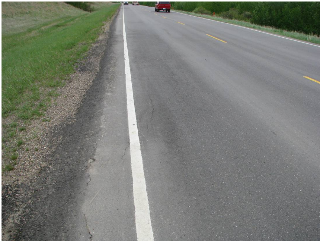
Photo #4 Looking south at reflective faint cracks on the highway NBL surface. The feathered end of the recent pavement patch is rough at this location
