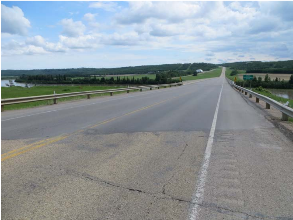
Photo#1 Looking south from the north side of the bridge at the ACP overlay
