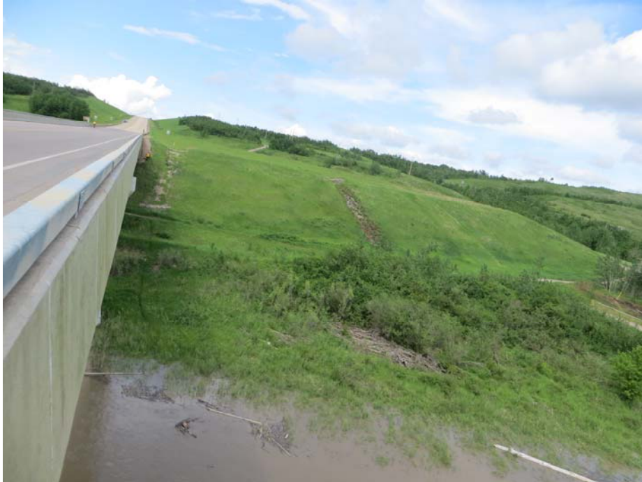
Photo#3 Looking north from the top of the bridge at the river valley and approach fill slopes; note the presence of two gabion mattresses along existing slope above the river valley slope
