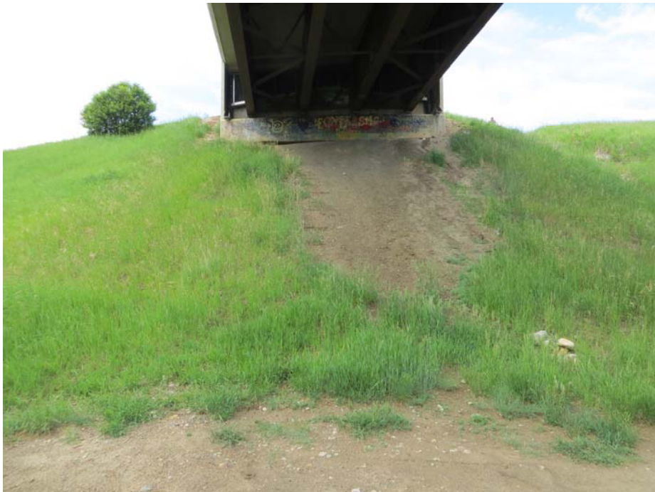
Photo#4 Looking north at the approach fill slope; note that the slope surface is partially bare of vegetation
