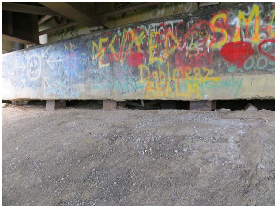
Photo#6 Looking north at north abutment seat; note the gap developed below the seat due to fill settlement
