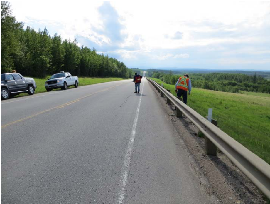
Photo#2 Looking northwest at a longitudinal reflective crack
