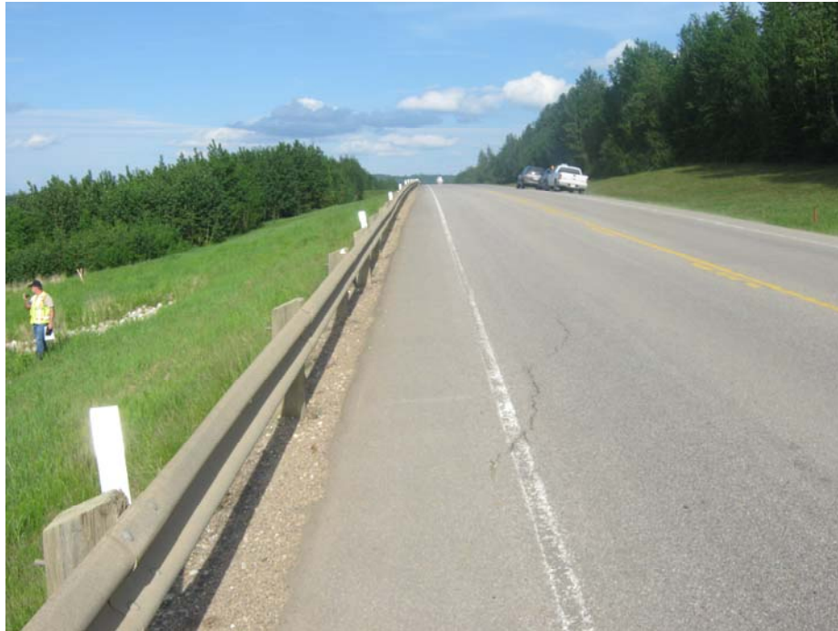
Photo#3 Looking northeast at a diagonal reflective crack
