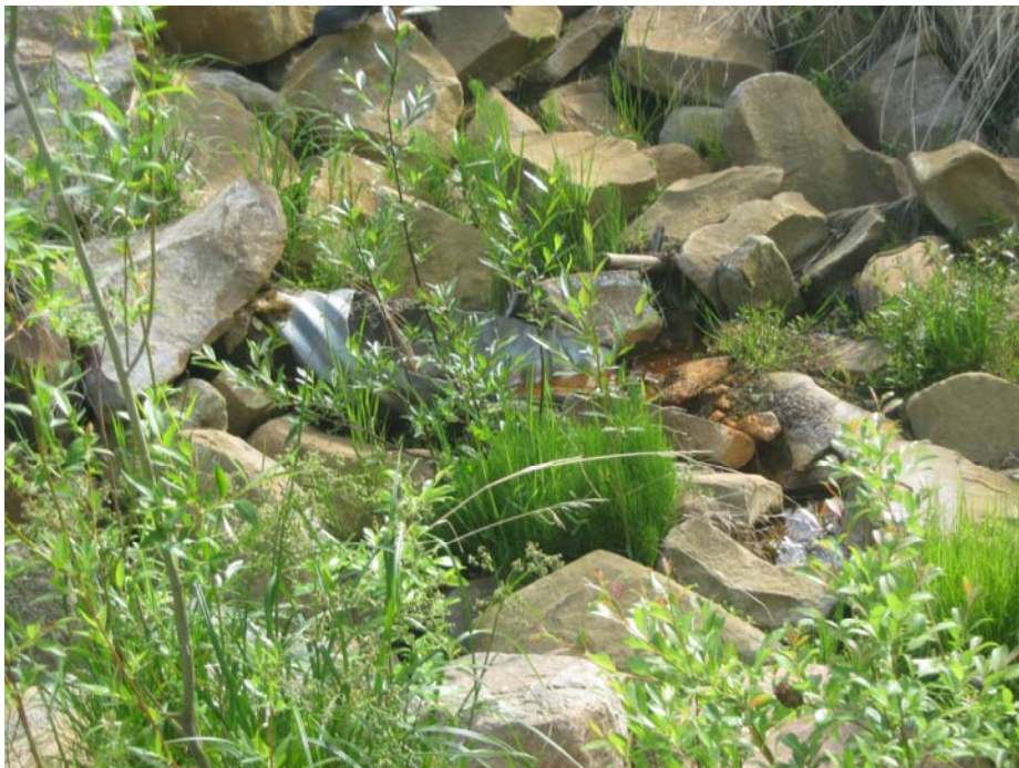
Photo#6 Looking at the outflow pipe from the bottom of the slope
