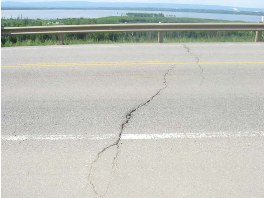
Photo#1 Looking northwest at a diagonal crack near the northeast limit of the site
