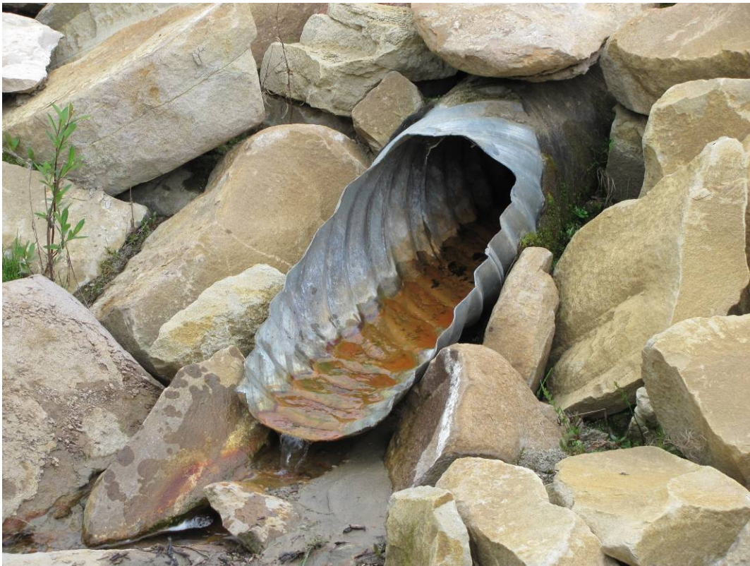
Photo#5 Looking at the outlet flow pipe from the bottom of the slope
