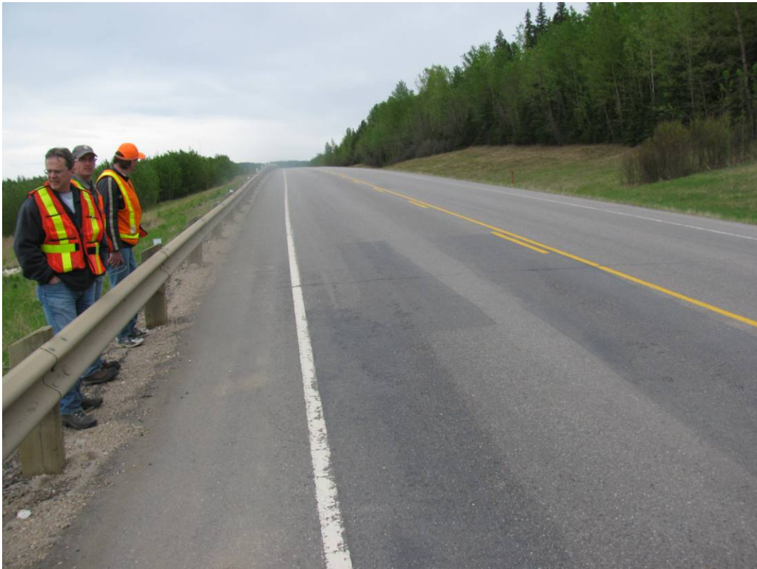
Photo#2 General view of the highway surface at the sealed crack location, looking northeast
