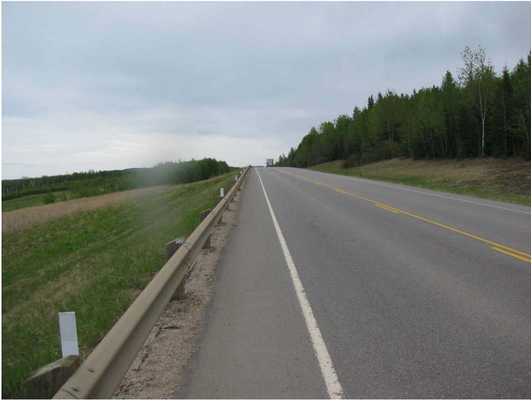
Photo#1 General view of highway surface conditions, looking northeast
