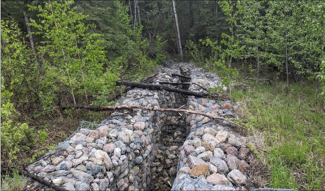
Photo No.13 – Gabion basket channel performing satisfactorily but showing signs of distortion
