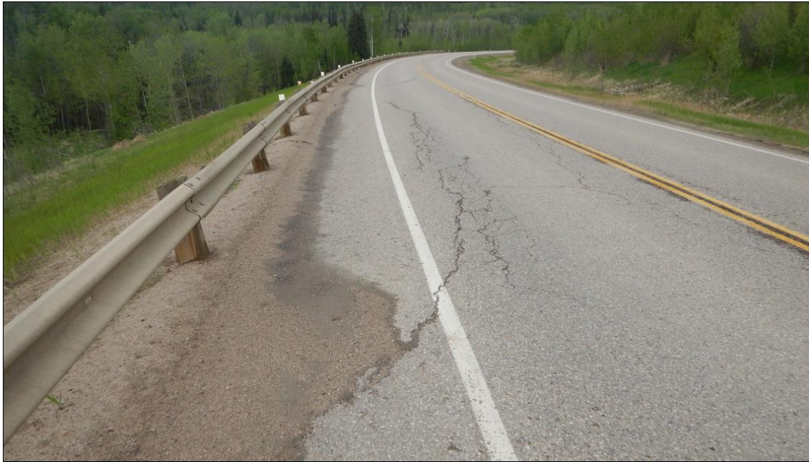
Photo No.3 - Looking north from the southern limit of the site at 30-50 mm wide diagonal Crack B, no drop
