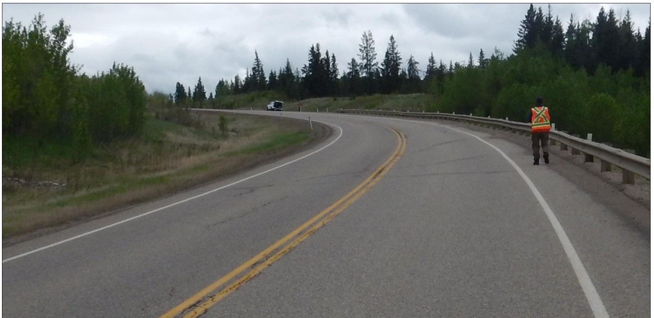
Photo No. 6 – Looking south at arc-shaped reflective Crack D
