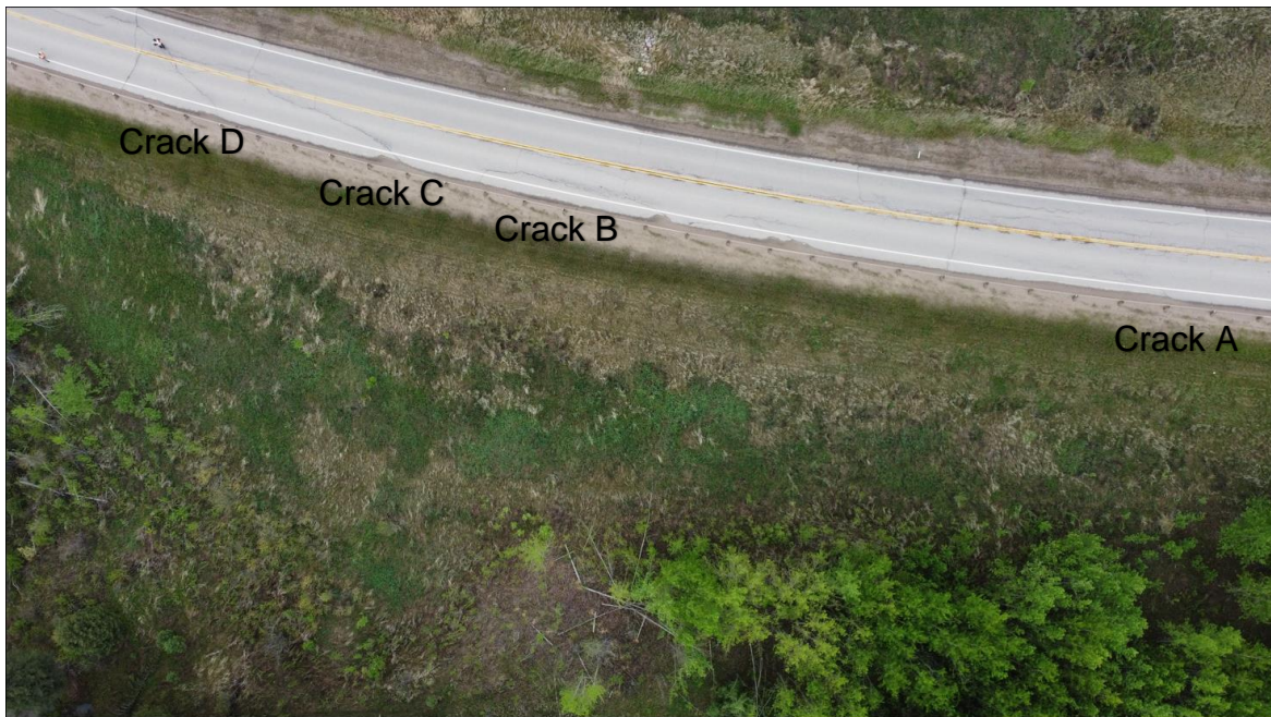
Photo No. 7 – Aerial photo showing Cracks A, B, C, and D
