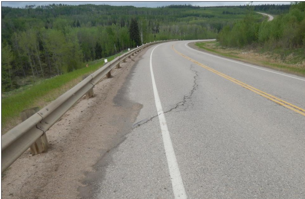
Photo No.4 – Looking north at the arc-shaped reflective Crack C (50 -100 mm wide, 15 mm drop)
