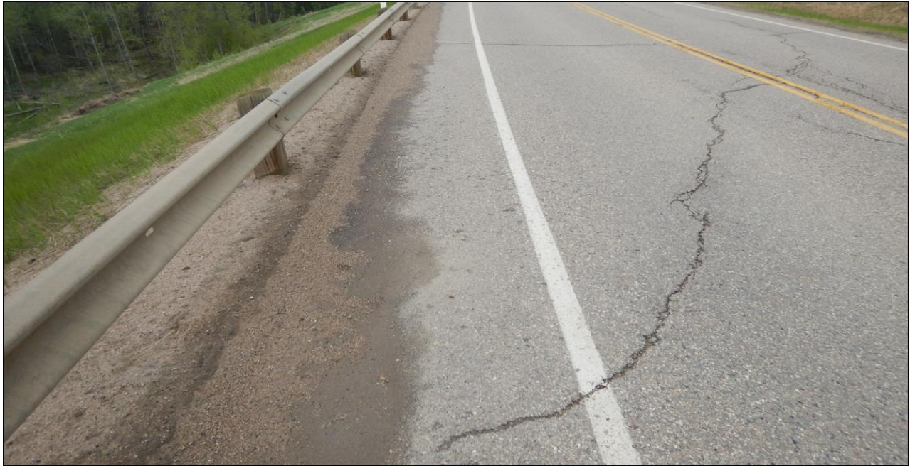
Photo No. 5 Looking north at the arc-shaped reflective Crack D (50-90 mm wide)
