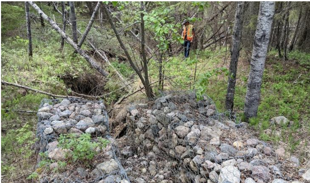
Photo No.10 – Looking north at erosion and fallen trees beyond the mouth of the gabion basket channel
