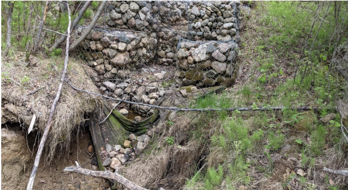
Photo No.9 - Looking at the mouth of the gabion basket channel. Note erosion around and below the base of the gabion basket
