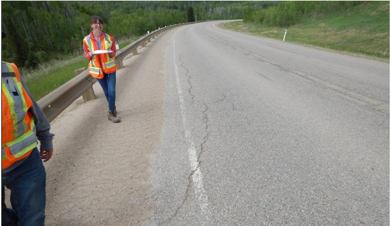
Photo No.2 - Looking north from the southern limit of the site at 10 mm wide diagonal Crack A
