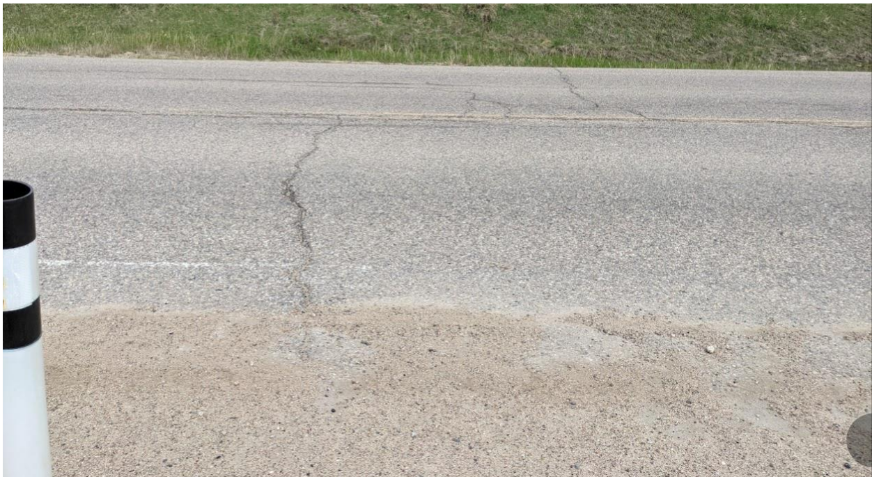
Photo No.6 – Looking east at a 10 mm wide transverse crack near the southern limit of the site
