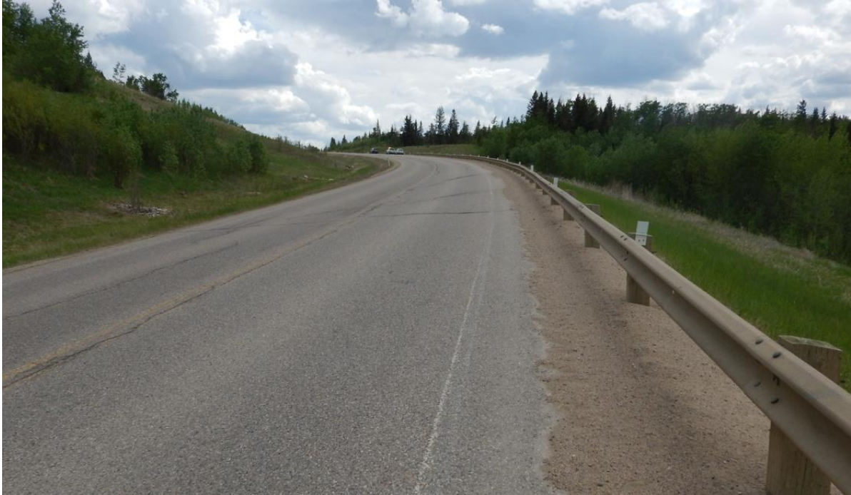
Photo No.5 – Looking south at a 20-30 mm wide arc-shaped reflective Crack D
