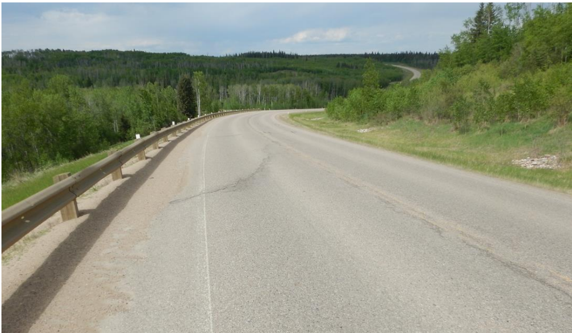
Photo No.4 – Looking north at a 20-40 mm wide arc-shaped reflective Crack C
