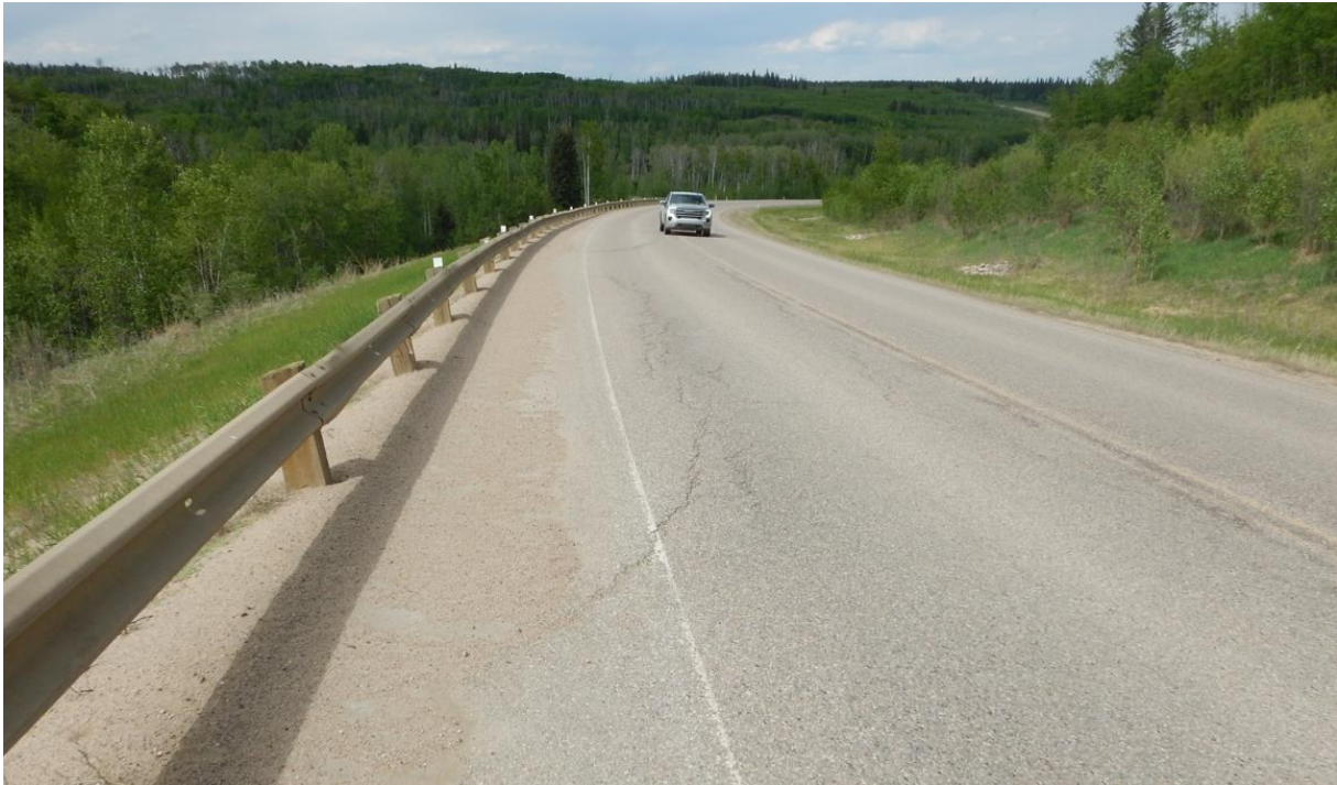
Photo No.3 - Looking north from the southern limit of the site at 10 -40 mm wide diagonal Crack B
