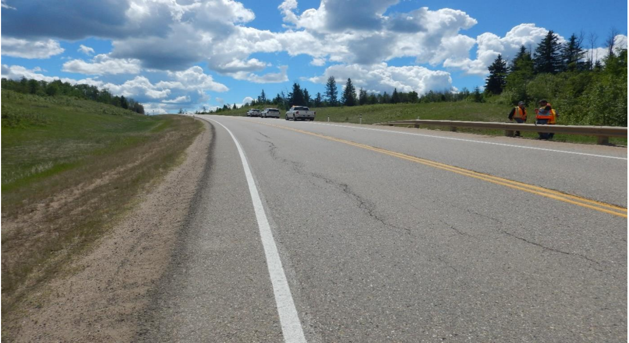
Photo No.1 - Looking south from the southern limit of the site at longitudinal cracks on the southbound lane
