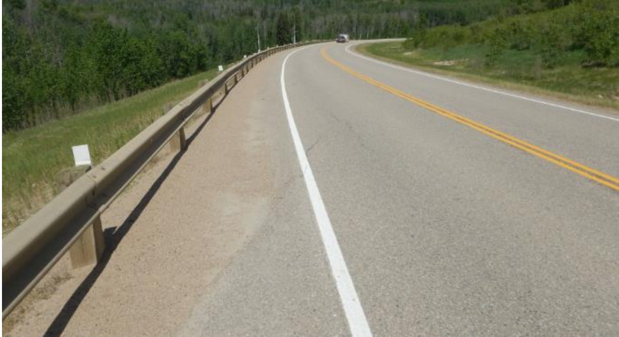
Photo No.1b - Looking north from the southern limit of the site at 10 -30 mm wide diagonal Crack B
