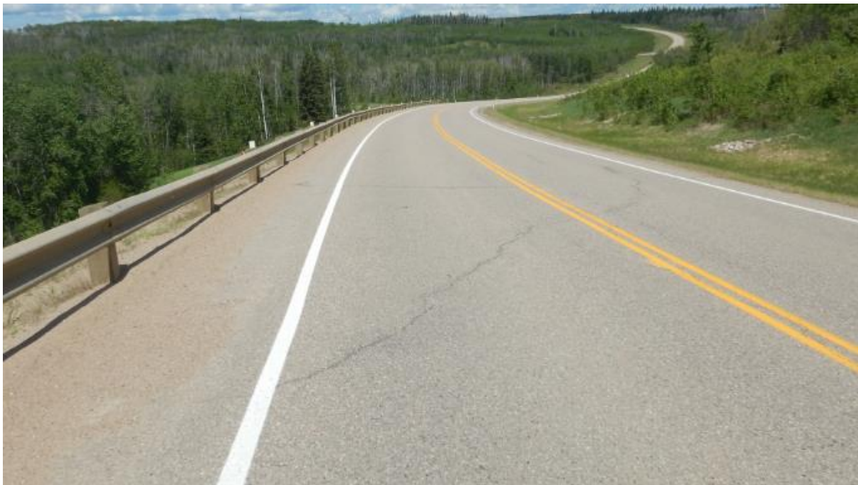
Photo No.4 - Looking north at a 10-30 mm wide arc-shaped reflective Crack D
