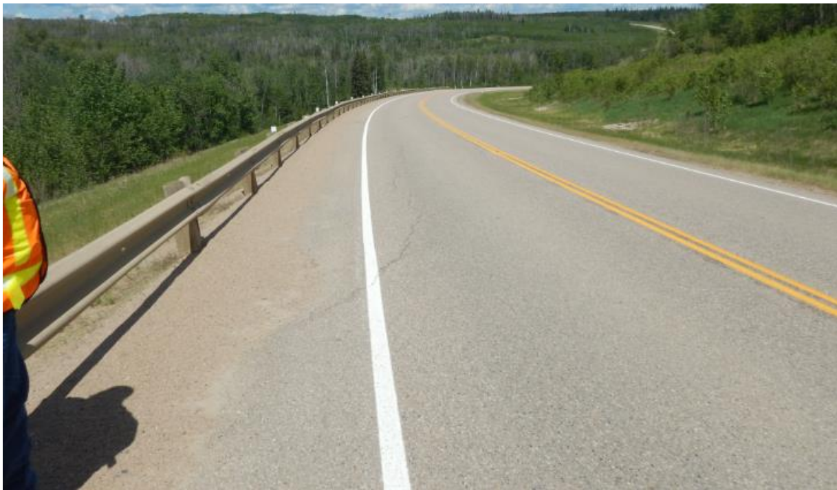
Photo No.2 - Looking north at a 10-40 mm wide arc-shaped reflective Crack B
