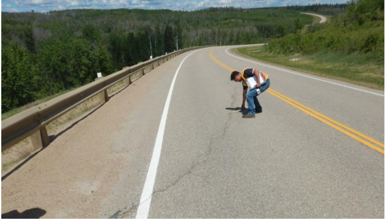
Photo No.3 - Looking north at a 10-40 mm wide arc-shaped reflective Crack C on the highway surface
