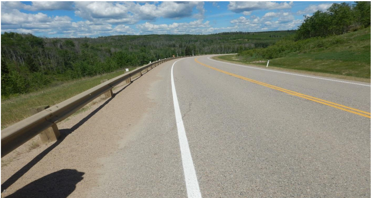
Photo No.1a - Looking south from the southern limit of the site at 10 mm wide diagonal crack A
