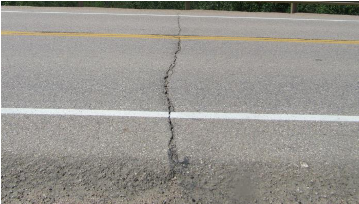
Photo No.6 - Looking west at a 10 to 50 mm wide transverse crack near the northern limit of the site
