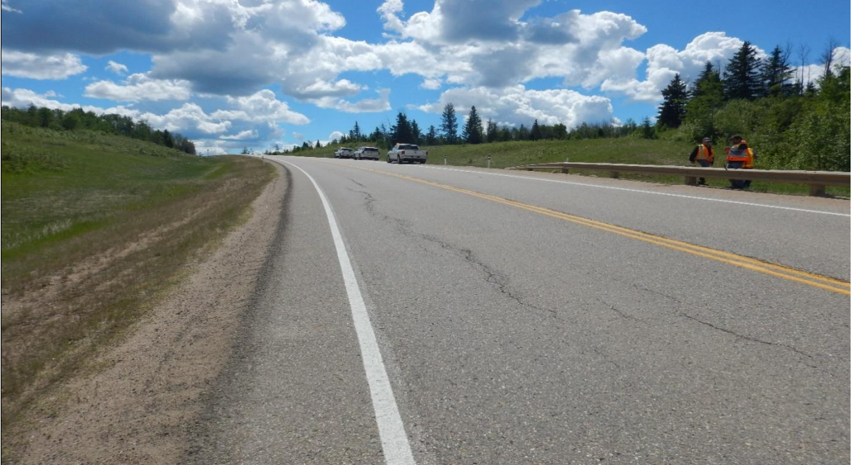
Photo No.1 - Looking south from the southern limit of the site at new longitudinal cracks on the southbound lane
