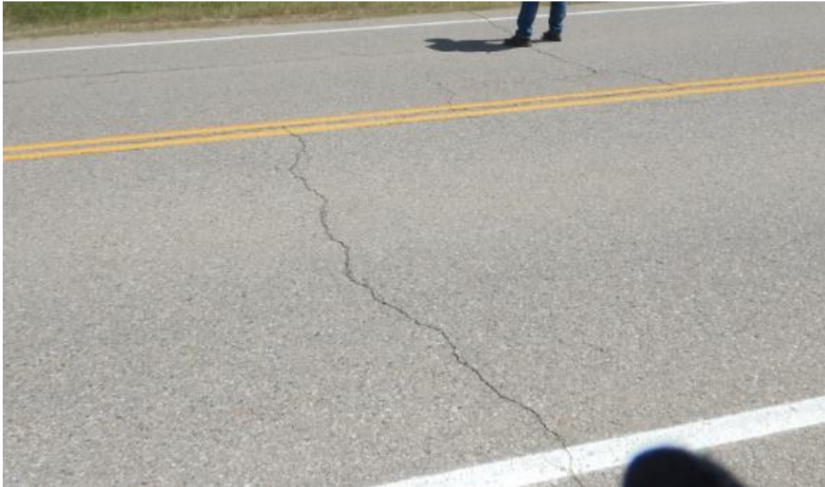
Photo No.7 – Looking east at 10 mm wide transverse crack near the southern limit of the site
