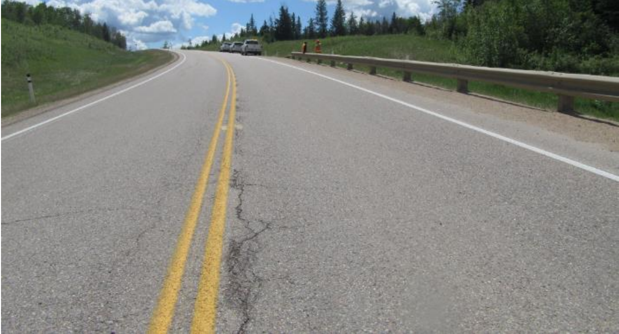
Photo No.5 - Looking south at a 10 to 15 mm wide reflective crack along the highway centerline
