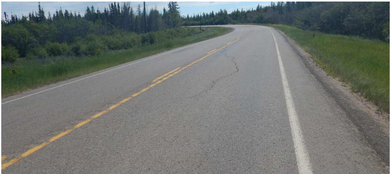
Photo No.2 - Looking east from the western flank of the eastbound landslide (South Slide) at a reflective crack (20 mm wide, no drop) on the east bound lane
