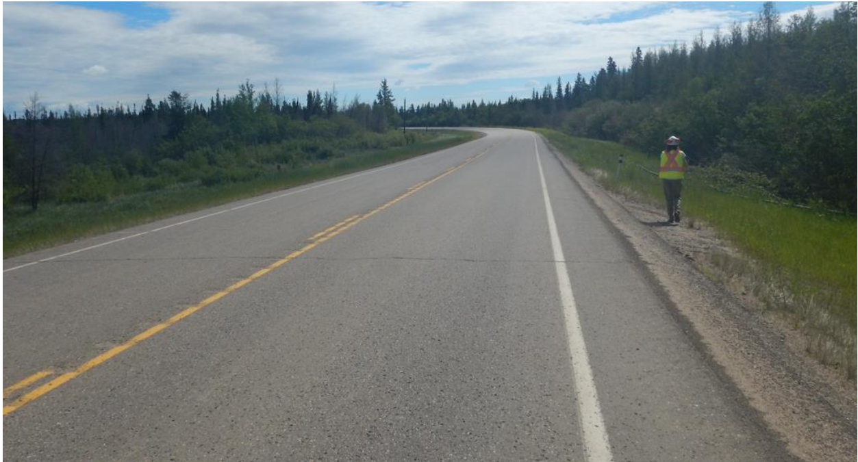
Photo No.1 - General view of the highway lanes at the landslide locations (looking east); the highway was overlaid in July 2018
