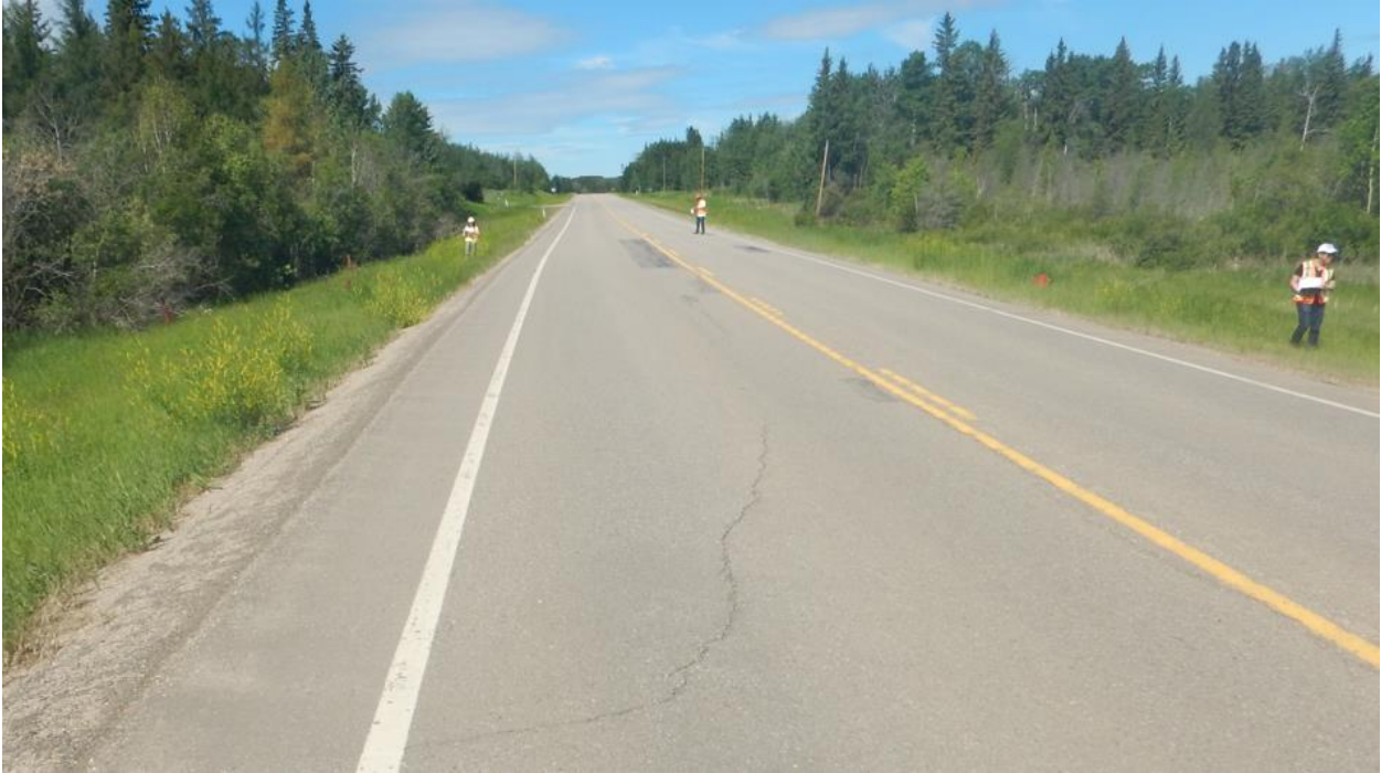
Photo No.3 - Looking west from the eastern flank of the eastbound lane landside at a reflective crack (20 mm wide, 5 mm drop) on the eastbound lane
