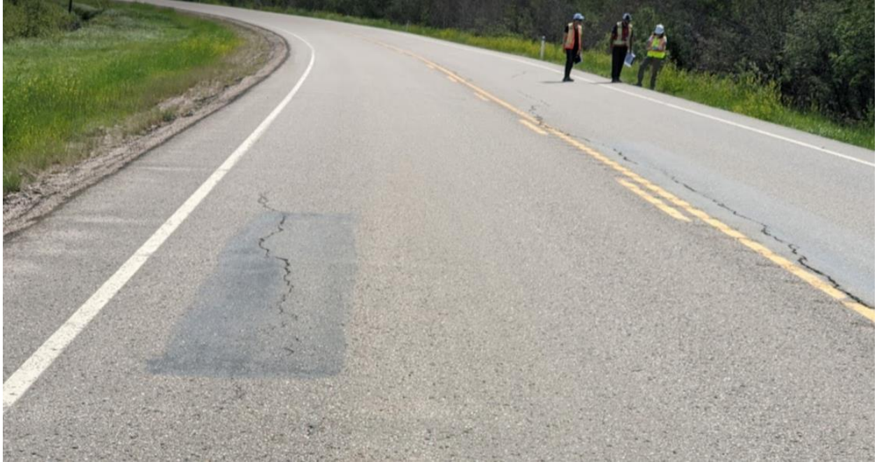
Photo No.5 - Looking east at a reflective crack on the westbound lane (5 to 10 mm wide, no drop)
