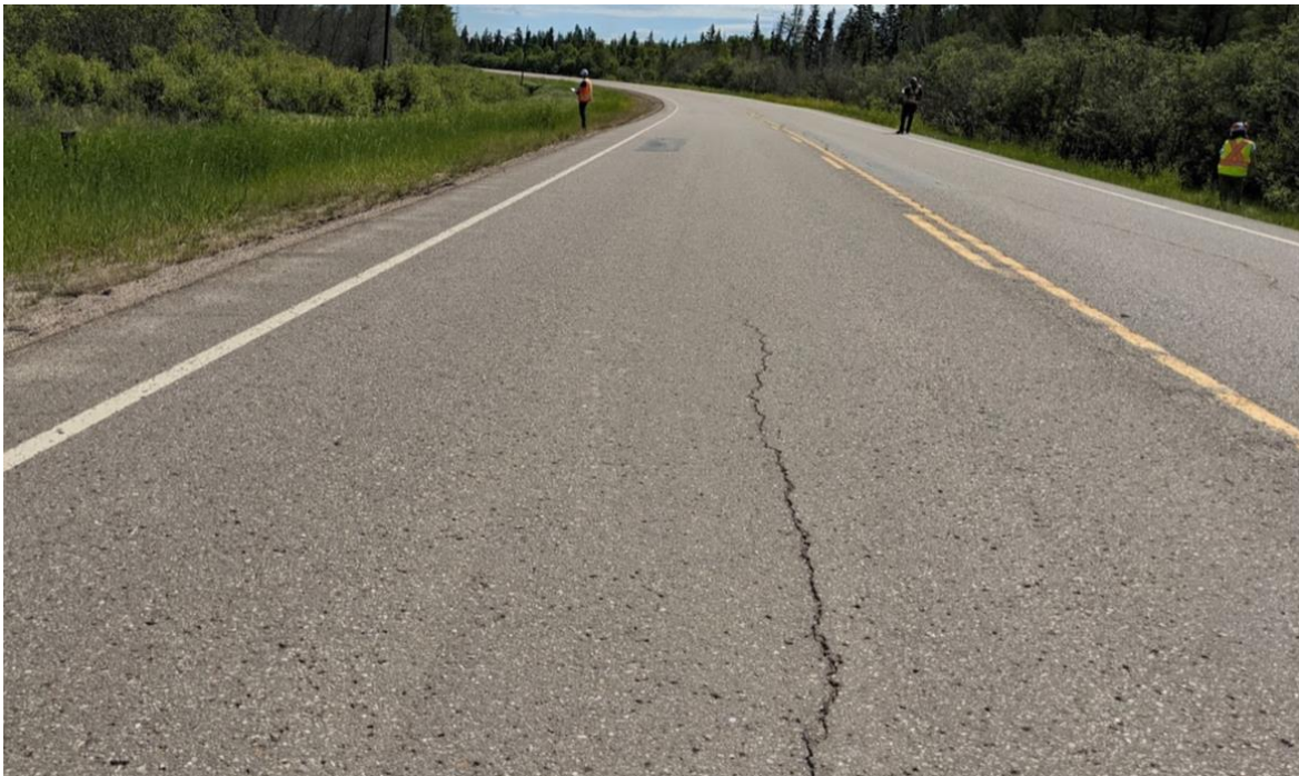
Photo No.4 - Looking east at a reflective crack on the highway westbound lane (10 to 20 mm wide, no drop)
