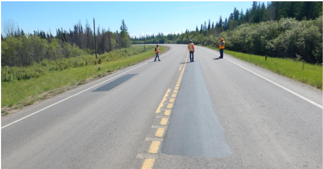
Photo No.2 - Looking east from the western flank of the eastbound landslide (NC58) at the 2019 crack seals
