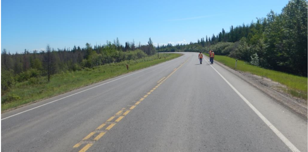
Photo No.1 - General view of the highway lanes at the landslide locations (looking east); the highway was overlaid in July 2018
