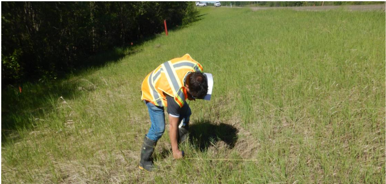
Photo No.4 - Looking at a void formed along the tops of the piles (NC58)
