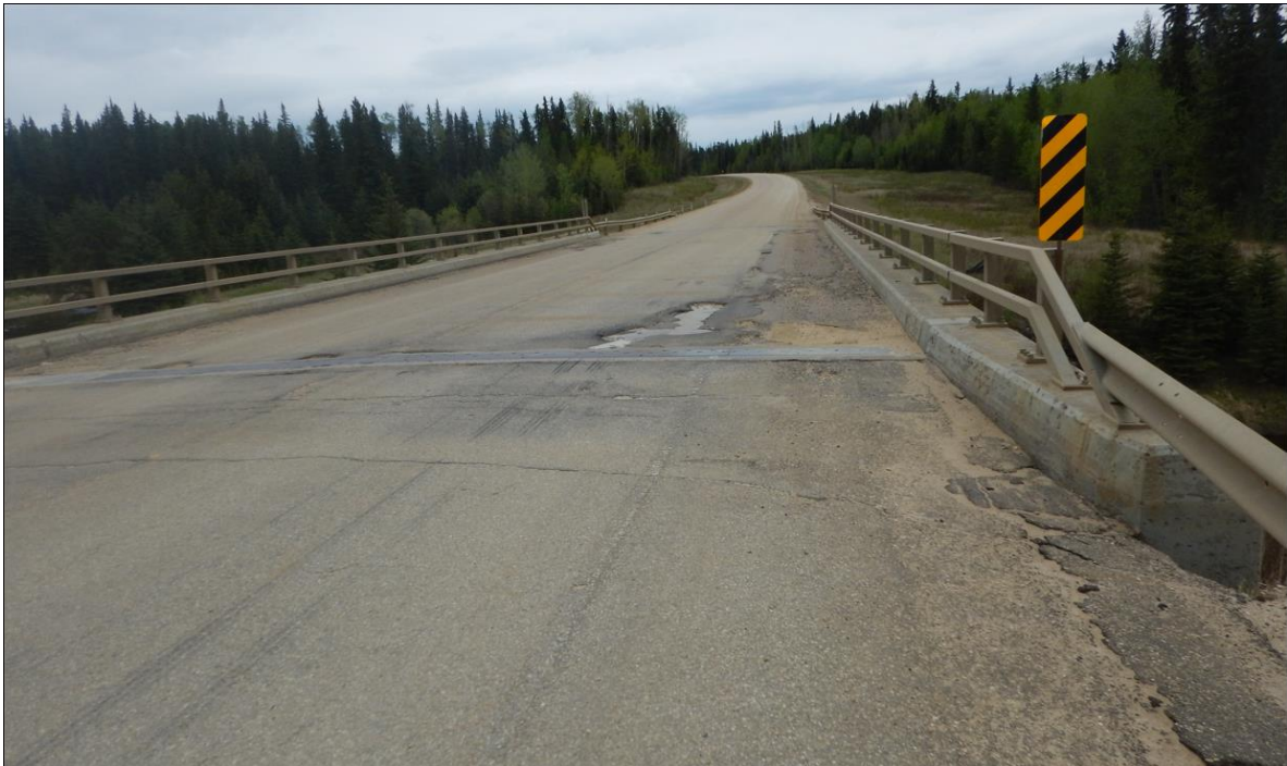
Photo 4. Bridge deck and highway surface condition (Looking north at the south expansion joint).
