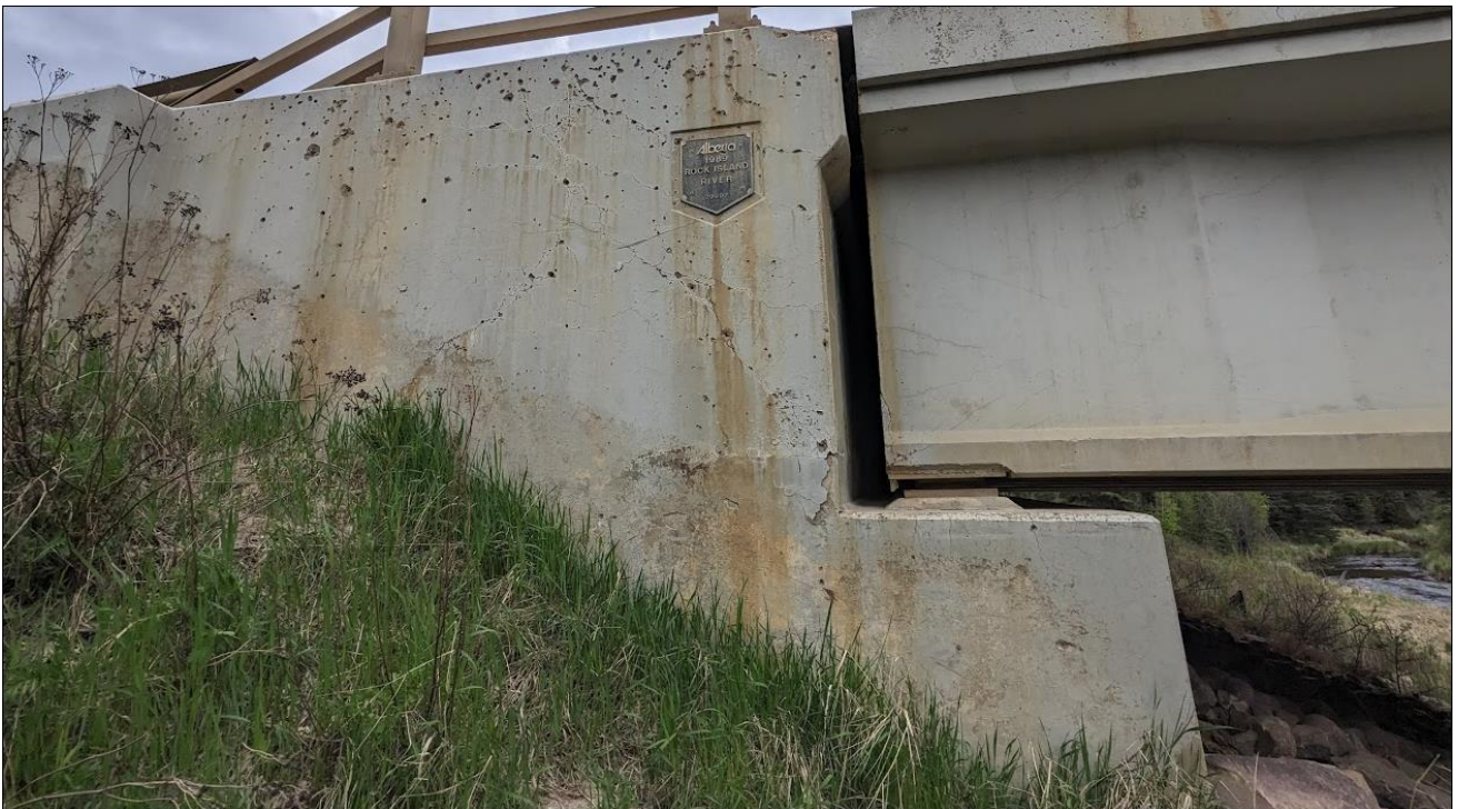
Photo 10. Northwest wingwall: soil staining on the wall face shows original design elevation of fill; approximately 1 m of gravel was placed in 2020 to buttress/cover the gap formed below the wing wall; vegetation has grown within the backfilled area since 2020; erosion up to 500 mm at the top developed within new fill placed against the wing wall. |
