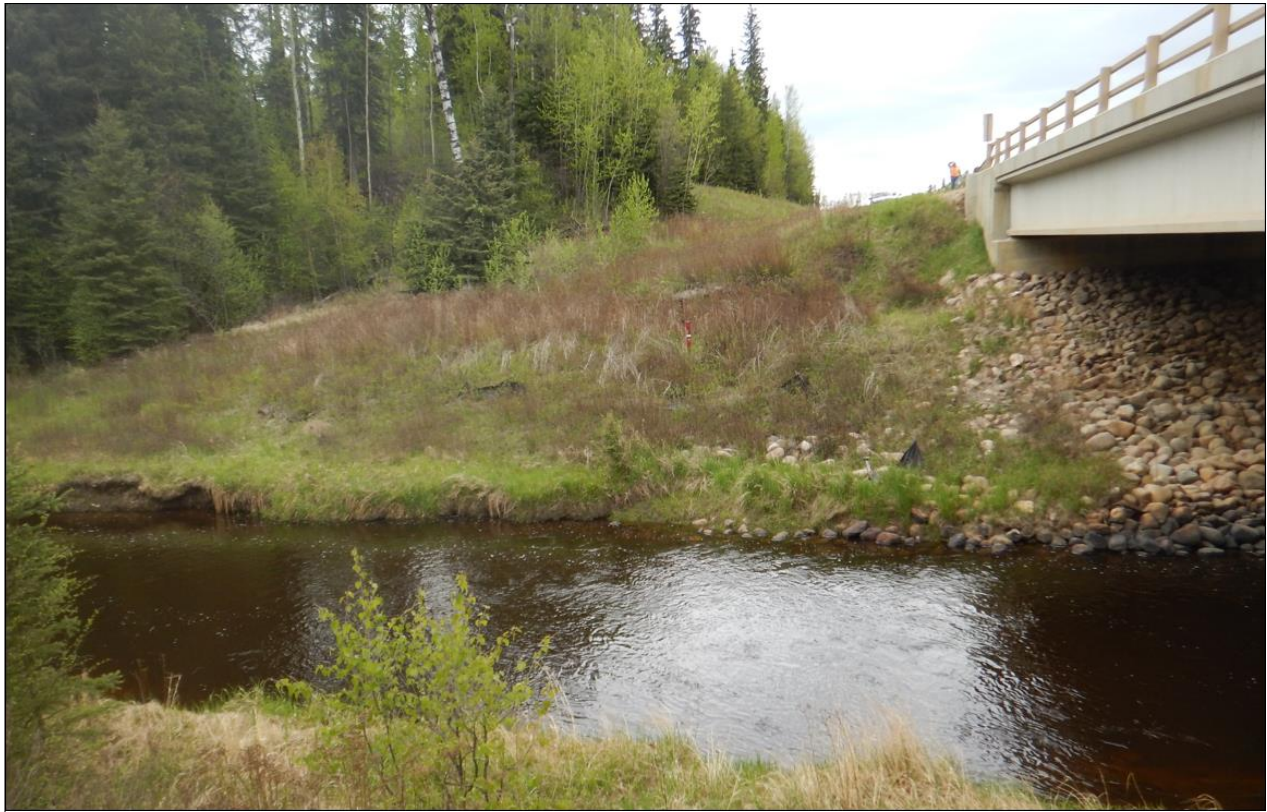
Photo 1. Landslide Area (Looking North).
