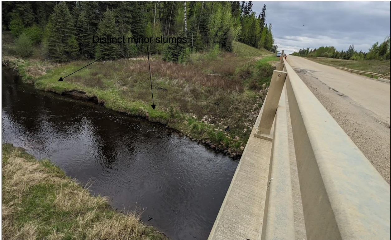
Photo 7. NW approach fill headslope; note two distinct slumps just above the stream level.
