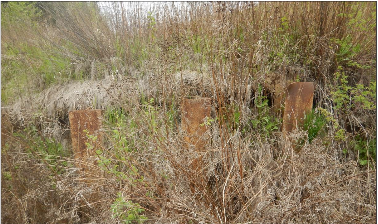
Photo 8. Exposed old bridge H piles within the active landslide mass.
