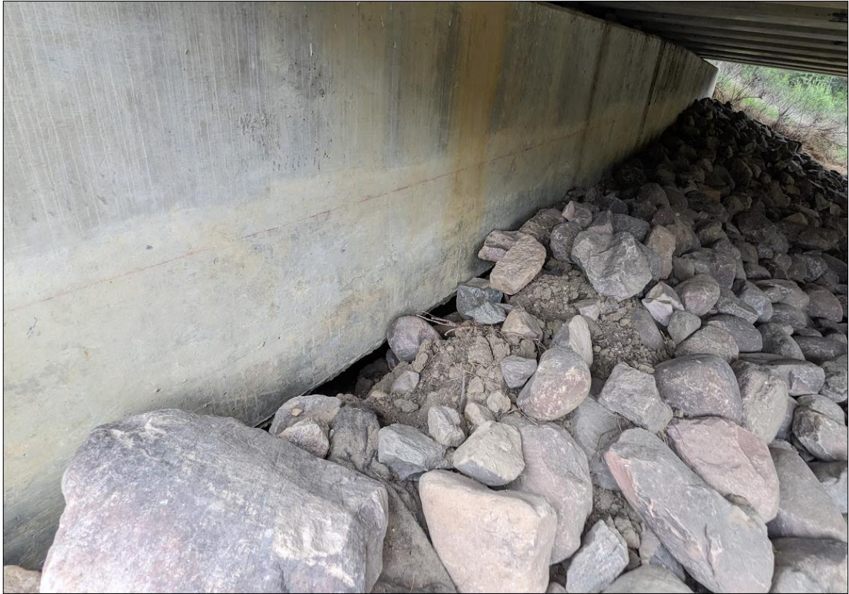
Photo 3. A closer look at the NW corner of the abutment seat. There is a 2.7 m long gap formed along the face of the abutment seat.
