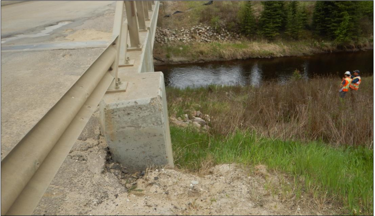
Photo 9. A void forming between the highway side slope and the top edge of the NE wingwall
