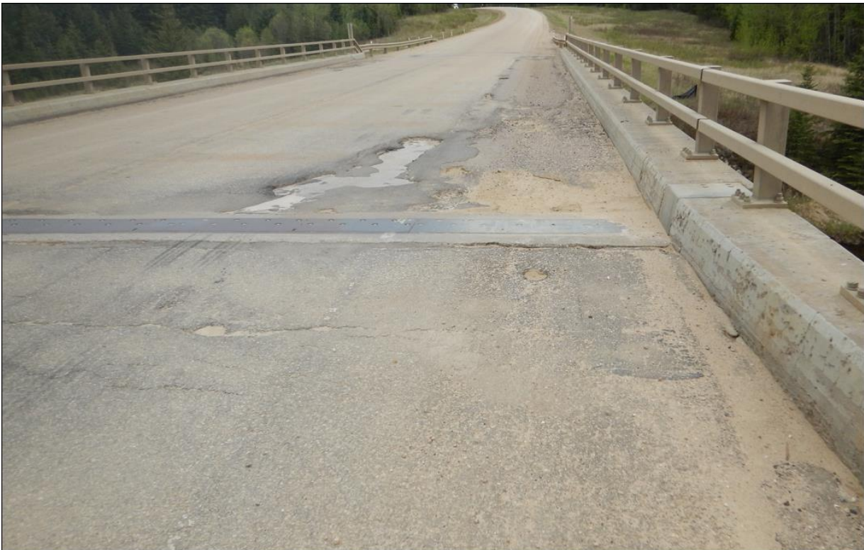
Photo 6. Sealed Cracks along north expansion joint (Looking east). ACP patch placed on the bridge deck in 2022 has failed.
