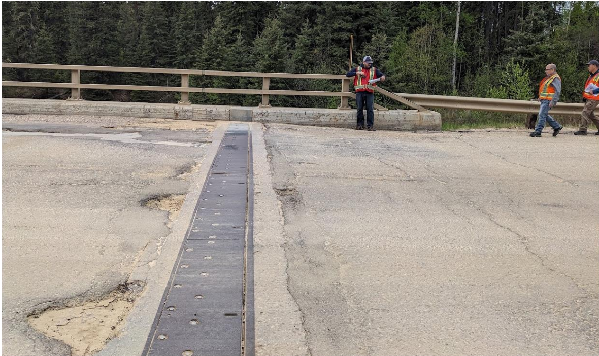
Photo 5. Looking at the north expansion joint. The approach slab dip by the NW wingwall has not changed since 2023.
