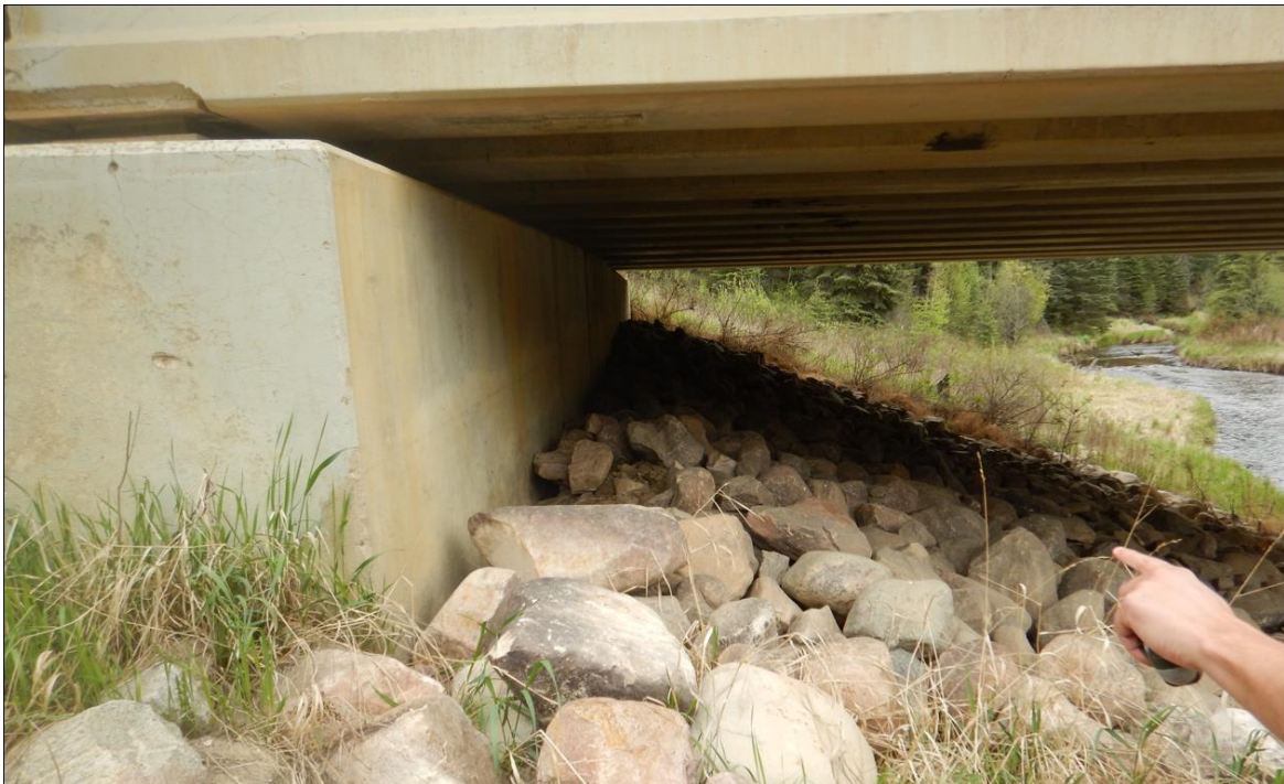
Photo 2. North Abutment (Looking East) showing riprap placed by TEC in 2021; The riprap top surface appears to have dropped for a distance of about 10 m along the face of the abutment seat and the riprap along this zone shifted laterally towards the river.
