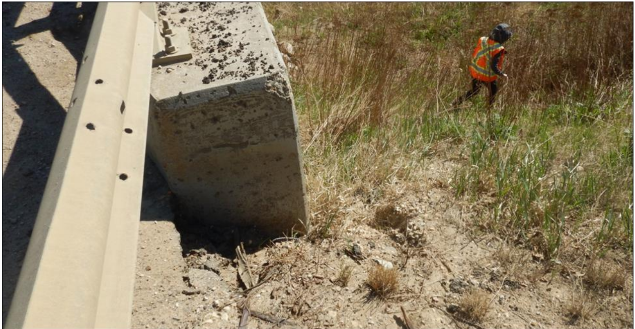
Photo 8. A void forming between the highway side slope and the top edge of the NE wingwall
