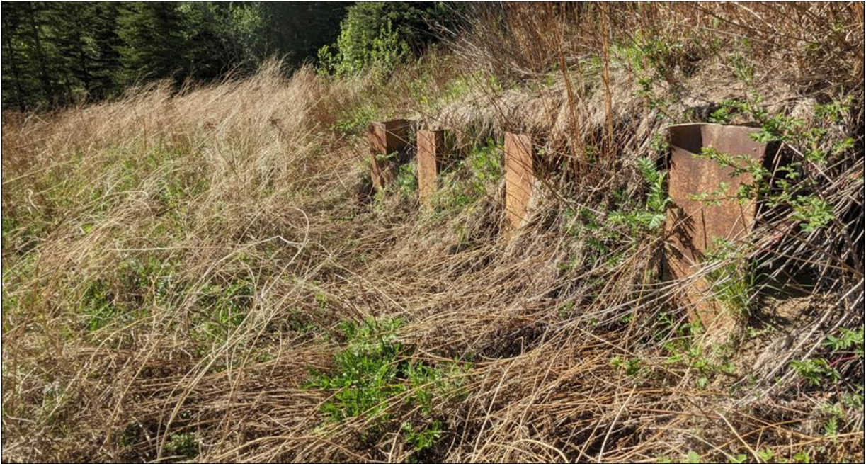
Photo 7. Exposed old bridge H piles within the active landslide mass.
