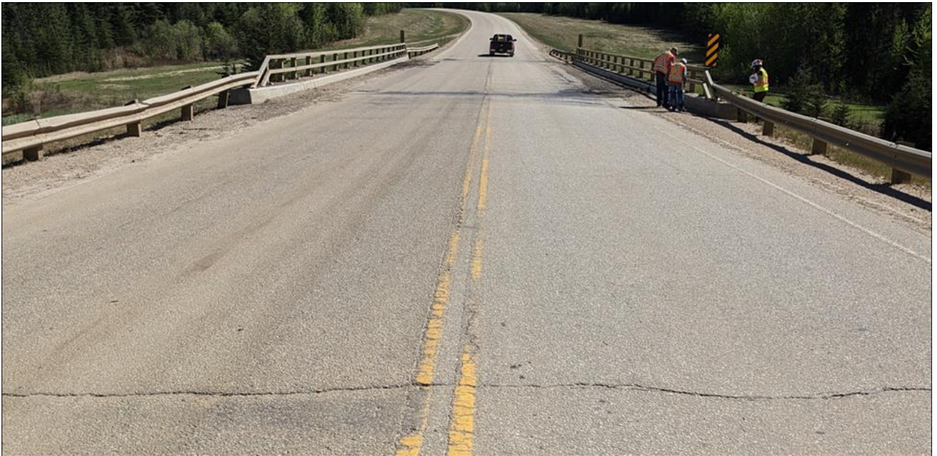
Photo 4. Bridge deck and highway surface condition (Looking south at north expansion joint). The approach slab dip by the NW wingwall was noted to be worse than the dip noted in 2022.
