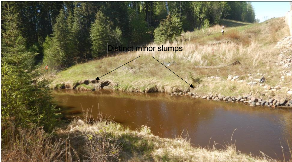
Photo 6. NW approach fill headslope; note two distinct slumps just above the stream level.
