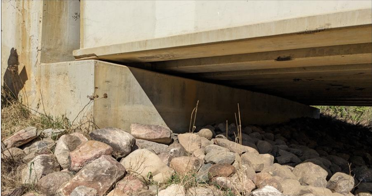
Photo 2. North Abutment (Looking East) showing riprap placed by TEC in 2021; The riprap top surface appears to have dropped for a distance of about 10 m along the face of the abutment seat and the riprap along this zone shifted laterally towards the river.
