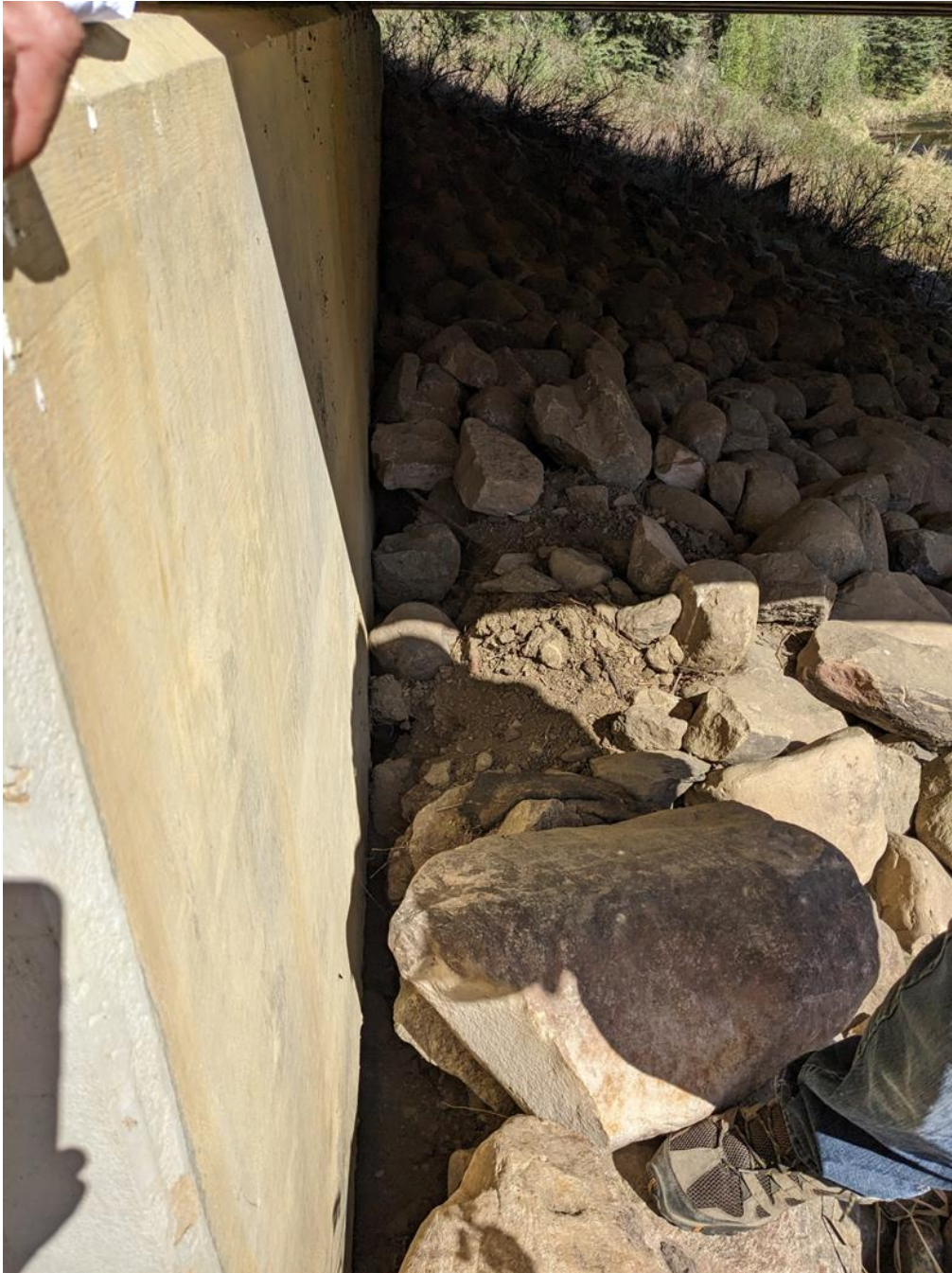
Photo 2A. A Close look at the NW corner of the abutment seat. There is a 2.7 m long gap formed along the face of the abutment seat.
