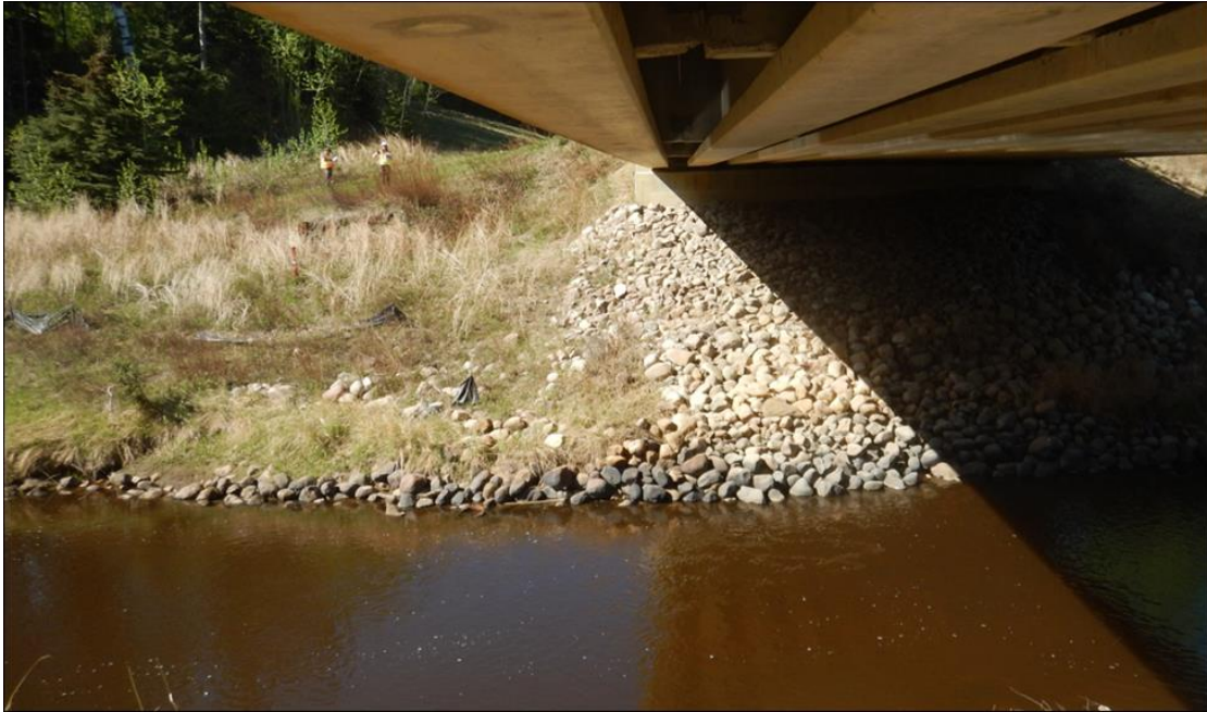
Photo 1. Landslide Area (Looking North).
