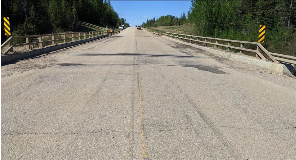
Photo 3. Bridge deck and highway surface condition (Looking north at the south expansion joint). ACP patch placed in 2022 to seal cracks and potholes at the joints and on the bridge deck.
