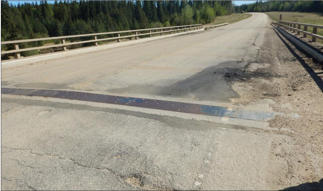
Photo 5. Sealed Cracks along north expansion joint (Looking east). ACP patch placed on the bridge deck in 2022 is failing.
