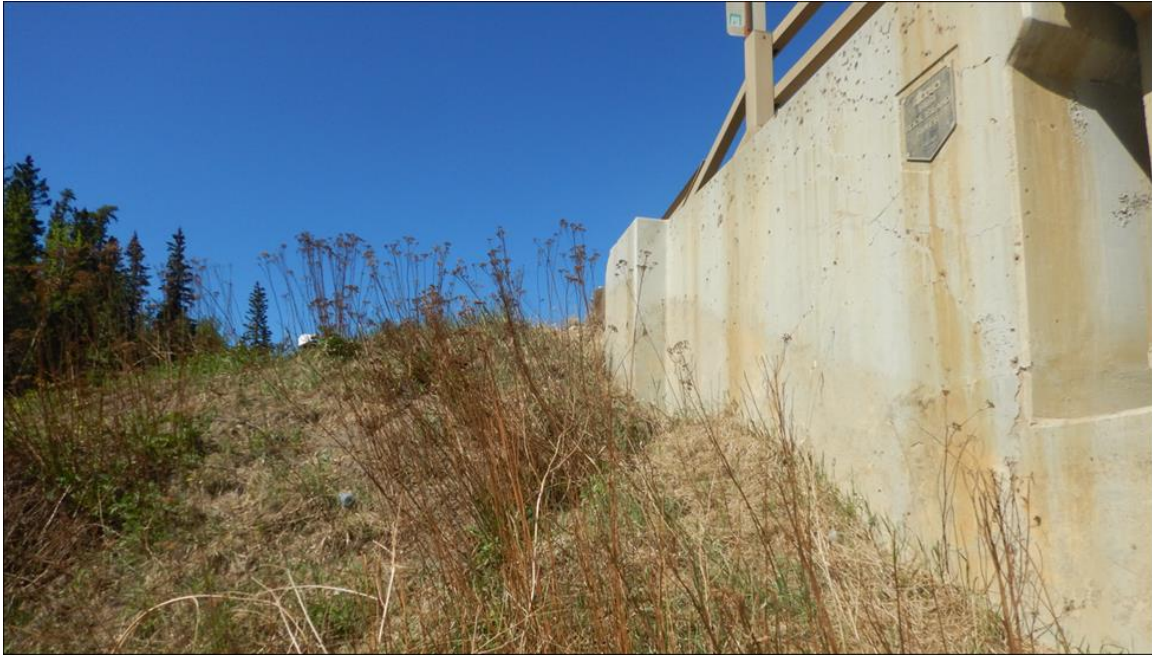
Photo 9. Northwest wingwall: soil staining on the wall face shows original design elevation of fill; approximately 1 m of gravel was placed in 2020 to buttress/cover the gap formed below the wing wall; vegetation has grown within the backfilled area since 2020; erosion up to 500 mm at the top developed within new fill placed against the wing wall. |
