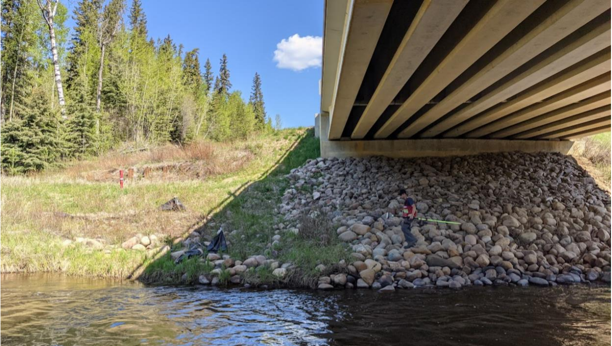
Photo No. 1 – Landslide Area (Looking North)
