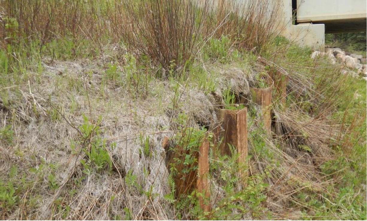
Photo No. 7 – Old bridge H piles showing 1.4 m drop by landslide (Looking East)
