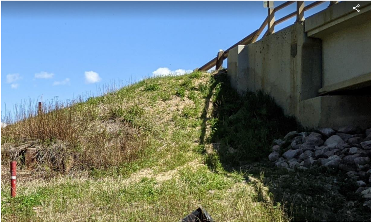
Photo No. 9 –Northwest wingwall: soil staining on the wall face shows original design elevation of fill; approximately 1 m of gravel was placed in 2020 to buttress/cover the gap formed below the wing wall; vegetation has grown within the backfilled area since 2020; slight erosion developed within new fill placed against the wing wall.
