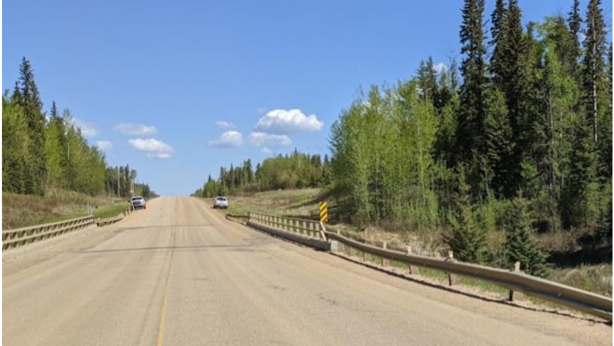
Photo No. 3 – Bridge deck and highway surface condition (Looking north at the south expansion joint).
