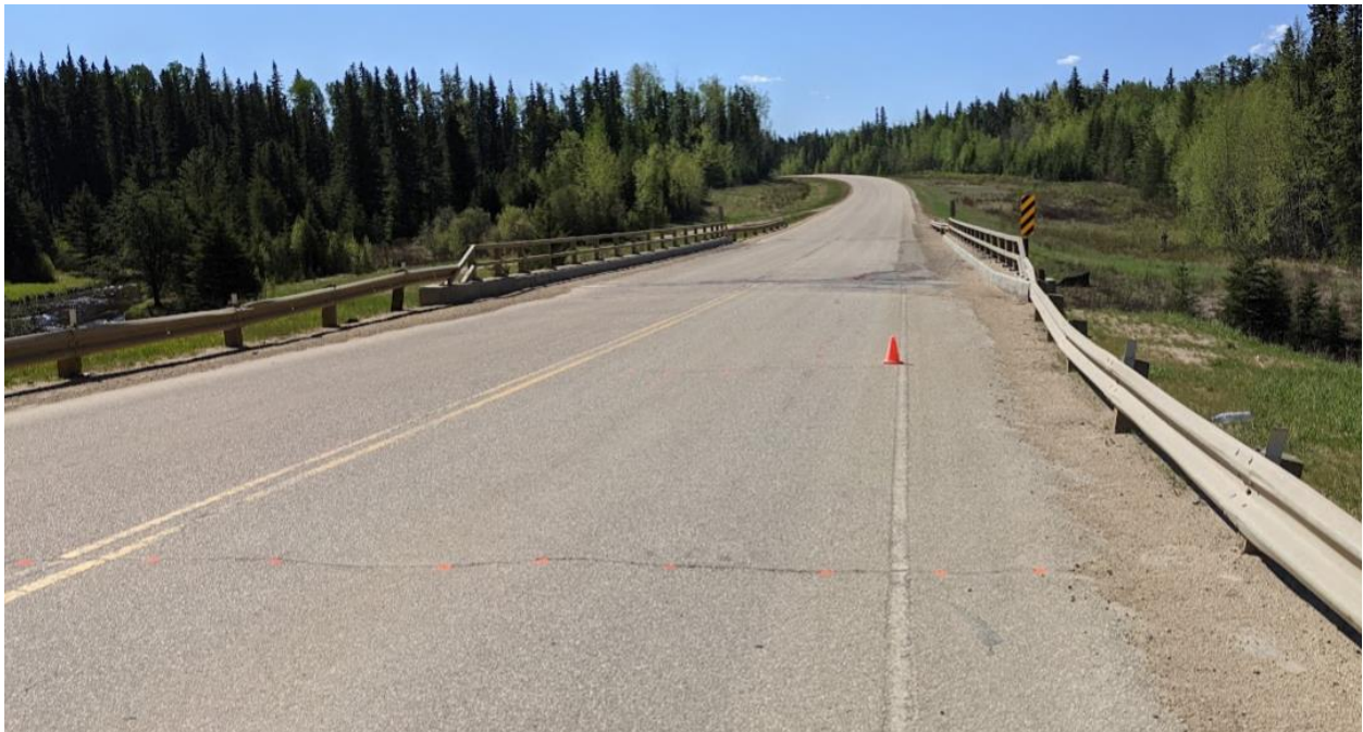
Photo No. 4 – Bridge deck and highway surface condition (Looking south at north expansion joint). Note poor condition of bridge deck wearing surface, and existing dip within the highway SBL by the NW wingwall
