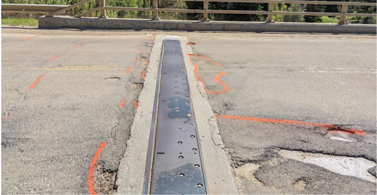
Photo No. 5 – Cracks along north expansion (Looking east)
