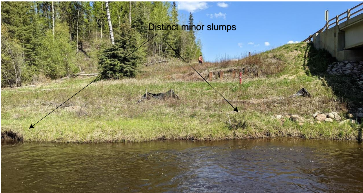
Photo No. 6 – Looking north at the NW approach fill headslope; note two distinct slumps just above the stream
