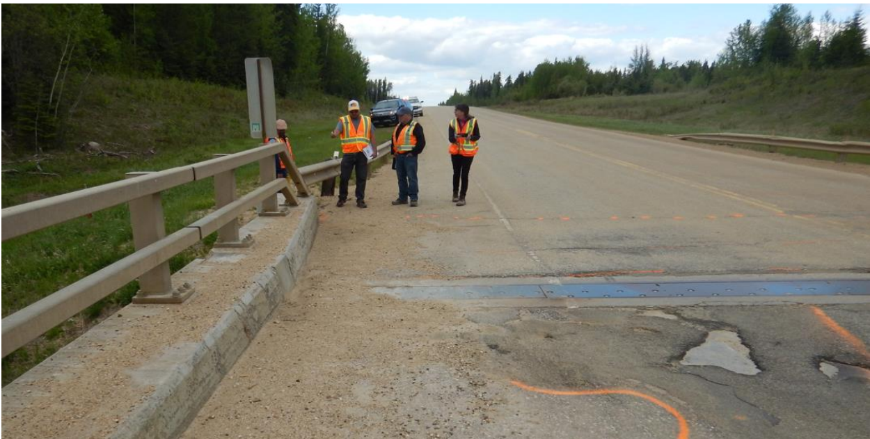
Photo No. 8 –Previous voids, formed behind the wing wall on the highway side and filled with instant patch in 2020 did not open again
