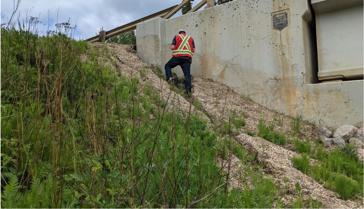
Photo No. 9 – Northwest wingwall. Previous soil staining on the concrete showing up to 1.8 m drop along the design head slopes was backfilled with approximately 1 m of gravel. Gap between bottom of wing wall / abutment seat and ground surface is not visible due to granular fill placed in this area. Note erosion developed on the steeply inclined gravel wedge placed adjacent to the wingwall
