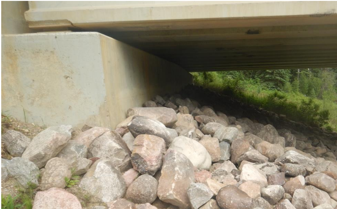
Photo No. 2 – North Abutment (Looking East) showing riprap recently placed by AT
