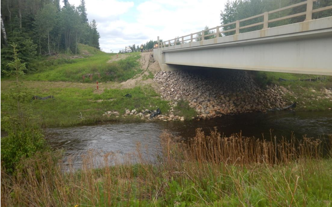
Photo No. 1 – Landslide portion under bridge (Looking North); note new riprap placed under the bridge and gravel wedge adjacent to wingwall covering landslide features
