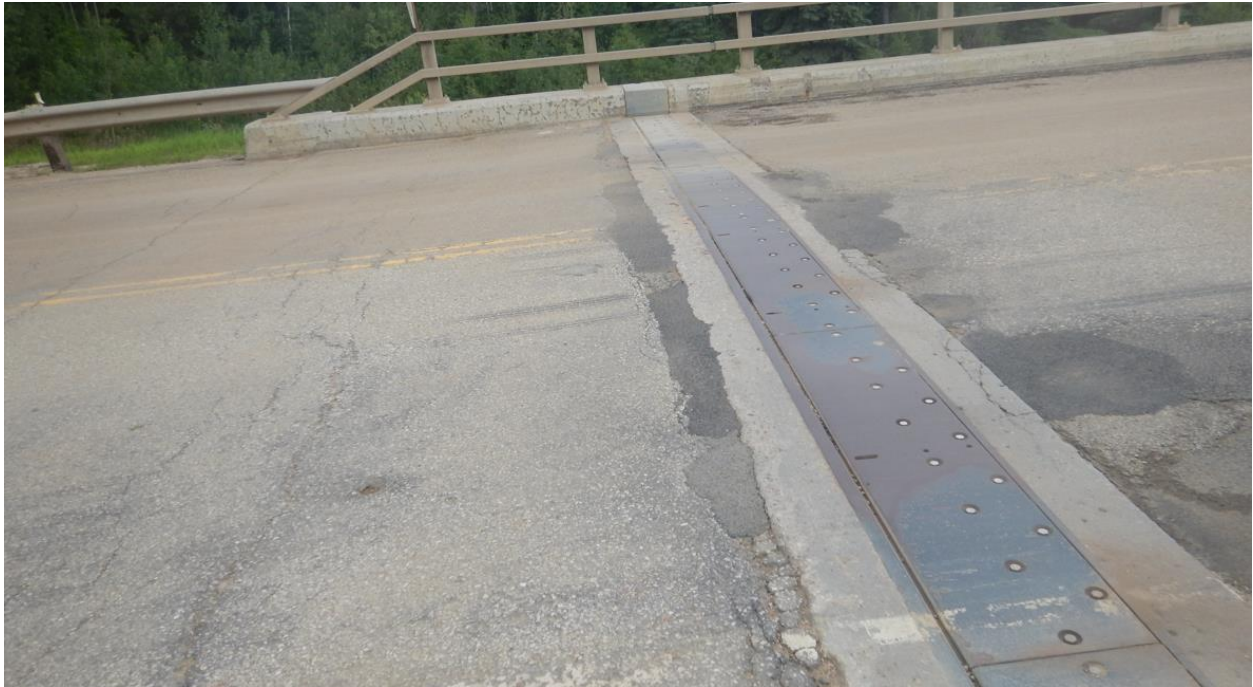
Photo No. 5 – Cracks along north expansion joint filled with instant Patch (Looking east); note cracks within the approach slab
