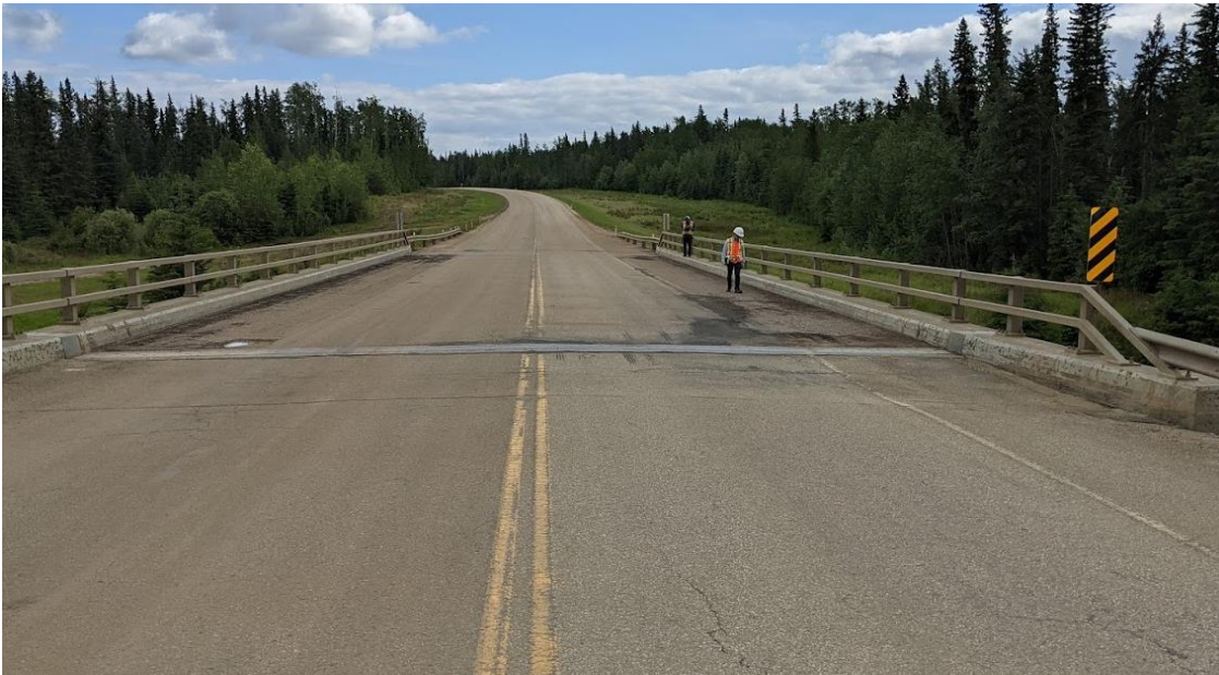
Photo No. 4 – Bridge deck and highway surface condition (Looking south at north expansion joint). Note water ponding on the northeast and northwest corners of the bridge deck, poor condition of bridge deck wearing surface, and existing dip within the highway SBL by the NW wingwall
