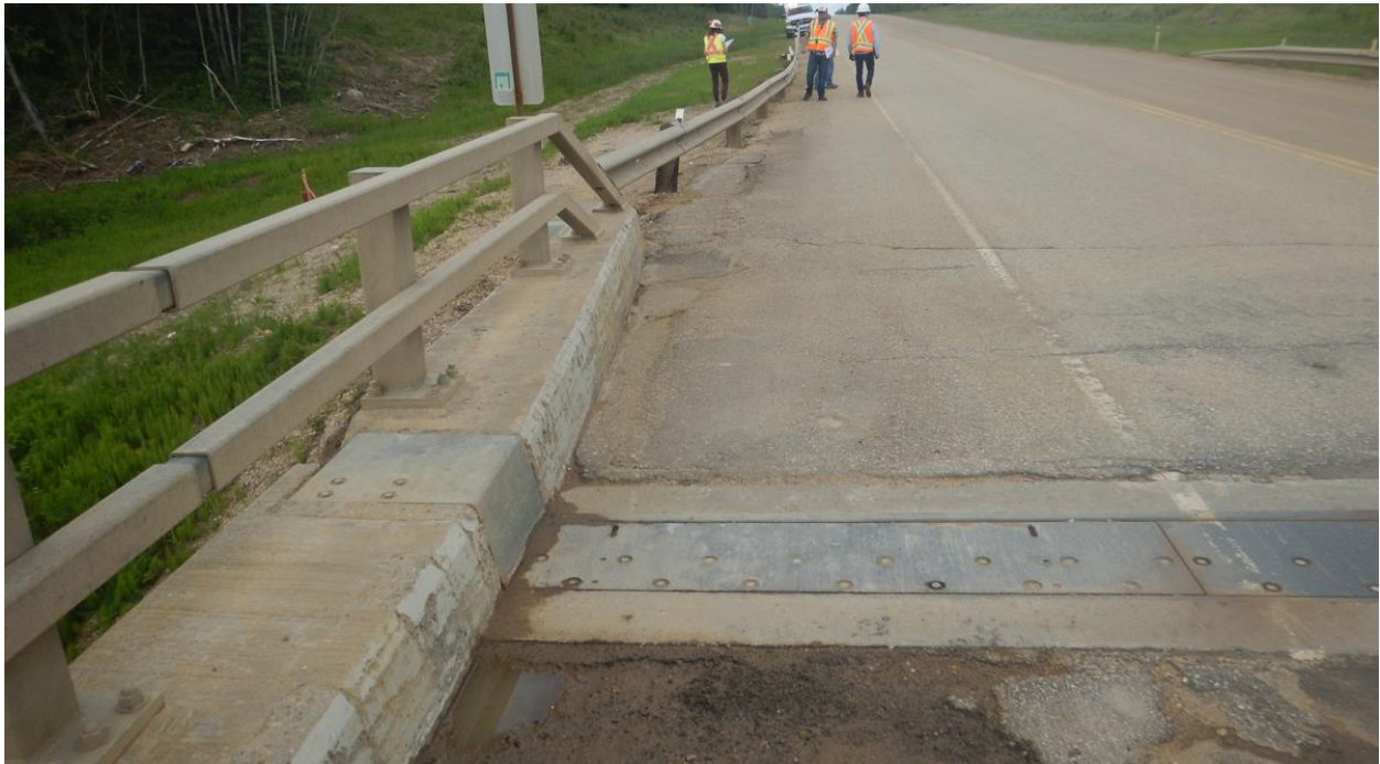
Photo No. 8 – Voids, noted in 2020, between the concrete curb and the asphalt above the NW wing wall (80 to 100 mm wide, 2.3 m long, > 3.5 m deep) filled with instant patch
