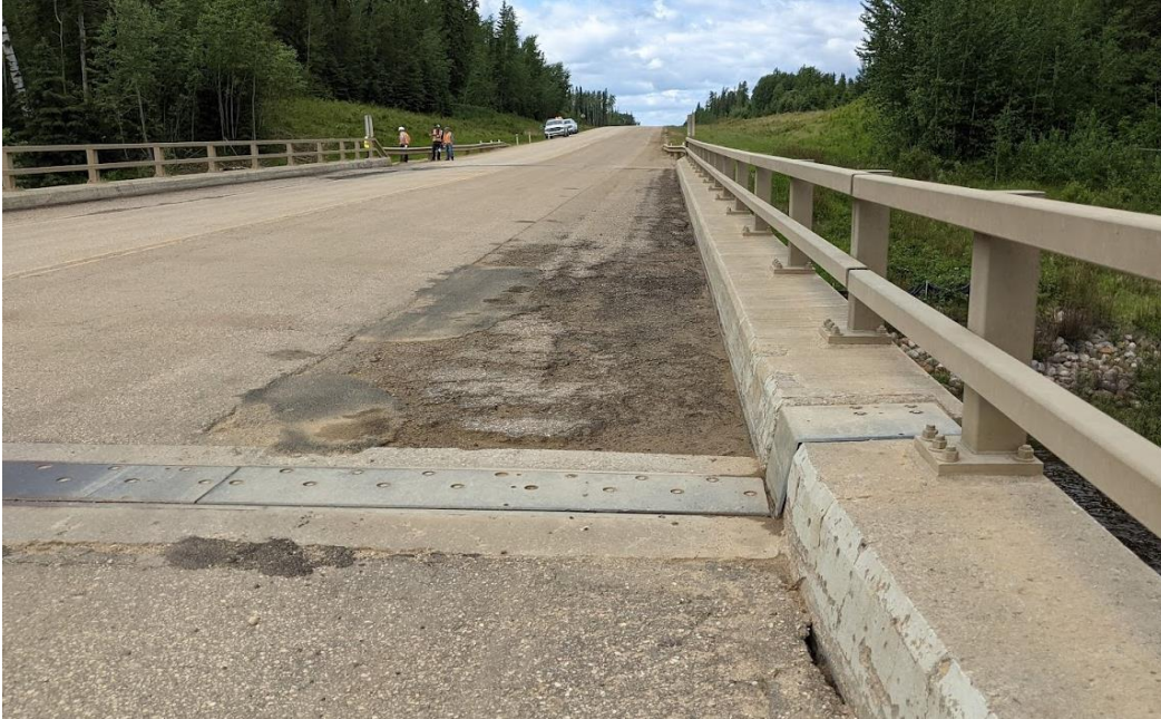
Photo No. 3 – Bridge deck and highway surface condition (Looking north at the south expansion joint). Note 50 mm gap between the pavement and wing wall
