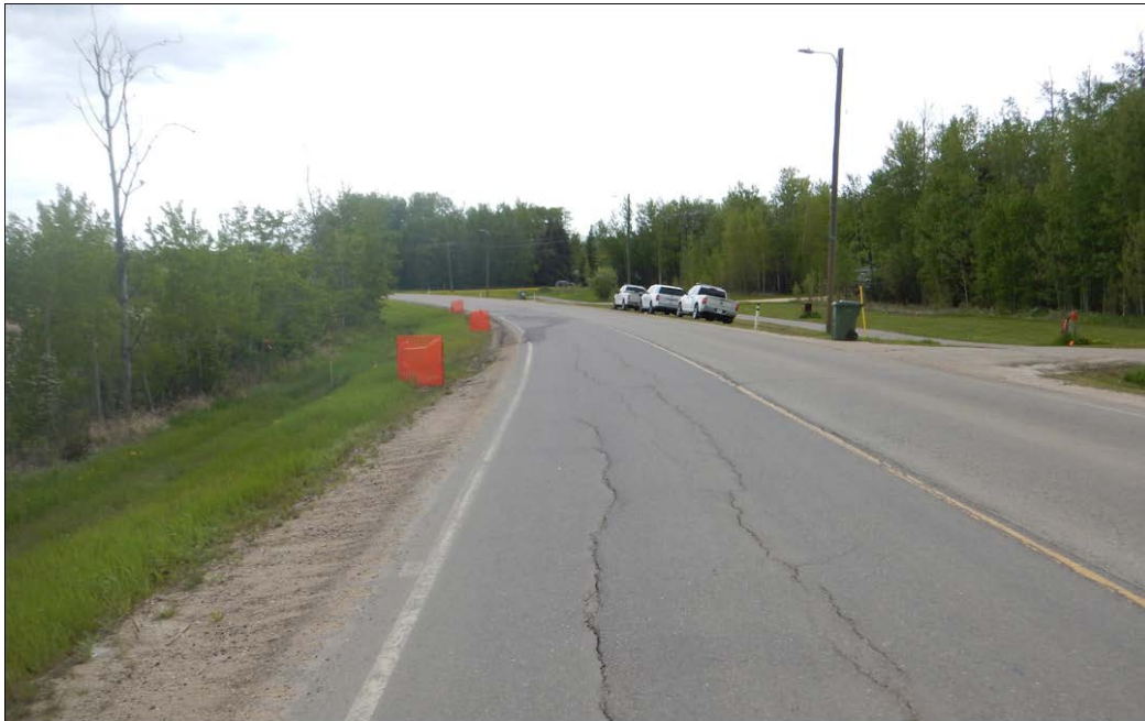
Photo 3. Longitudinal cracks (15-20 mm wide, 20 mm drop) within the previously patched area. There is a 50 mm dip with a twist on the southern portion of the site.
