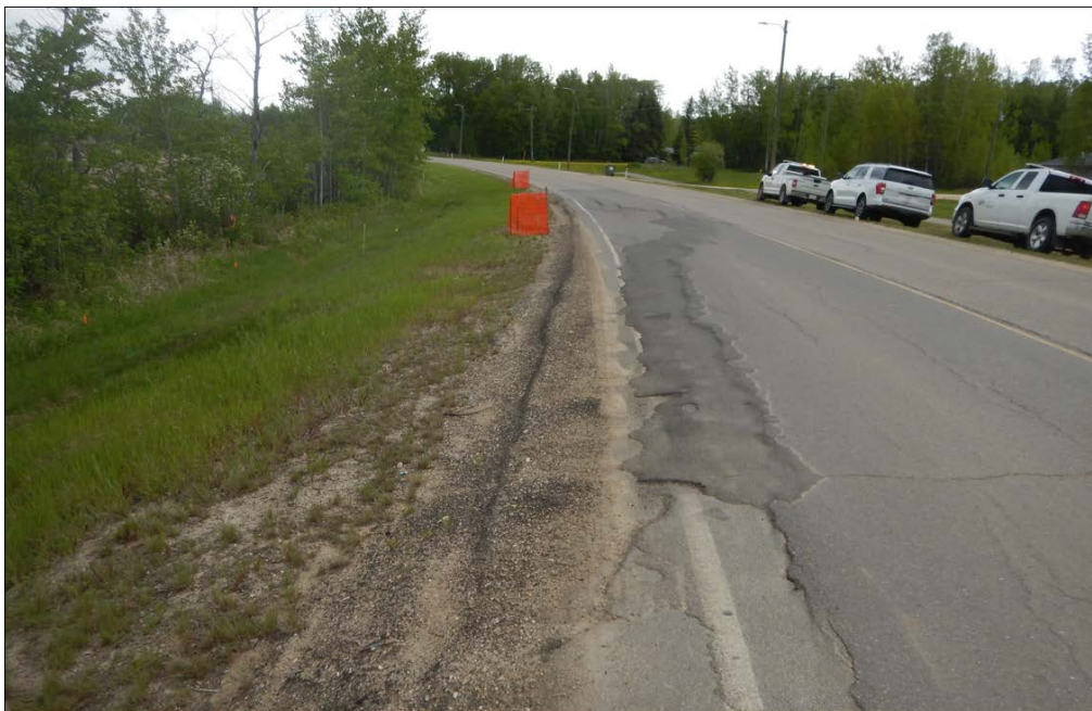
Photo 5 B. (2024) – Headscarp Crack 50 m long, 300 mm wide, 300 mm drop
