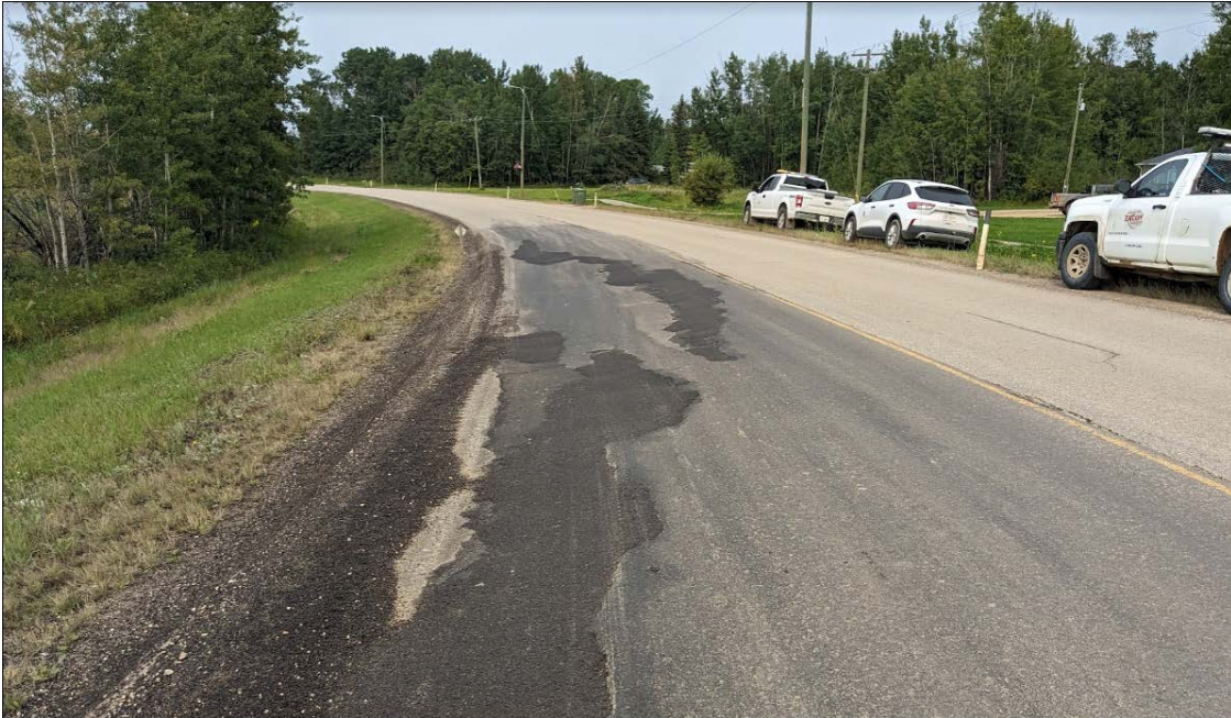
Photo 5 A. (2023) – Headscarp Crack 45 m long, 300 mm wide with 200 mm drop
