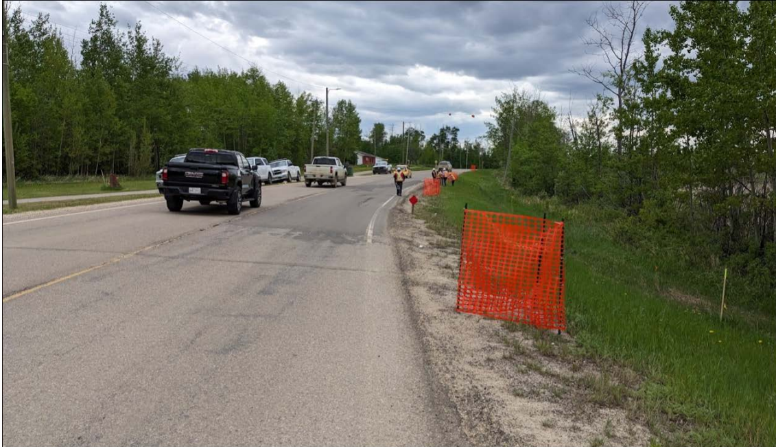
Photo 1. Northern flank of landslide. Head scarp open cracks were filled with ACP in early Spring 2024. Note the significant dip on the highway surface (approximately 300 mm drop).
