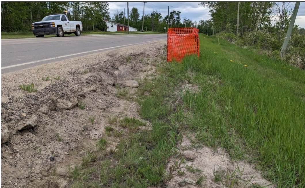
Photo 4. Southern flank of the landslide (looking south); 1.2 m wide x 0.2 m deep landslide crack on the highway west side slope.
