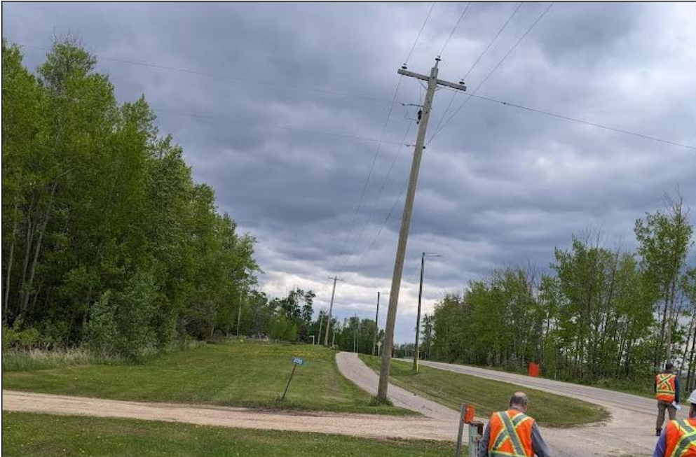
Photo 6. Looking south from the east side of the highway at Power Pole No. 2, which appeared to have tilted more between 2023 and 2024
