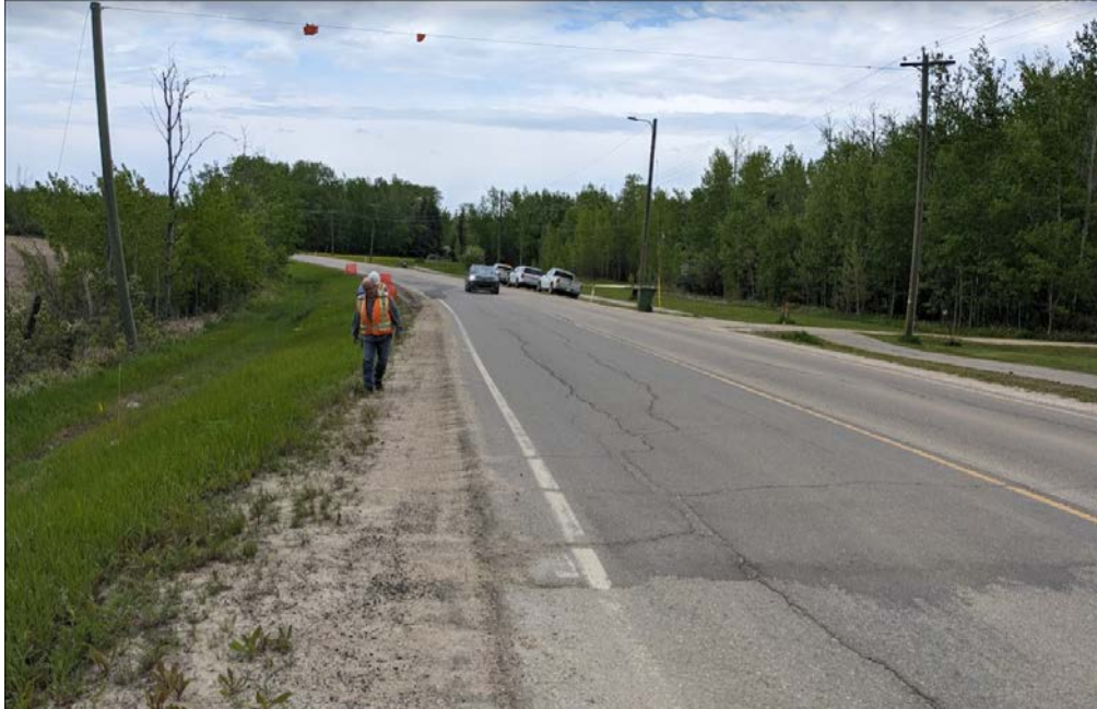
Photo 2. Looking north at the landslide area. Anchor Power Pole No. 3 on the LHS and the Power Pole No. 2 on the RHS of the photo are bent due to the high tension in the overhead cable.
