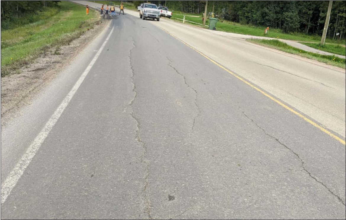
Photo 3. Longitudinal cracks (30 mm wide by 30 mm deep) within the previously patched area. There is a 50 mm dip with a twist on the southern portion of the site.
