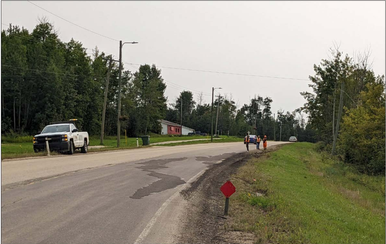
Photo 1. Northern flank of landslide. Head scarp crack was patched a few days before August 24, 2023 site visit. Note the sharp drop off on the highway shoulder (approximately 300 mm drop).
