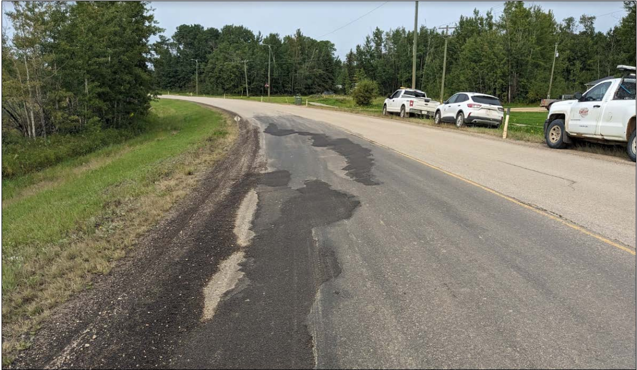
Photo 5. Looking north at the severely impacted section of the highway by the landslide movement. Head scarp crack at this section (near the northern flank of the landslide) is 300 mm wide with up to 200 mm drop.
