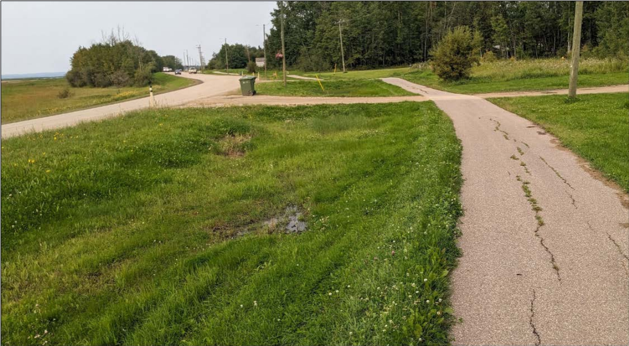
Photo 7. Minor water ponding on the east side of the highway
