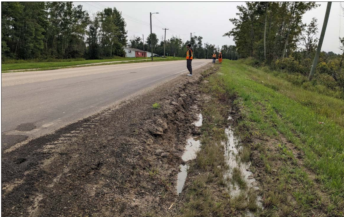
Photo 4. Southern flank of the landslide (looking south); 1.2 m wide x 0.2 m deep landslide crack on the highway west side slope.
