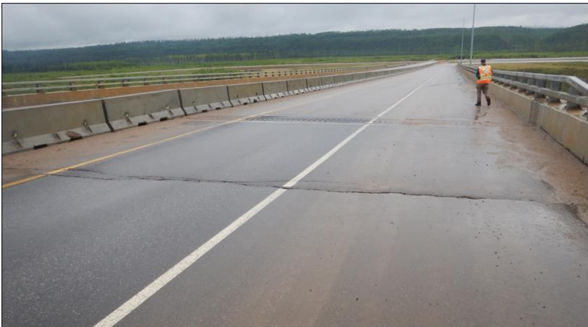
Photo No. 2 – Looking east at east bound lane. Cracks up to 60 mm wide and 90 mm deep
