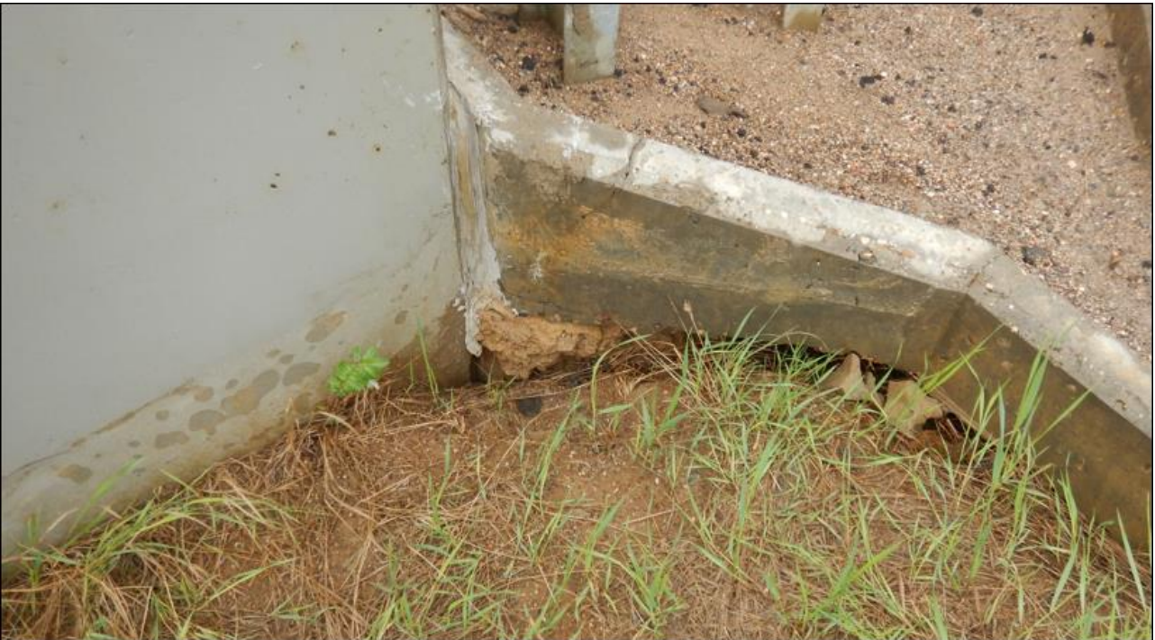
Photo No. 4 – A Flexible filler placed in 2024 to seal the 50 mm wide separation gap between the northwest wing wall and the drain trough. However, up to 300 mm deep gap was noted below the drain trough in response to fill settlement
