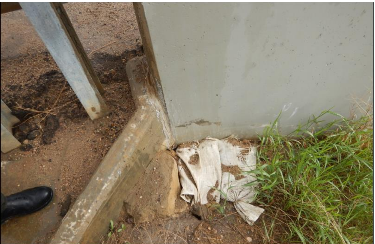
Photo 7 – South drain trough. The gap between the drain trough and wingwall was sealed with a flexible filler.
