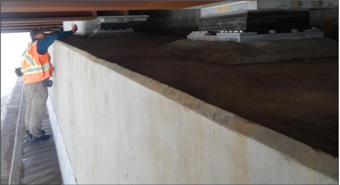
Photo No. 6 – Bridge bearings appear to have maxed out.
