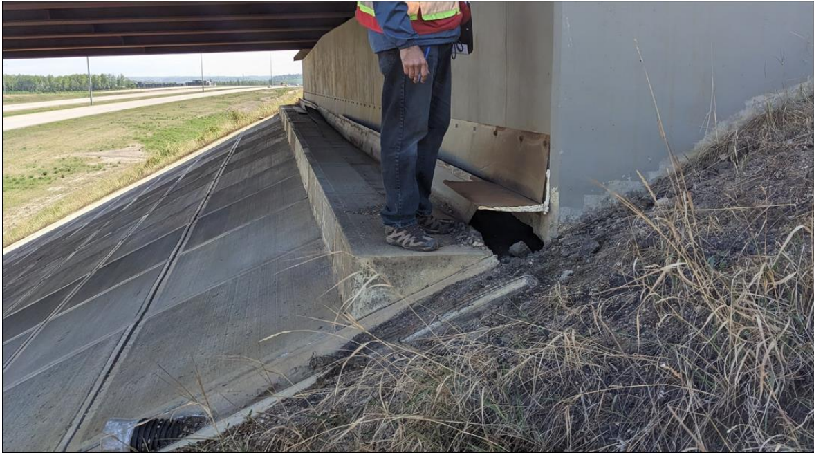
Photo No. 5a – (Taken in Spring of 2023) Looking south at head slope movement (300 mm vertical drop x 300 mm lateral shift towards east); Void under abutment seat ranges from 0.8 m to 2.7 m.
