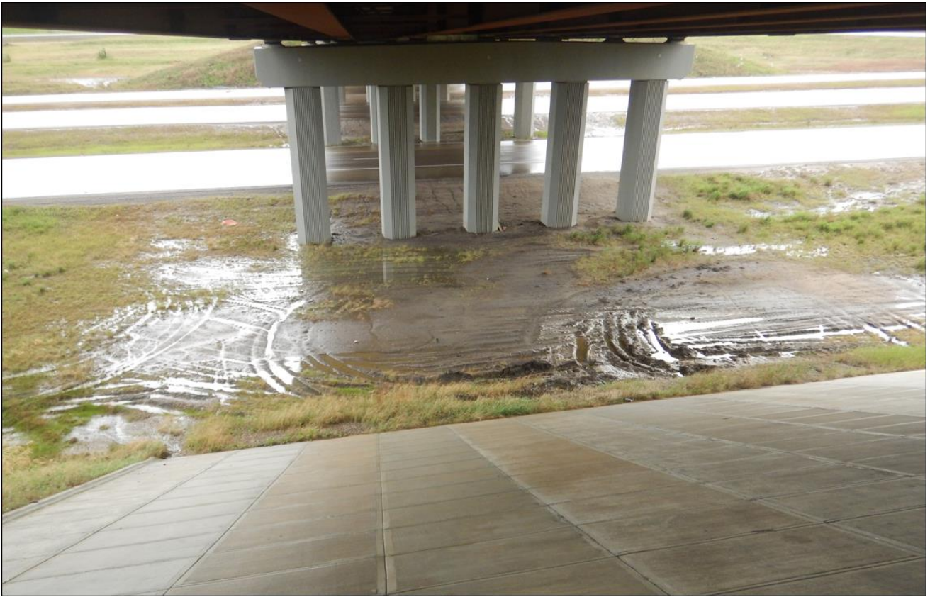
Photo 8 – Water ponding and rutting at the toe of the bridge west headslope
