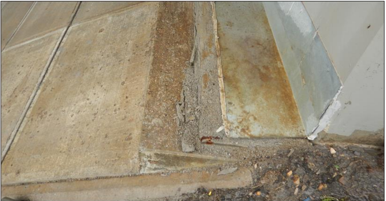
Photo No. 5b – (Taken in Spring of 2024) Void under the abutment seat shown in photo 5a was filled with grout; However, ground appears to have dropped by 20 mm and displaced laterally by 10 mm at this location
