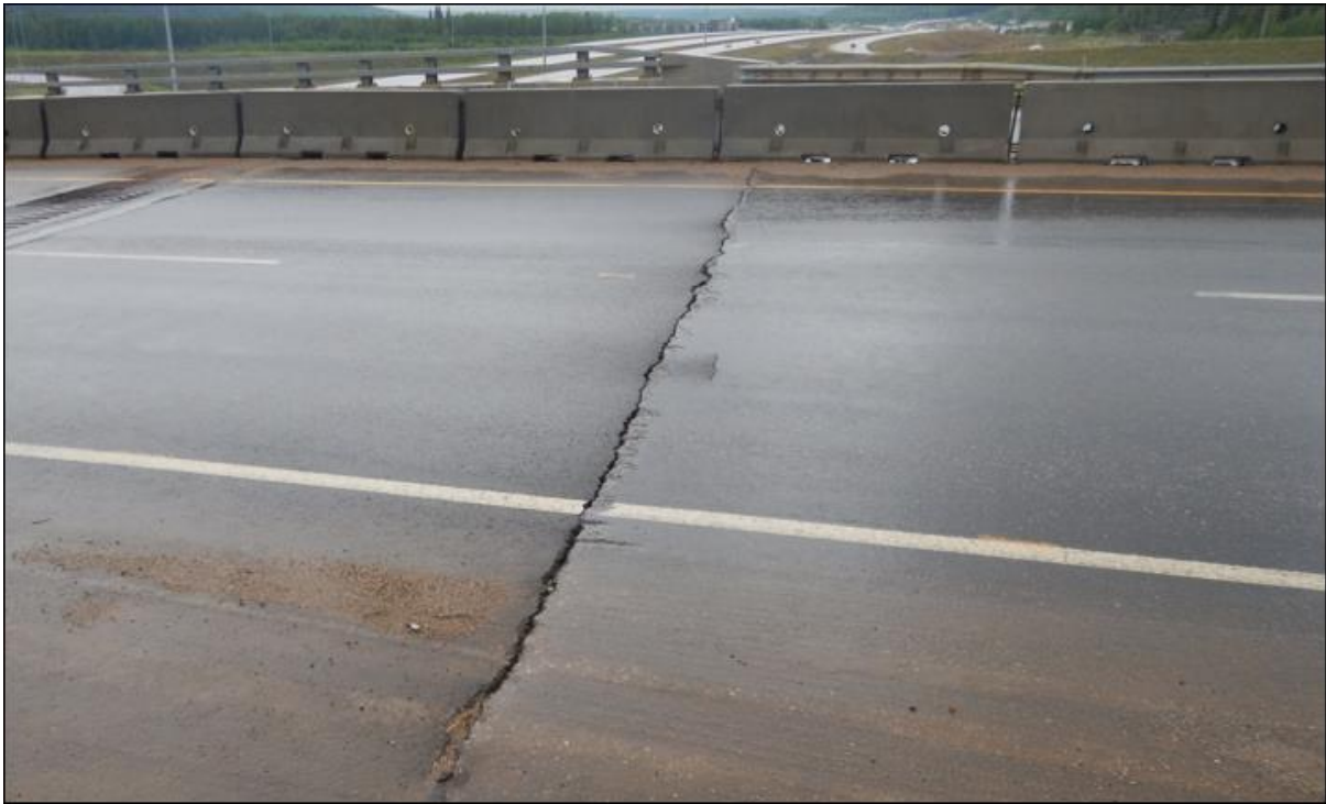
Photo No. 1 – Looking south at the crack developed across the westbound lanes towards the median. The main crack is 20 to 40 mm wide x 10 to 40 mm deep. The cracks are across both traffic lane directions and have formed between the approach slab and the pavement, about 6 m west of the west abutment fingerplate; a new ACP patch was noted in 2024.
