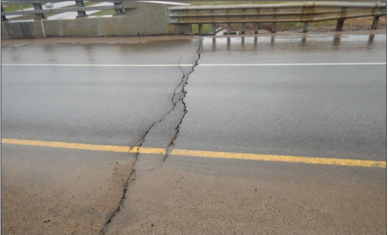
Photo No. 3 – Looking south at east bound lane. Cracks up to 60 mm wide and 90 mm deep
