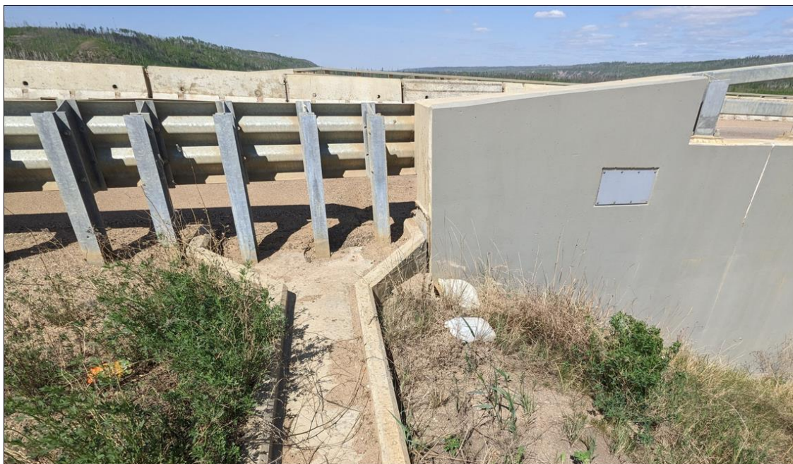
Photo 6 – Drain trough. Note the cracking between the drain trough and wingwall.
