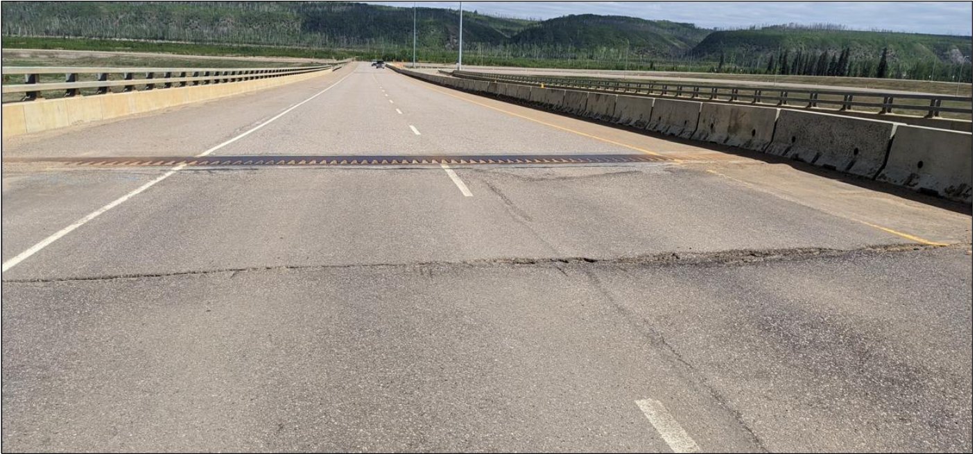
Photo No. 1 – Looking east at the bridge westbound lanes. The cracks are across both traffic lane directions and has formed between the approach slab and the pavement, about 6 m west of the west abutment fingerplate; note ACP patch placed in 2022 and the dip to the west of the expansion joint.
