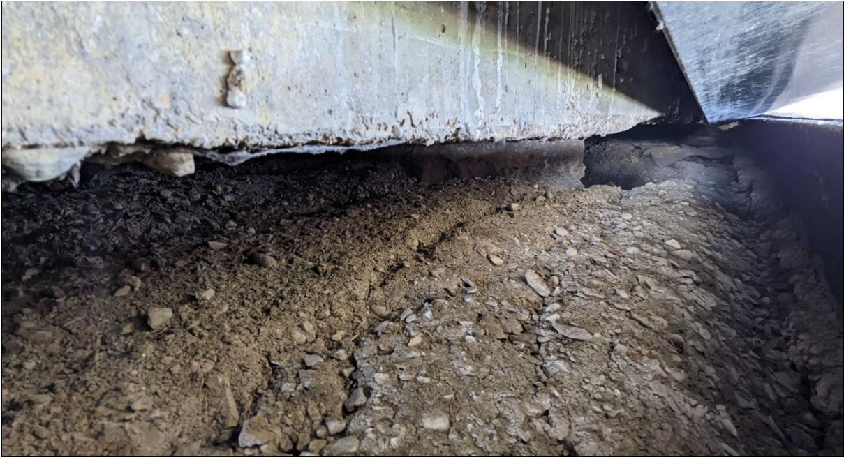
Photo No. 3 – Void under abutment seat. Head slope dropped by up to 300 mm and moved eastward by up to 300 mm
