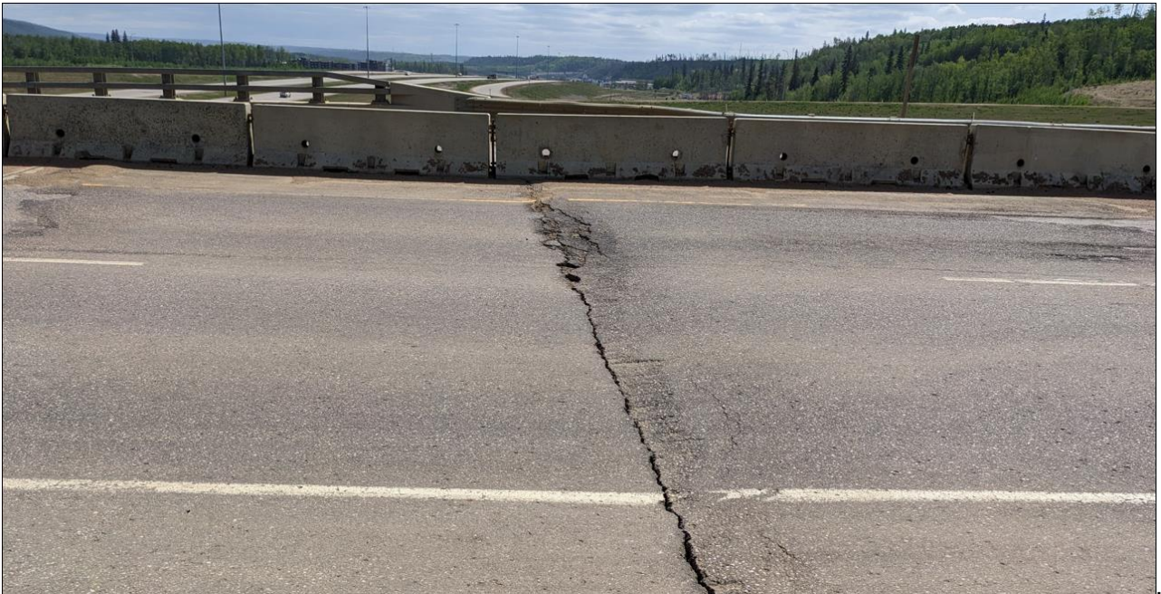
Photo No. 2 – Looking south at the crack developed across the westbound lanes towards the median. The main crack is 30 to 100 mm wide x 70 to 100 mm deep.
