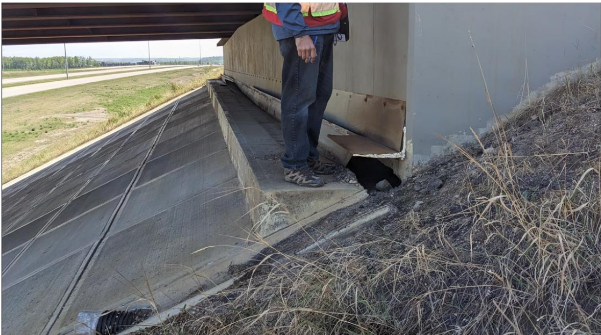
Photo No. 4 – Looking south at head slope movement (300 mm vertical drop x 300 mm lateral shift towards east); Void under abutment seat ranges from 0.8 m to 2.7 m.
