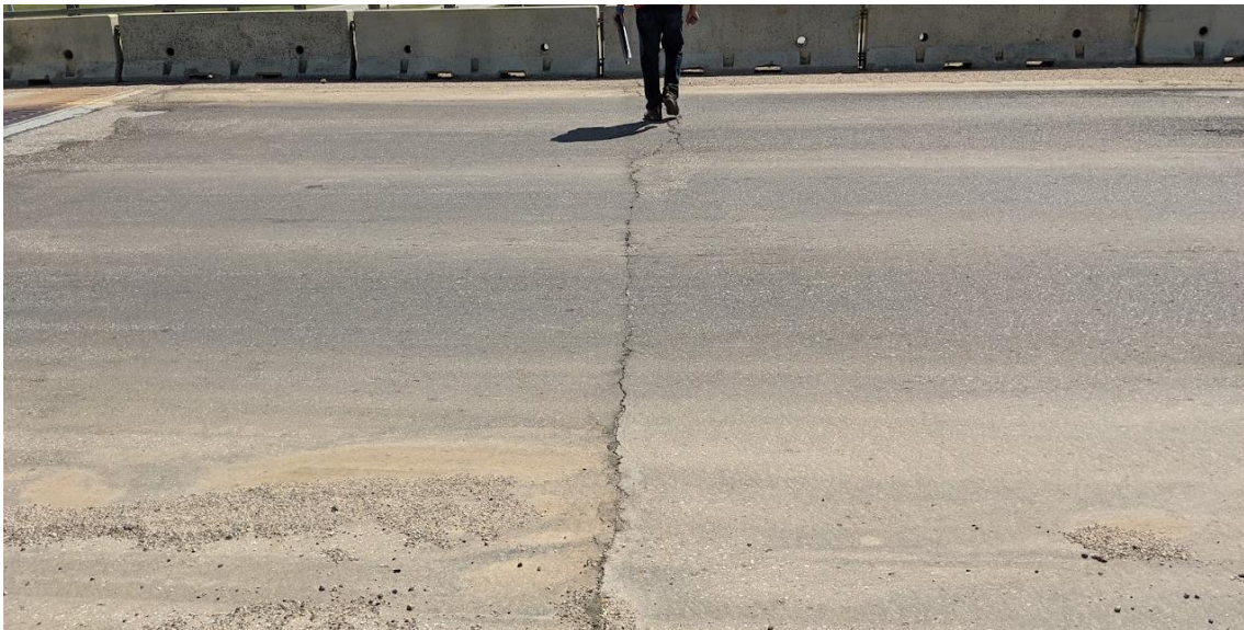
Photo No. 2 – Looking south at the crack across the westbound lanes towards the median. The crack is 5 to 20 mm wide x 5 to 15 mm deep
