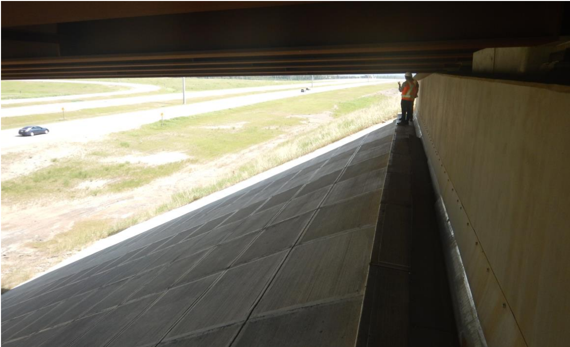
Photo No. 4a – Looking south at the separation of the sheet metal parging on the west abutment
