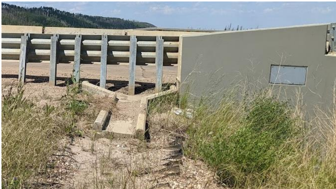
Photo 5 – Looking at the north drain trough. Note the cracking between the drain trough and wingwall.
