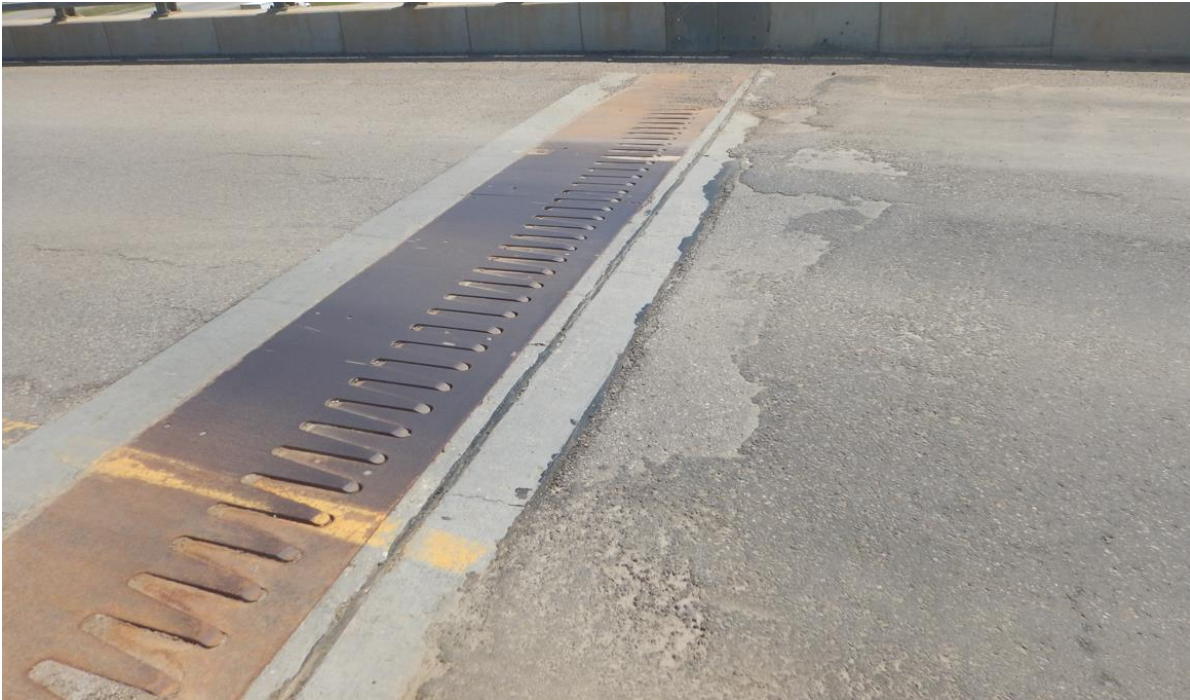
Photo No. 3 – Looking south across the eastbound lanes; there is almost no gap at the joint to accommodate any further movement
