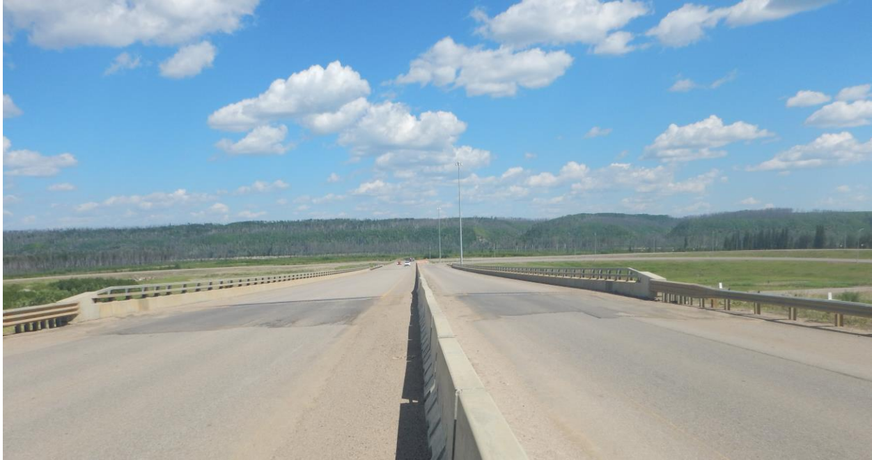
Photo No. 1 – Looking east at the bridge eastbound and westbound lanes. The cracks are across both traffic lane directions and has formed between the approach slab and the pavement, about 6 m west of the west abutment fingerplate; note ACP patch placed in 2020 and the dip to the west of the expansion joint
