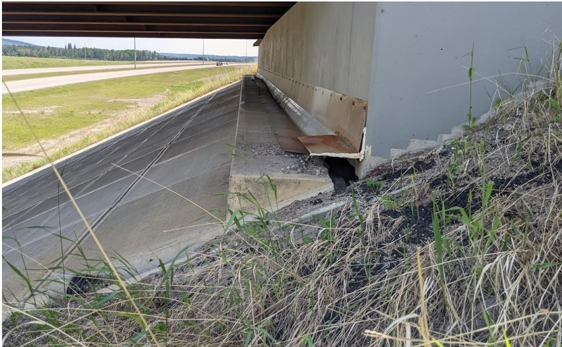
Photo No. 4 – Looking south at a void (50 mm below abutment seat x 1.5 m into the wall) under abutment seat within the northeast corner of the bridge abutment
