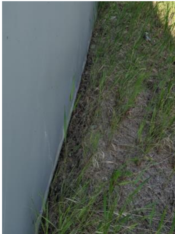
Photo 6 – Looking at the north face of the north wingwall and side slope above the west abutment. Note the fill settlement averages ~100 mm marked by the alkali staining on the paint.
