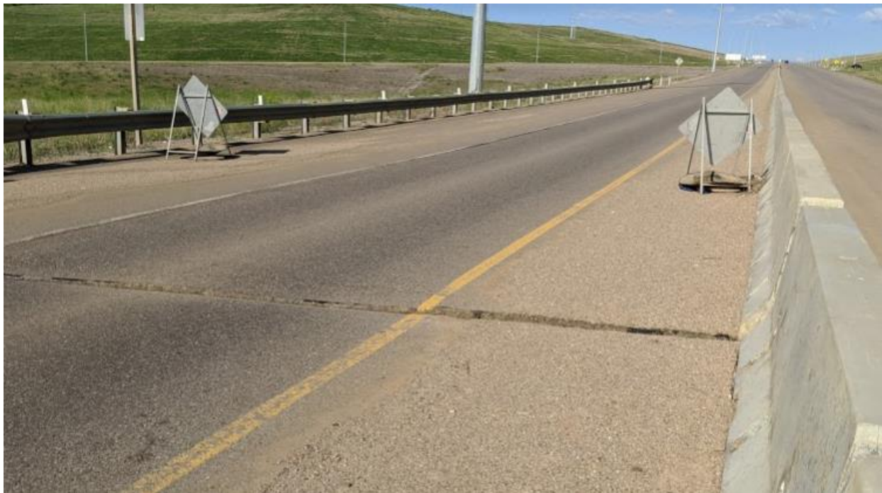
Photo 8 – Looking west at bump on the eastbound lanes. The approach slab settled by 10 to 30mm.
