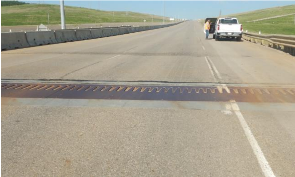
Photo 9 – Looking west at bump on the westbound lanes. The approach slab settled by 10 to 40mm.
