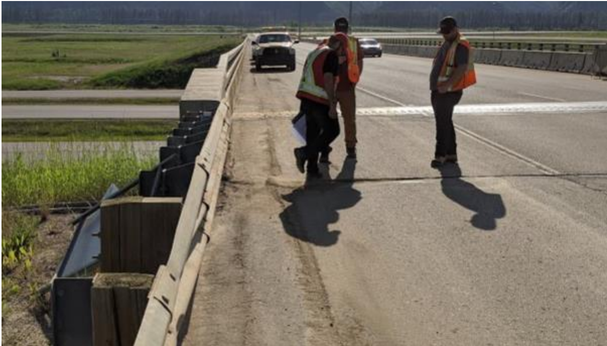
Photo 1 – Looking east at the bridge westbound lanes. The crack is across both traffic lane directions and has formed between the approach slab and the pavement, about 6 m west of the west abutment fingerplate.
