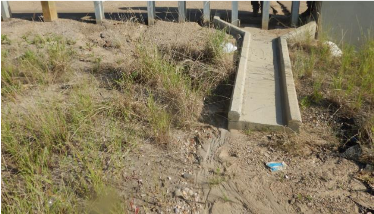
Photo 7 – Looking north at the erosion formed along the south wingwall and side slope at drain trough location
