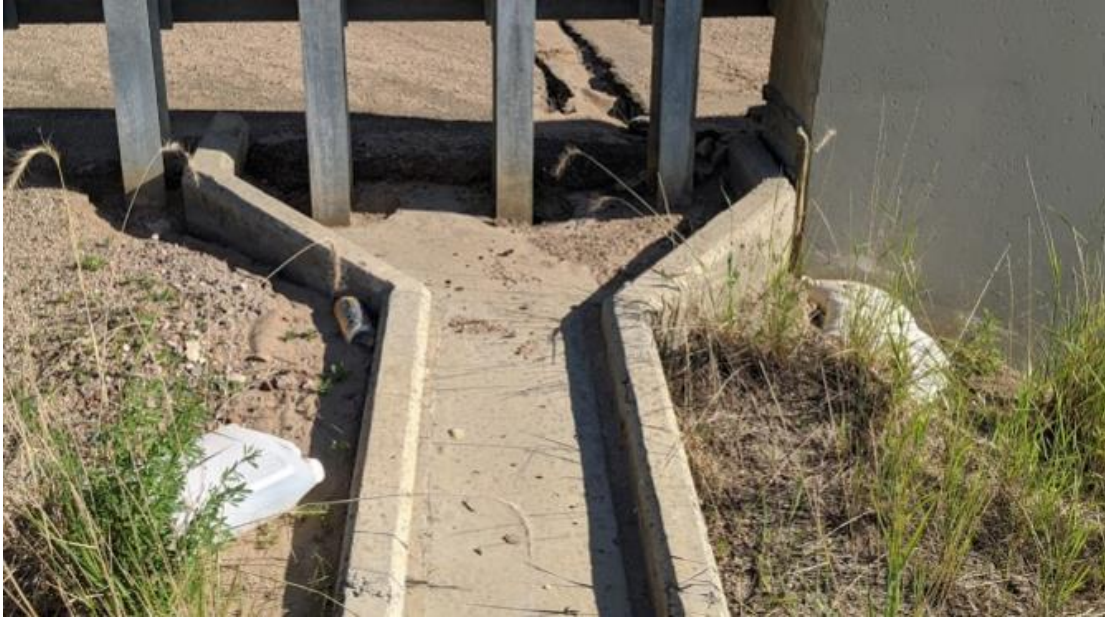
Photo 5 – Looking at the south drain trough. Note the cracking between the drain trough and concrete wingwall.
