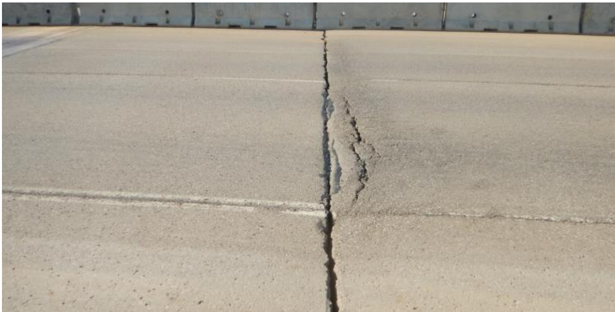
Photo 2 – Looking south at the crack across the westbound lanes towards the median. Note the ~0.3 m wide fatigue cracking on the west (higher) side of the crack. The crack is 40 to 50 mm wide x 40 m deep.
