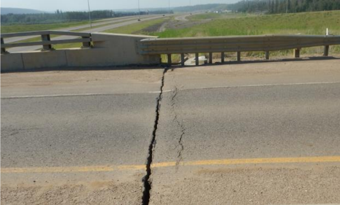
Photo 3 – Looking south across the eastbound lanes. Note the fatigue cracks along the west (higher) side of the main crack.
