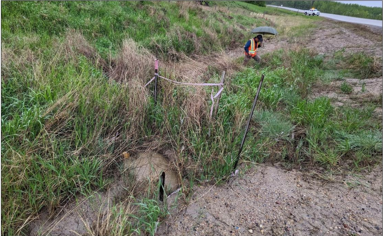
Photo 9. A sink hole (800 mm long x 500 mm wide x 600 mm deep) developed to the west of C3 culvert inlet.
