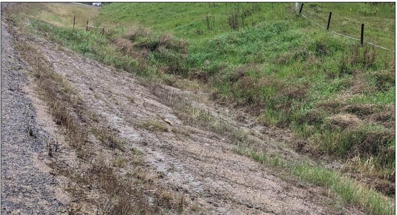
Photo 6. Looking west at the regraded section of the ditch in 2019; side slopes and sections of the ditch bottom are still bare of vegetation; note the presence of erosion rills along the side slope and a deep erosion gully in the ditch.
