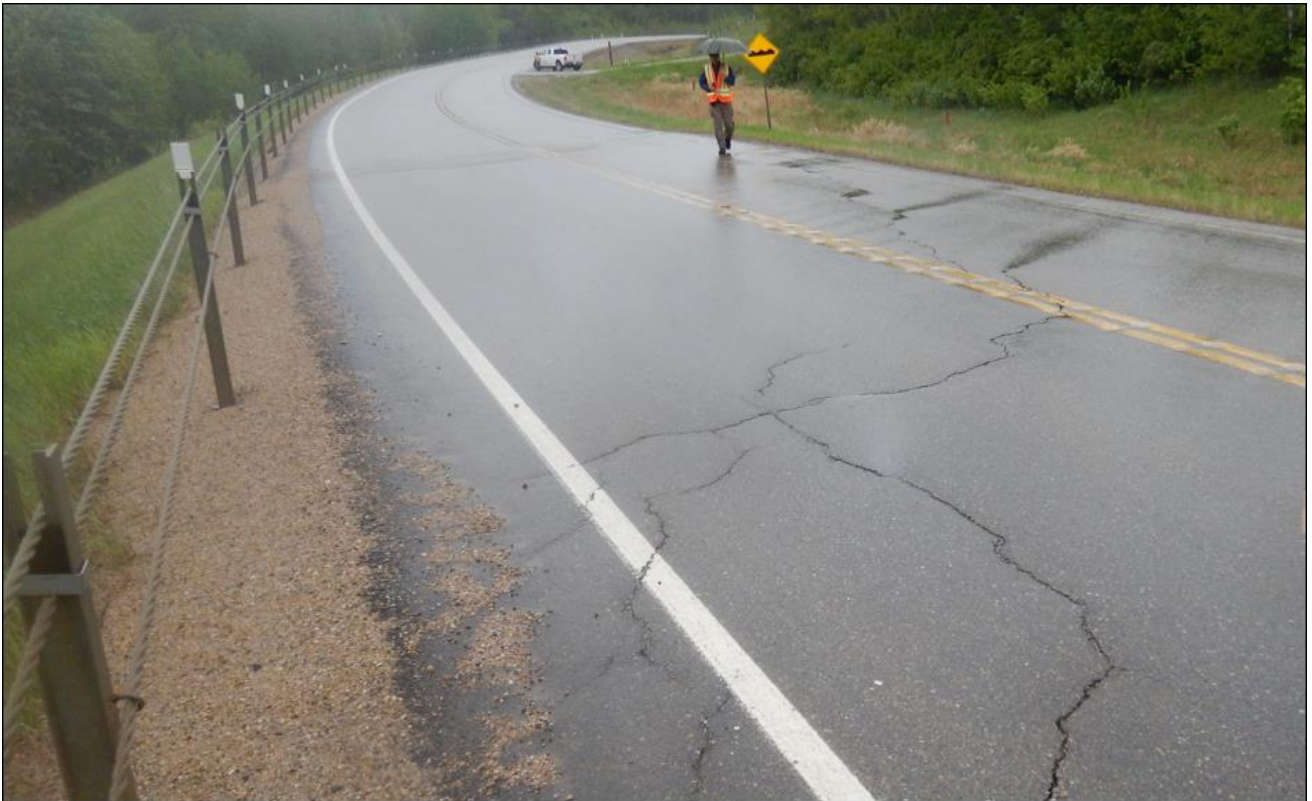
Photo 5 Diagonal cracks located about 15 m east of the landslide western flank
