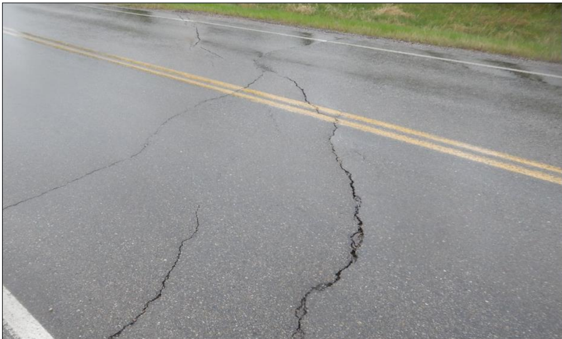
Photo 4. Looking northwest at the eastern flank reflective diagonal cracks
