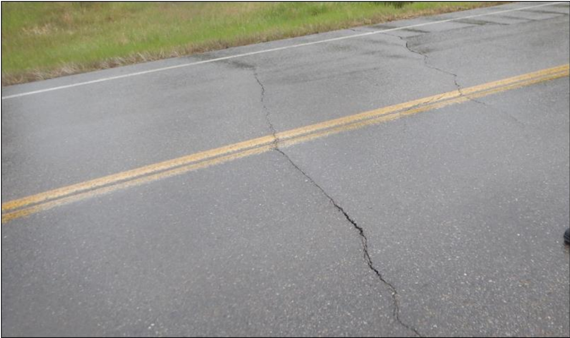
Photo 3. Looking north at a transverse crack (10 - 15 mm wide with no drop).
