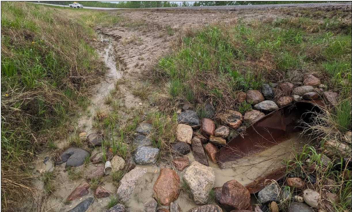
Photo 8. C3 inlet; Water flowing; side slope is bare of vegetation; erosion developing upstream of the inlet within the ditch.
