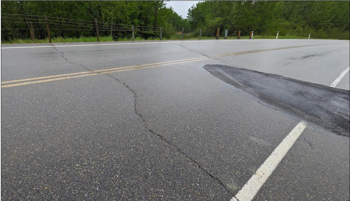
Photo 7. Looking southwest at the sinkhole previously developed within the northern edge of pavement of the highway above the original 600 mm diameter culvert (C3); Original pipe was grouted and a new 760 mm diameter SWSP was auger bored in 2021; cold mix patch placed on the highway surface (2022), larger ACP patch was noted in 2024.
