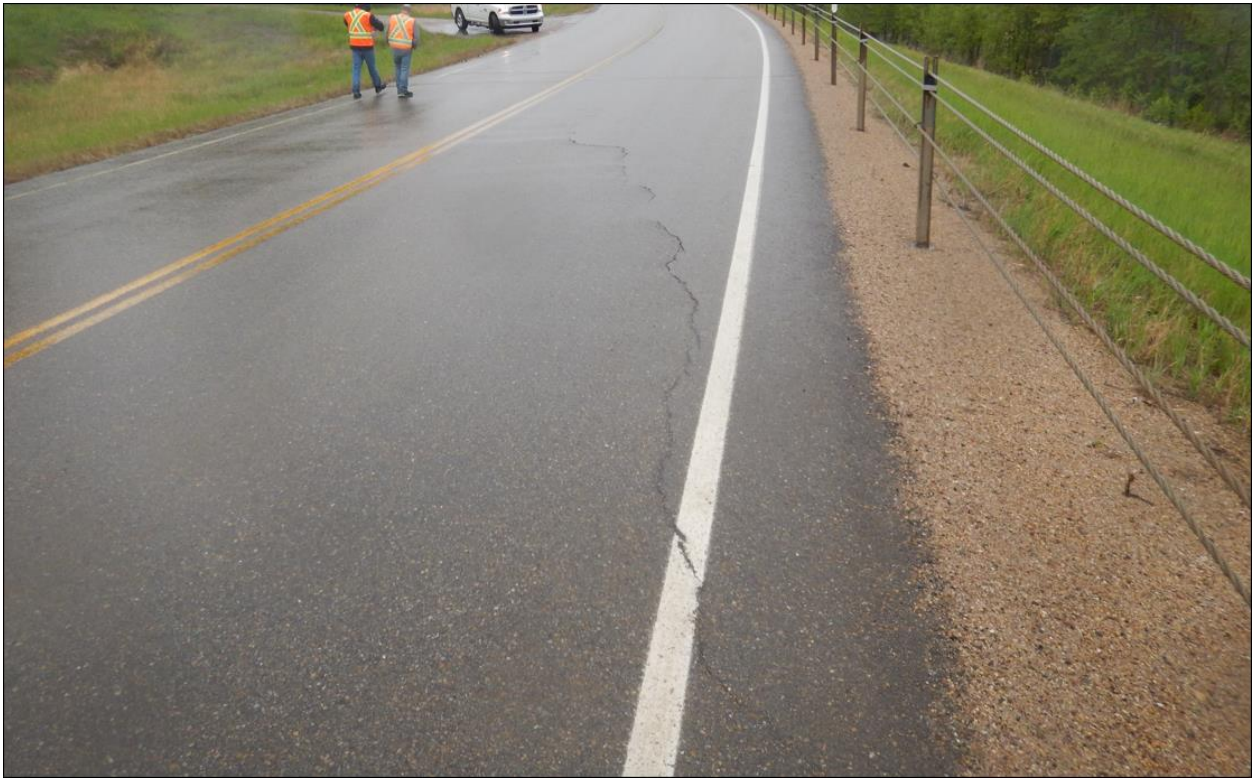
Photo 1. Looking at (15-20 mm wide, 5 mm drop) diagonal crack on the highway surface from the western limit of the site.
