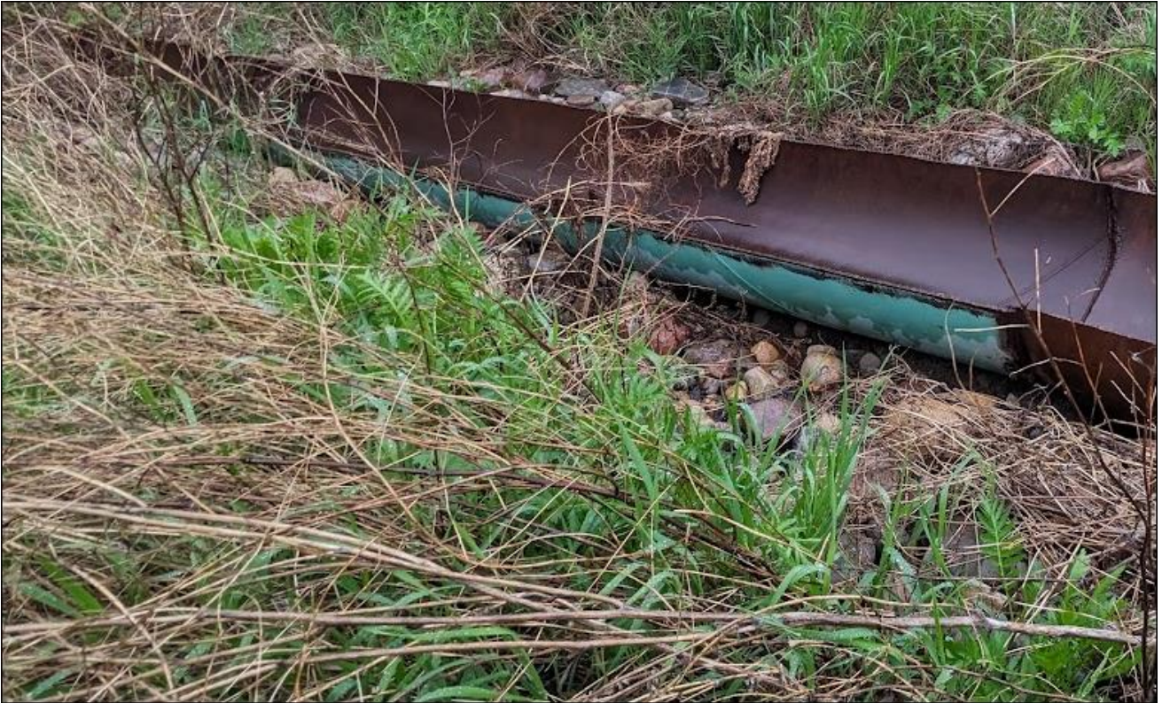
Photo 11. Outlet of culvert C3, installed in 2021. There is a void below the half pipe extension piece.
