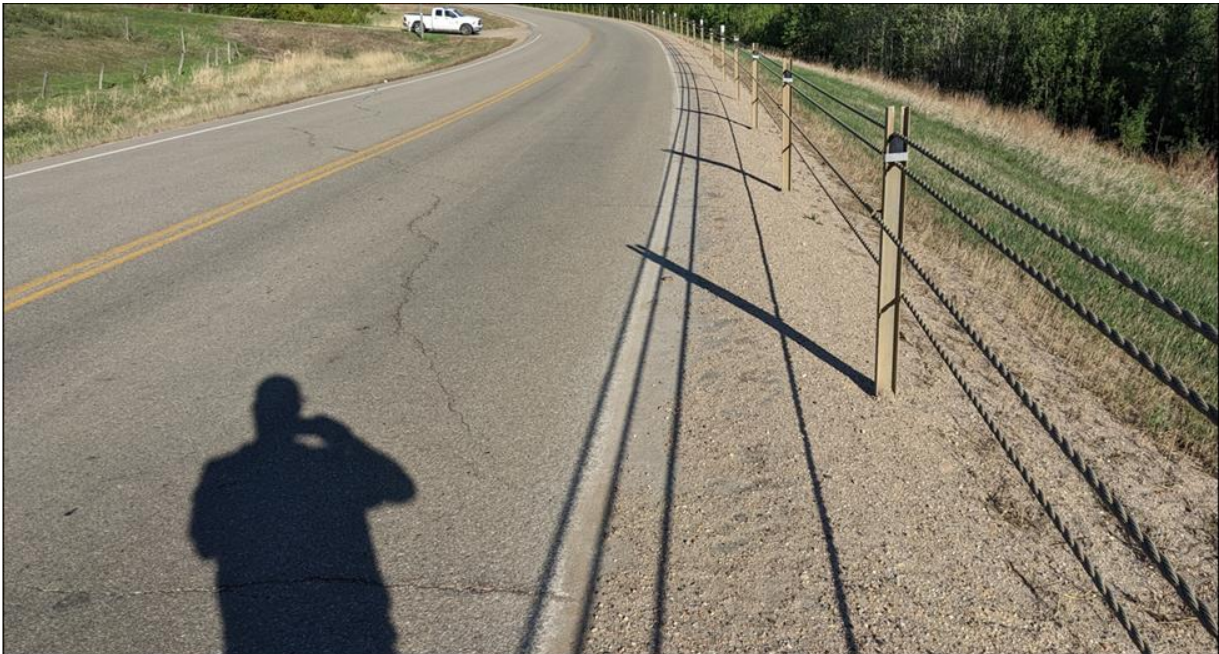
Photo 1. Looking at reflective diagonal cracks on the highway surface from the western limit of the site.
