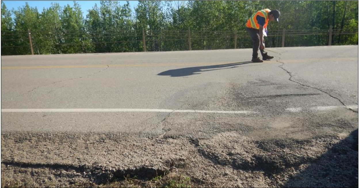
Photo 7. Looking southwest at the sinkhole previously developed within the northern edge of pavement of the highway above the original 600 mm diameter culvert (C3); Original pipe was grouted and a new 760 mm diameter SWSP was auger bored in 2021; cold mix patch placed on the highway surface, but cracks are still visible around the patched area; there is a 50 mm dip within the previously patched area.
