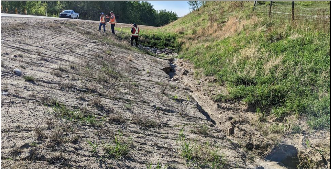
Photo 6. Looking west at the regraded section of the ditch in 2019; side slopes and sections of the ditch bottom are bare of vegetation; note the presence of erosion rills along the side slope and a deep erosion gully in the ditch.
