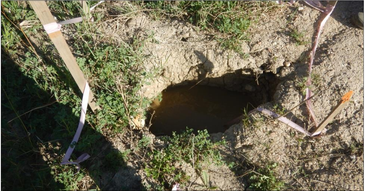
Photo 9. A sink hole (800 mm long x 500 mm wide x 600 mm deep) developed to the west of C3 culvert inlet.
