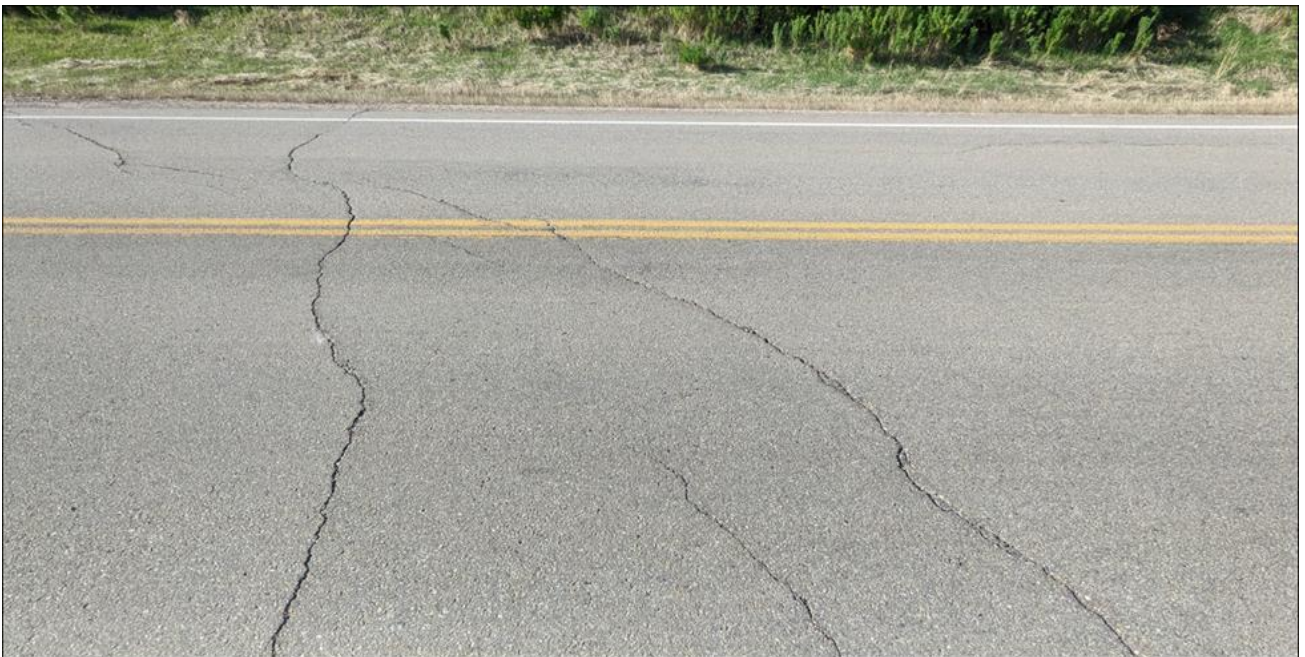
Photo 4. Looking northwest at the eastern flank reflective diagonal cracks (20 -25 mm wide with no drop).
