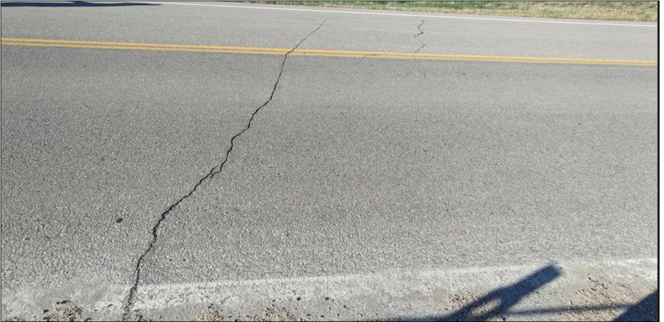
Photo 3. Looking north at a transverse crack (10 to 15 mm wide with no drop)
