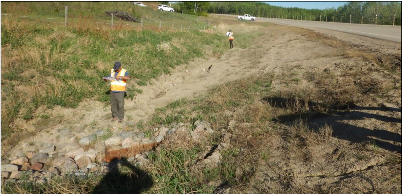
Photo 8. C3 inlet; side slope is bare of vegetation; open crack around culvert inlet and erosion developing upstream of the inlet within the ditch.
