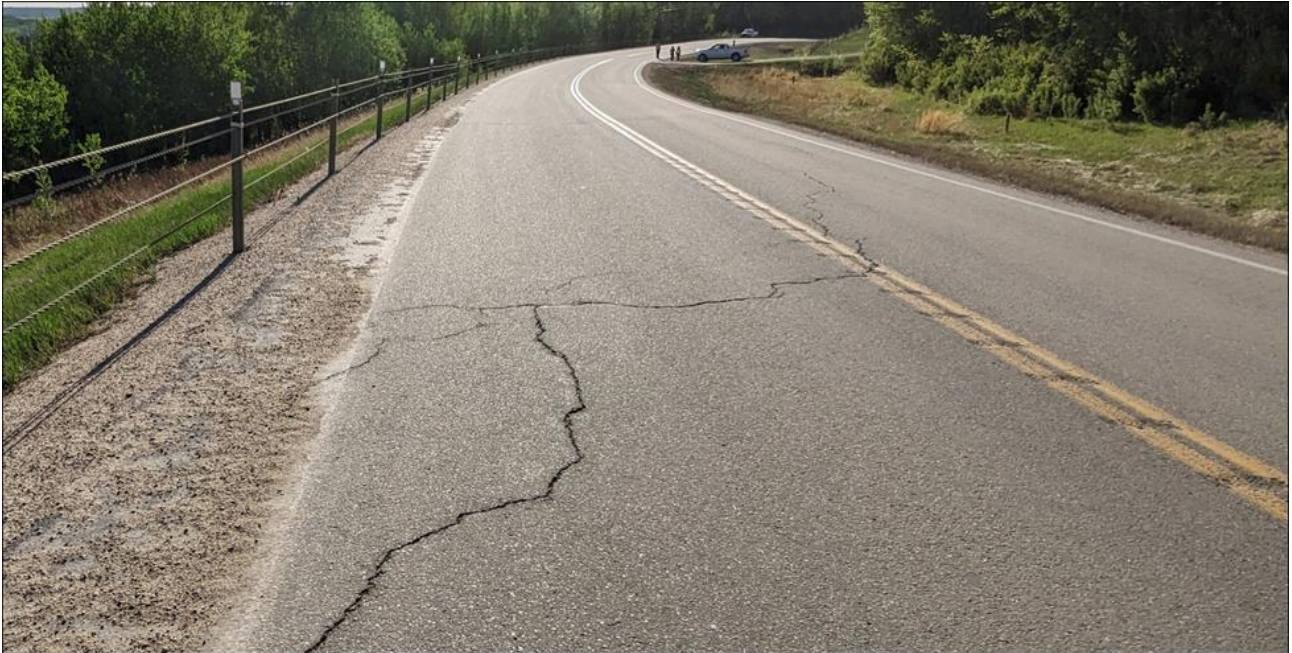
Photo 5 Diagonal cracks located about 15 m east of the landslide western flank; 20mm – 30 mm wide with no drop.
