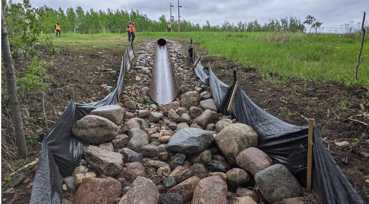
Photo No. 9 – Looking north at the outlet of culvert C3, installed in 2021. There is a void below the half pipe extension piece.
