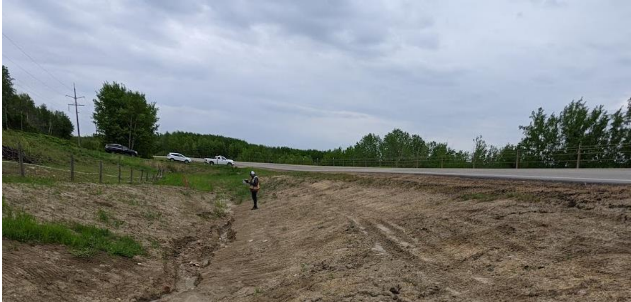
Photo No. 5 – Looking east at ditch regraded in 2019 by WSP; the north ditch has been regraded from culvert C1 outlet to culvert C3 inlet; culvert C2 appears to have been abandoned; side slopes and sections of the ditch bottom are bare of vegetation; erosion developed within the ditch
