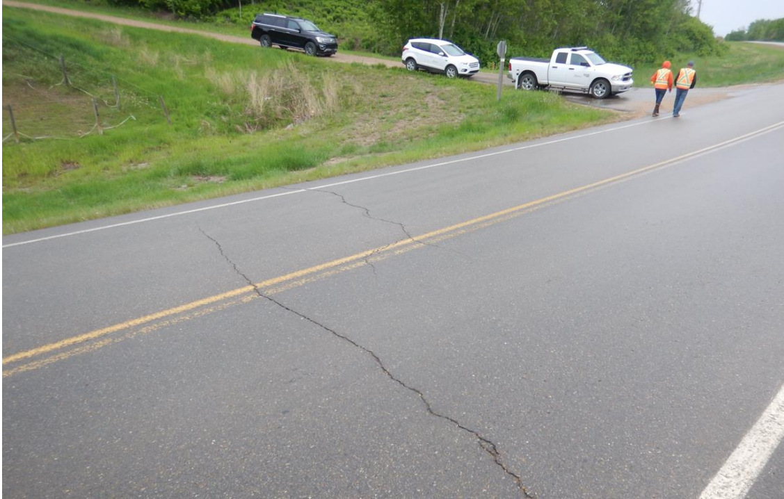
Photo No. 3 – Looking north at a transverse crack (10 to 15 mm wide with no drop)
