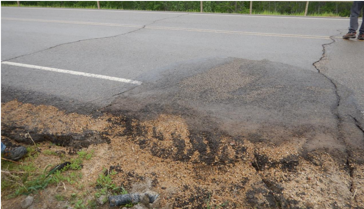
Photo No. 6 – Sinkhole previously developed within the northern edge of pavement of the highway above the original 600 mm diameter culvert (C3) ; Original pipe was grouted and a new 760 mm diameter SWSP was auger bored in 2021; cold mix patch placed on the highway surface but cracks are still visible around the patched area
