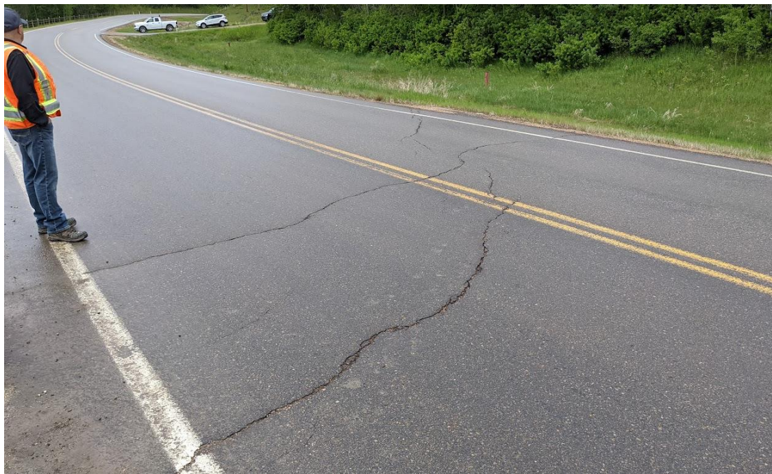
Photo No. 4 – Looking northwest at the eastern flank reflective diagonal cracks (20 – 40 mm wide with no drop)
