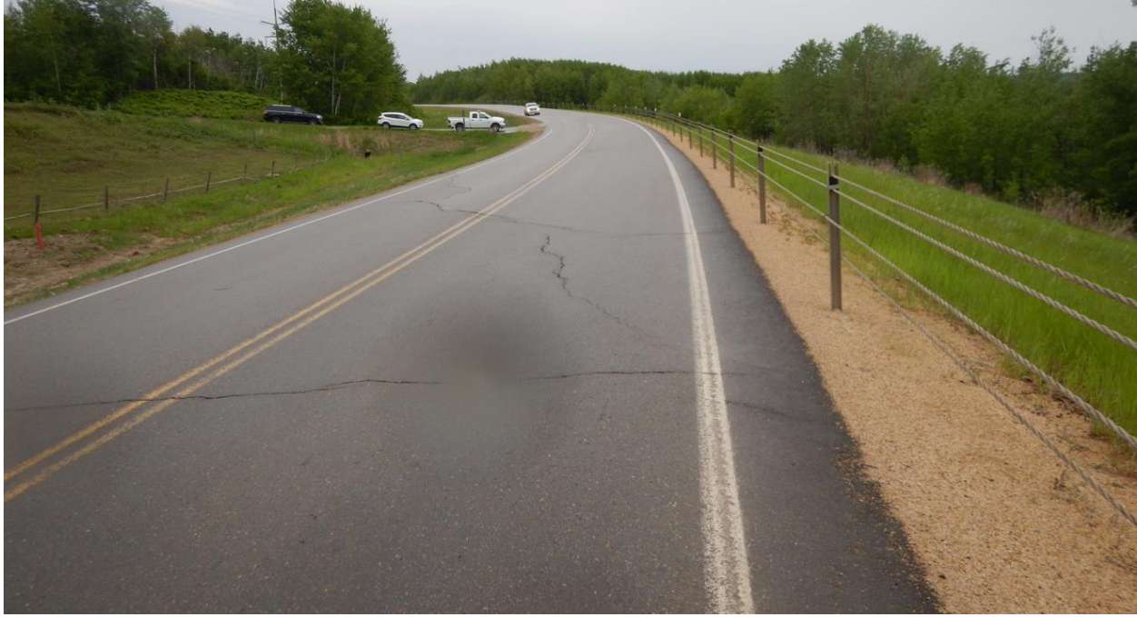
Photo No. 1 – Looking at reflective diagonal cracks on the highway surface from the western limit of the site
