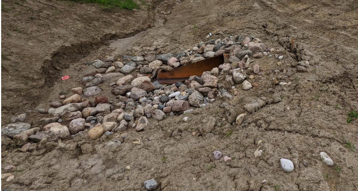
Photo No. 7 – Looking south at new culvert C3 inlet; note bare vegetation, crack around culvert inlet and erosion developing upstream of the inlet within the ditch
