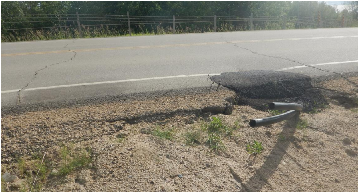
Photo No. 6 – Sinkhole developed above culvert C3 near the north edge of pavement appears to have been fixed in 2020 by grouting the void and placing cold mix patch at the surface; there is a 50 mm dip within the patched surface of the original sinkhole and cracks are developing around the patched area
