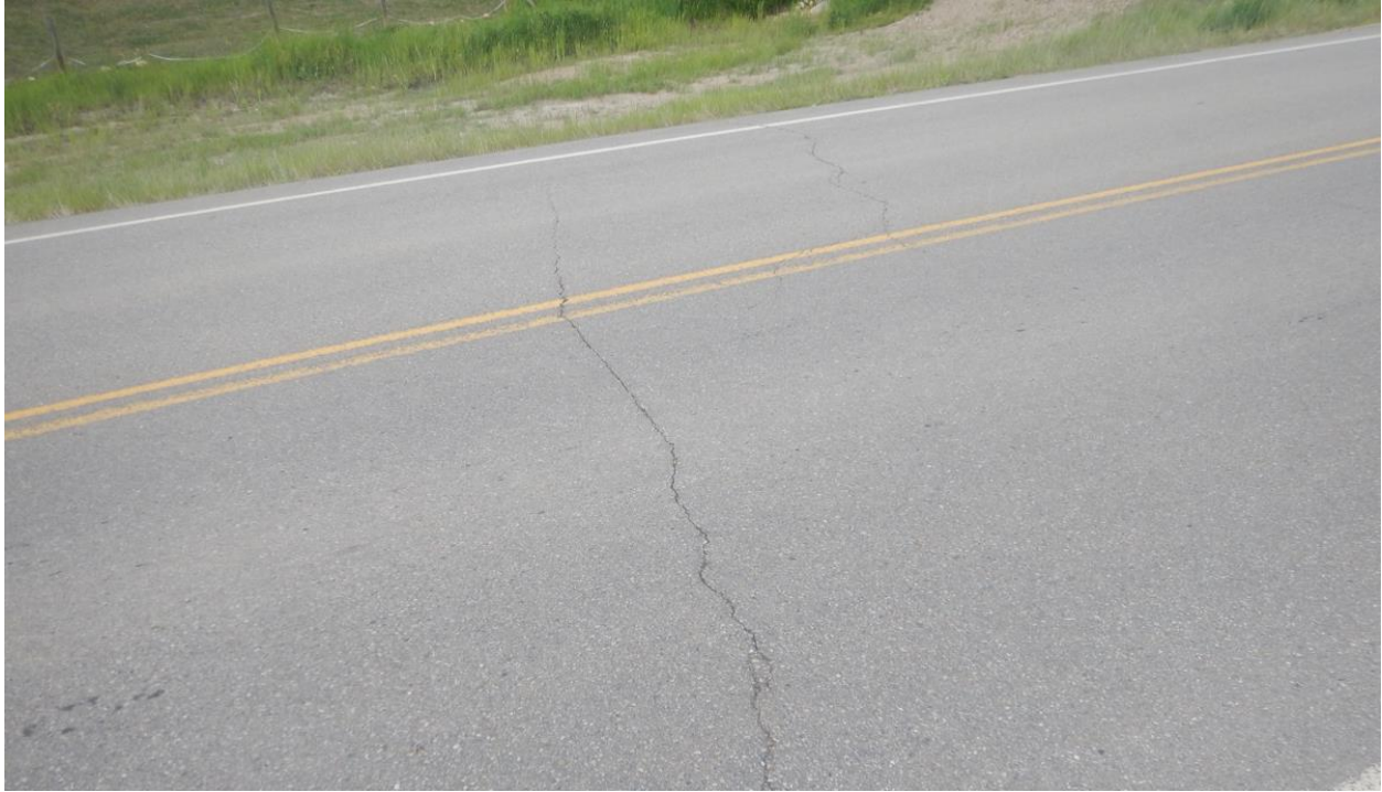
Photo No. 3 – Looking north at a transverse crack (5 to 10 mm wide with no drop)
