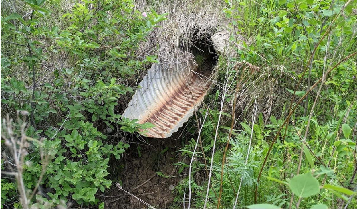
Photo No. 9 – Looking west at culvert C3 outlet; note 2.2 m deep scour at the culvert outlet
