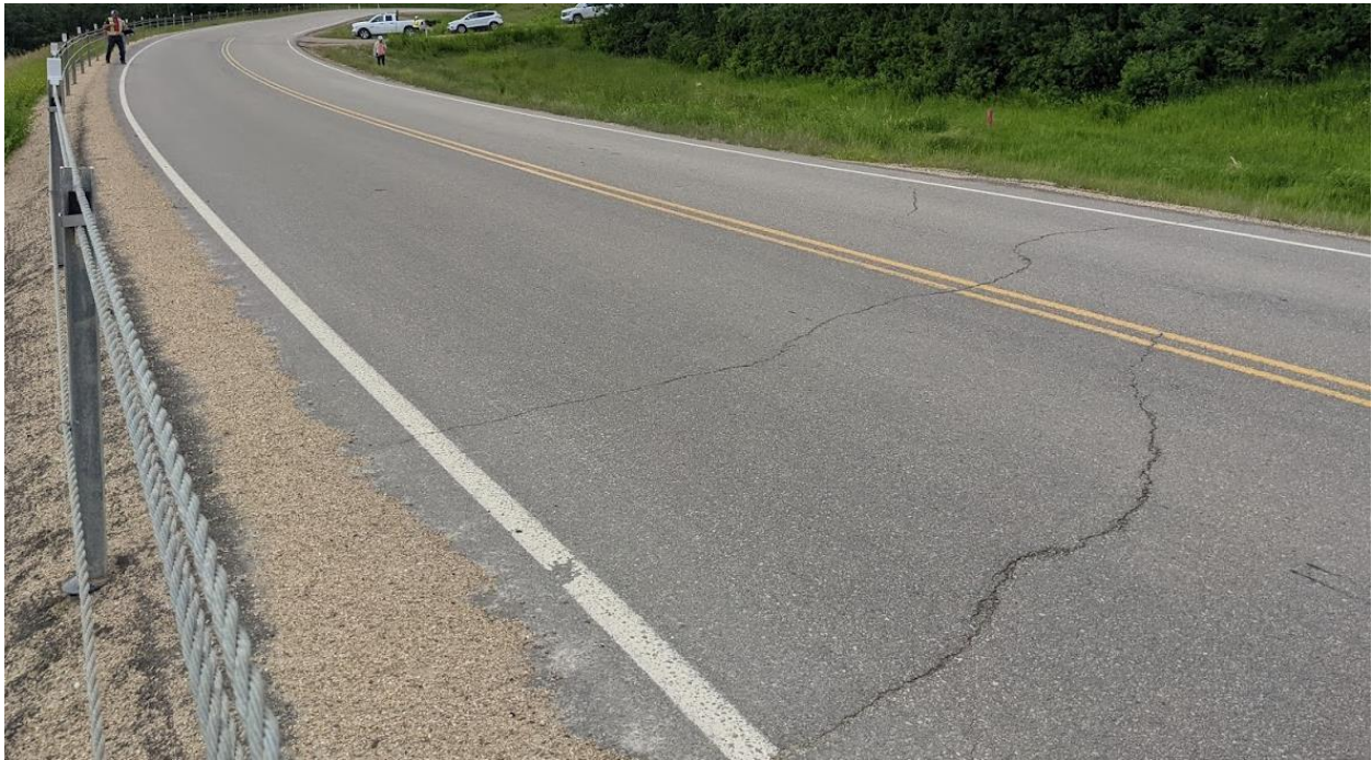
Photo No. 4 – Looking northwest at the eastern flank reflective diagonal cracks (5 – 20 mm wide with no drop)
