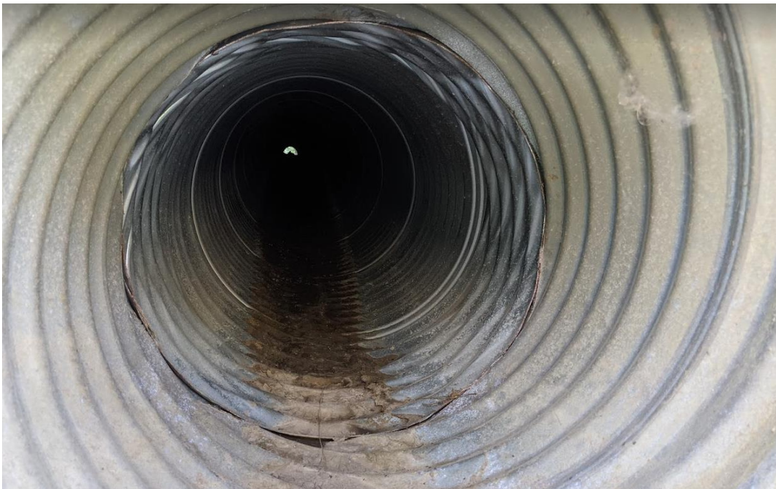
Photo No.8 – Looking inside culvert C3 inlet; note culvert separation and rusting at the base
