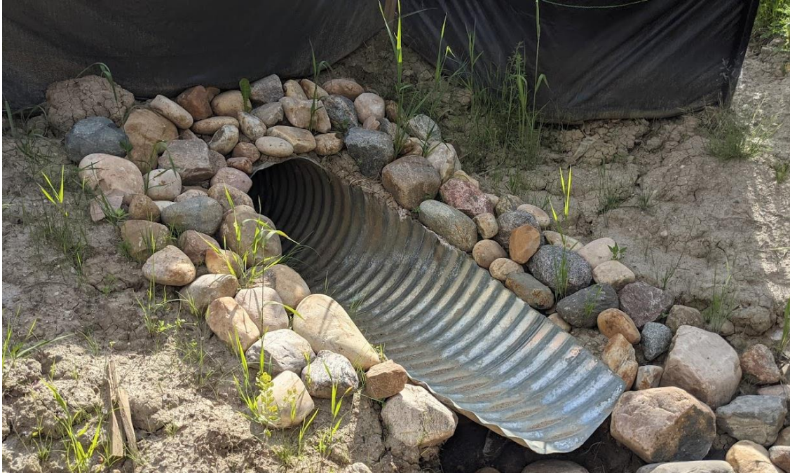
Photo No. 7 – Looking south at culvert C3 inlet; note that the inlet invert is hanging above ground and the presence of a scattered riprap
