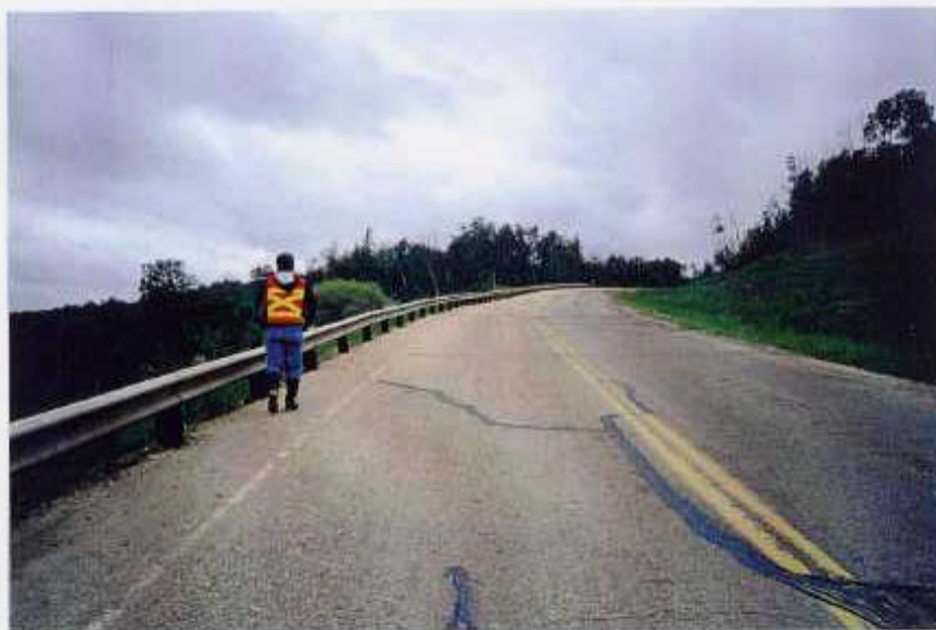
PHOTO NC14-2 LOOKING NORTHWEST (UPSLOPE) AT DIP IN SHOULDER.
