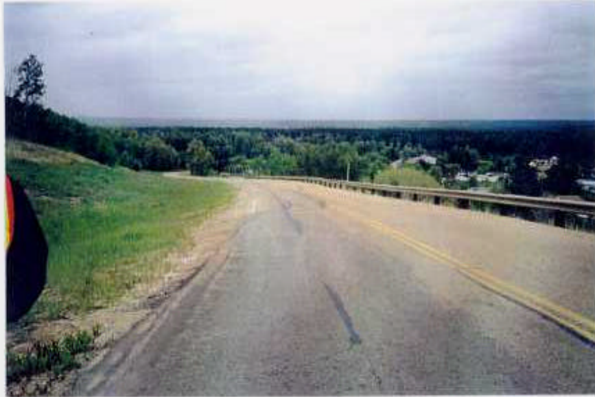
PHOTO NC14-3 LOOKING SOUTHEAST AT PATCH IN ROADWAY (UPPER SLOPE).
